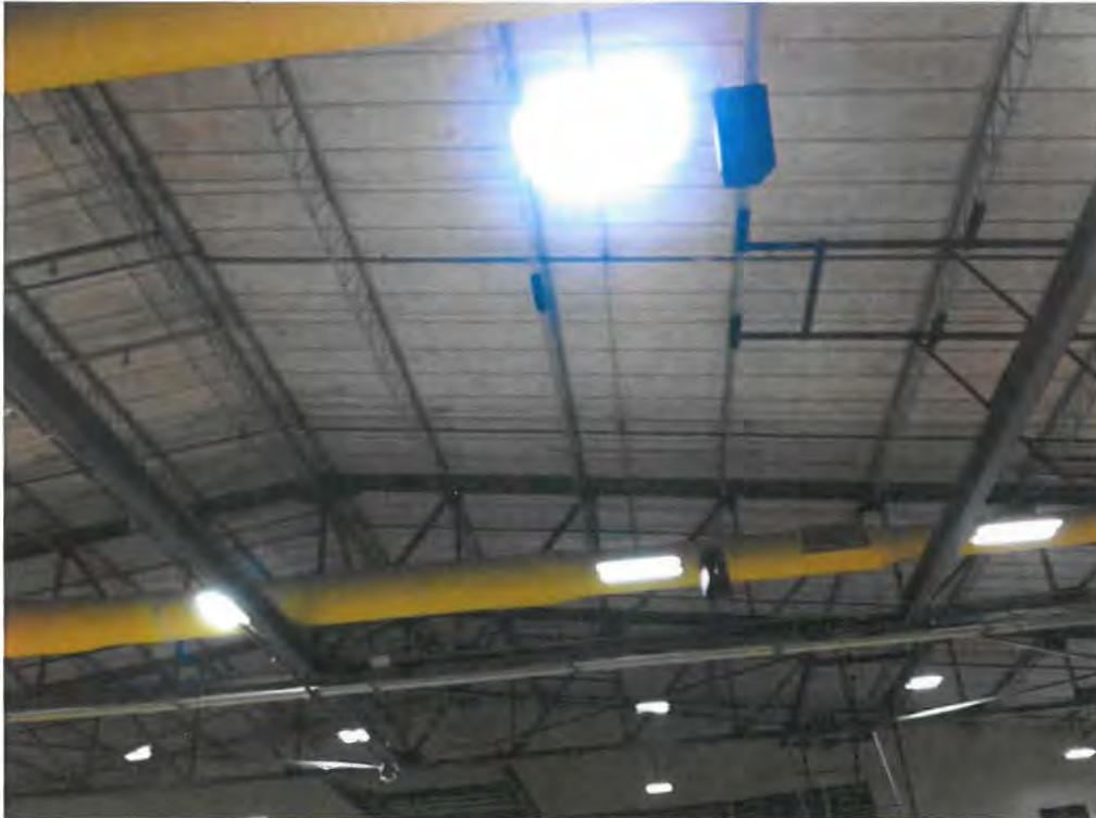
This picture shows a gymnasium in Scott County which was converted from metal halide fixtures to LED fixtures.
