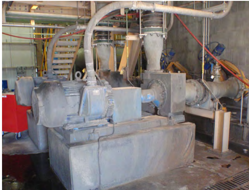
Figure 26. Bleed Pumps at Brown Station
