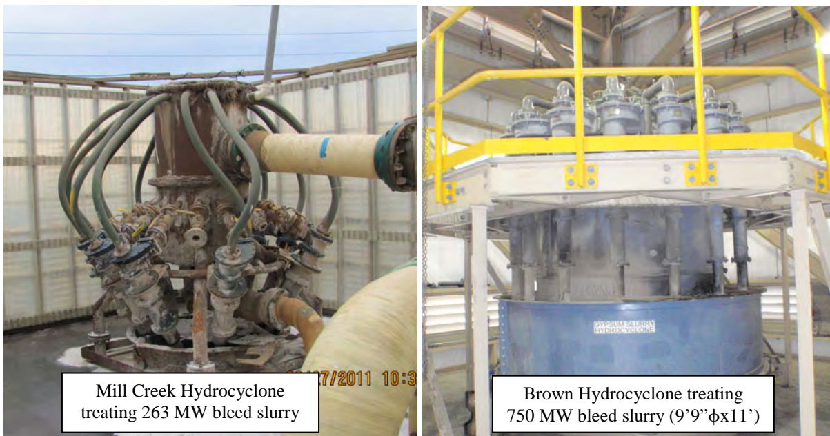
Figure 10. Photos of Hydrocyclone Assemblies at Mill Creek and Brown
