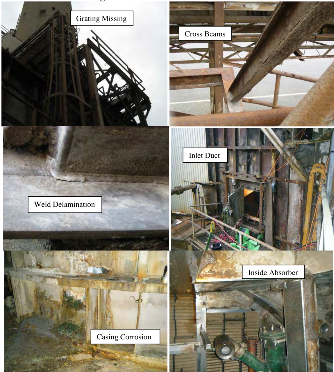
Figure 4. Areas of Corrosion on Unit 4
