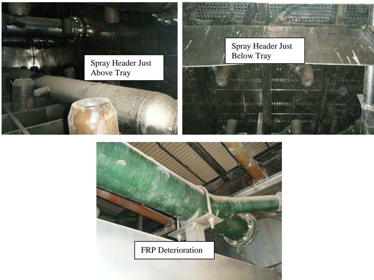
Figure 6. Existing Absorber Spray Headers
