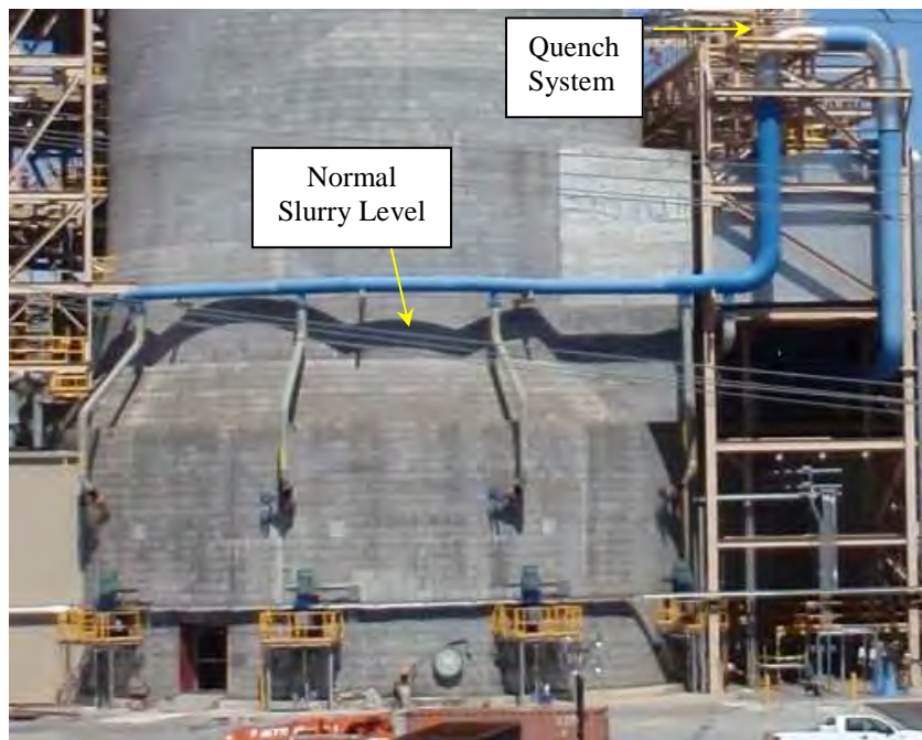
Figure 23: Oxidation Air Distribution Ring and Agitators
