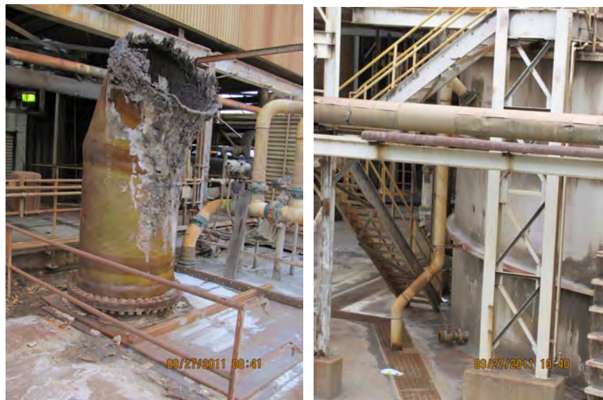
Figure 1. Absorber Reaction Tank Vent and Overflow
