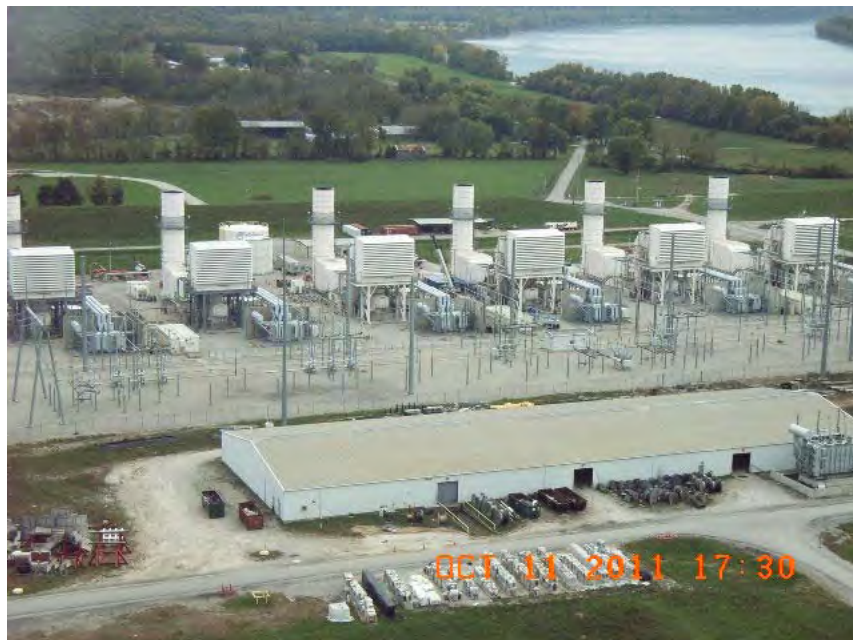
6 CT Units at Trimble County Generating Station
