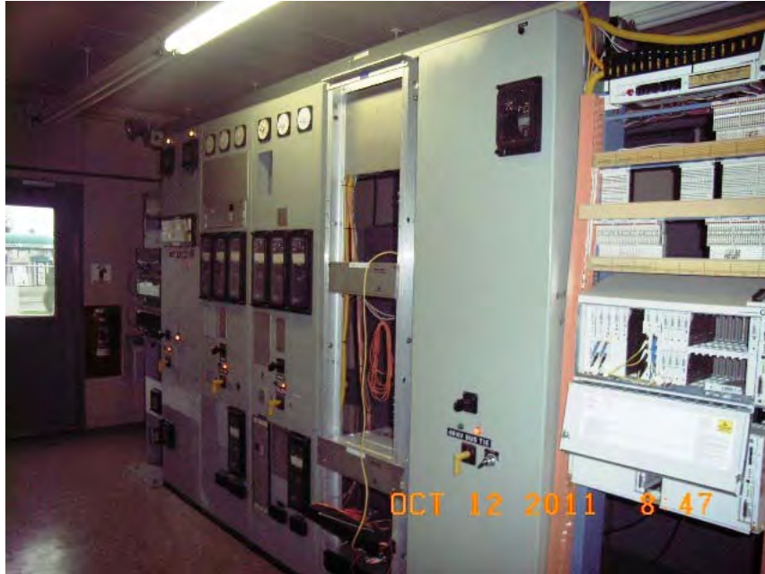
Controls at Frey's Hill Substation
