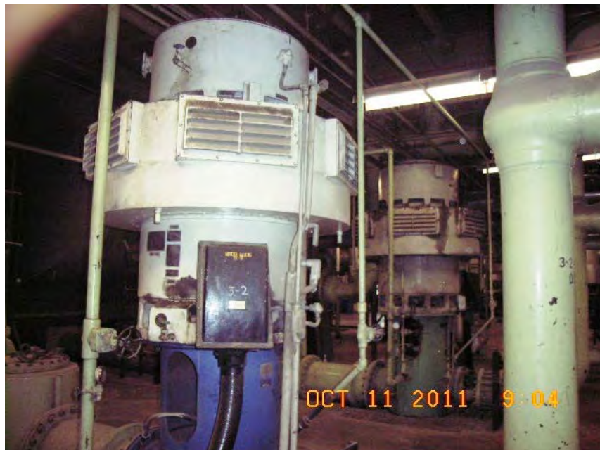
Unit 5 Condensate Pumps at Brown Generating Station
