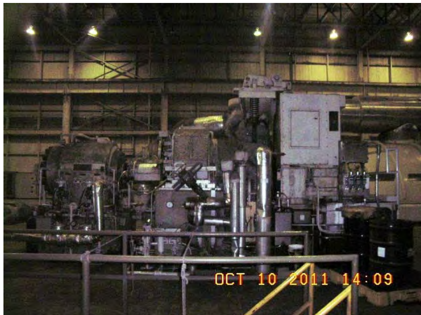
Boiler Feed Pump at Mill Creek Generating Station
