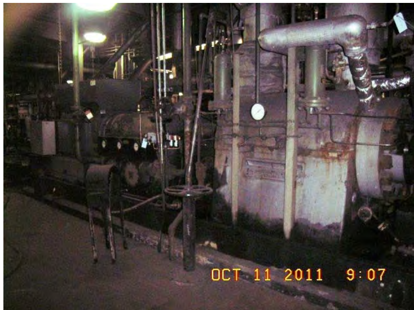
Unit 2 Boiler Feed Pumps at Brown Generating Station
