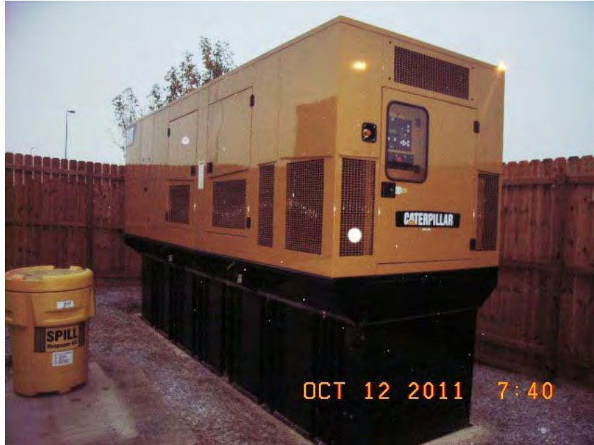
Emergency Generator at East Service Center
