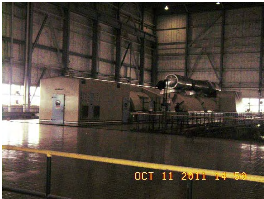
Unit 2 Turbine at Ghent Generating Station
