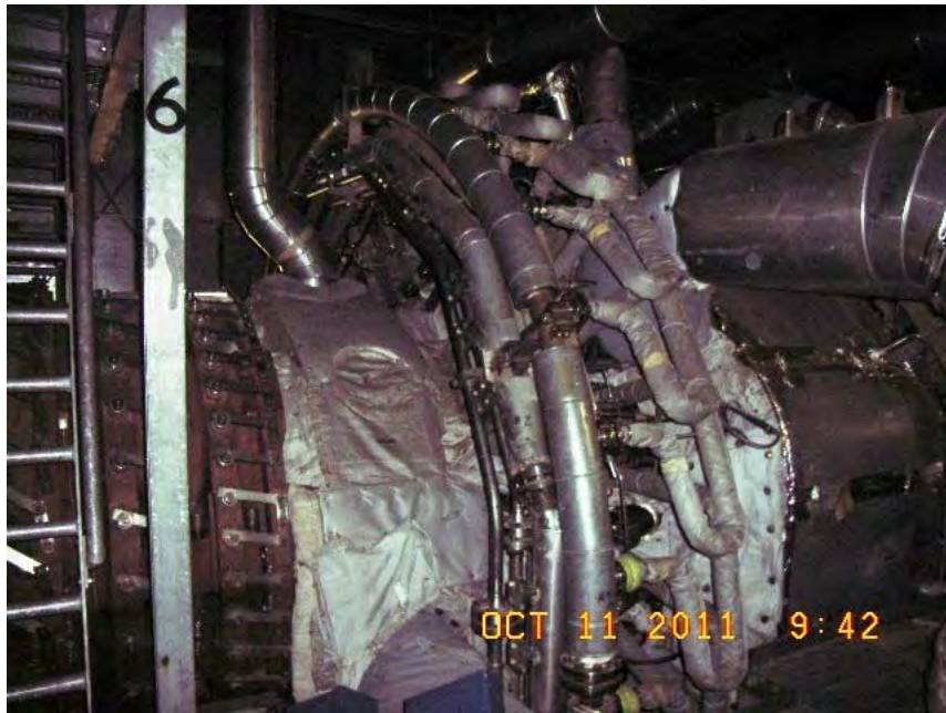
Unit 6 Turbine at Brown CT Generating Station
