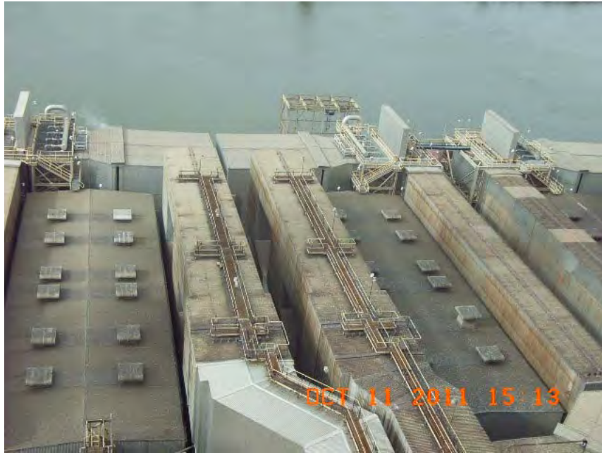
Unit 4 Precipitator and SCR at Ghent Generating Station
