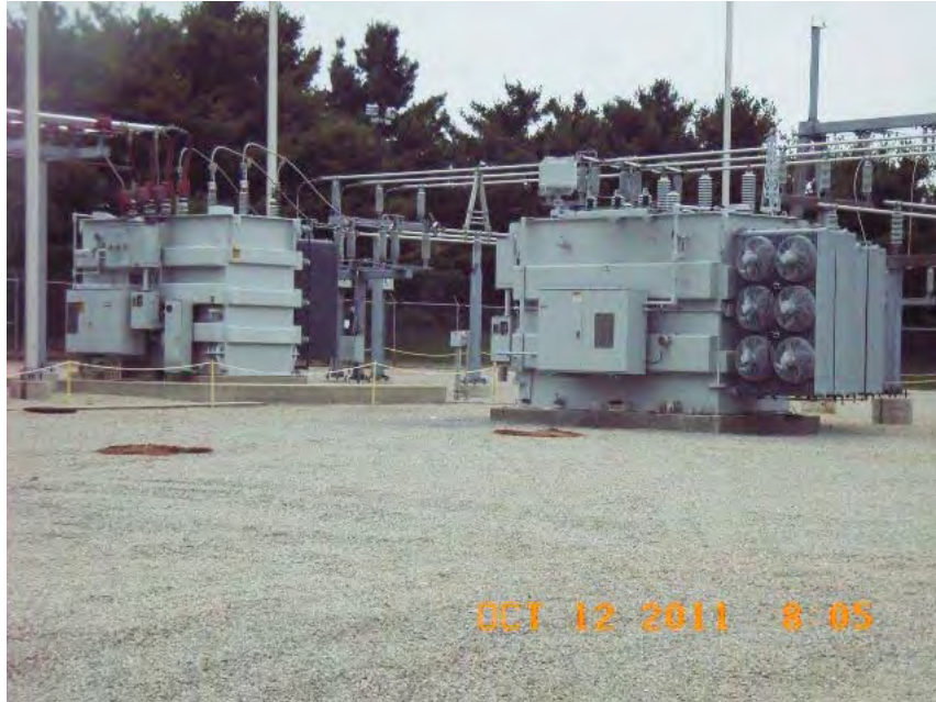
Transformers at Worthington Substation
