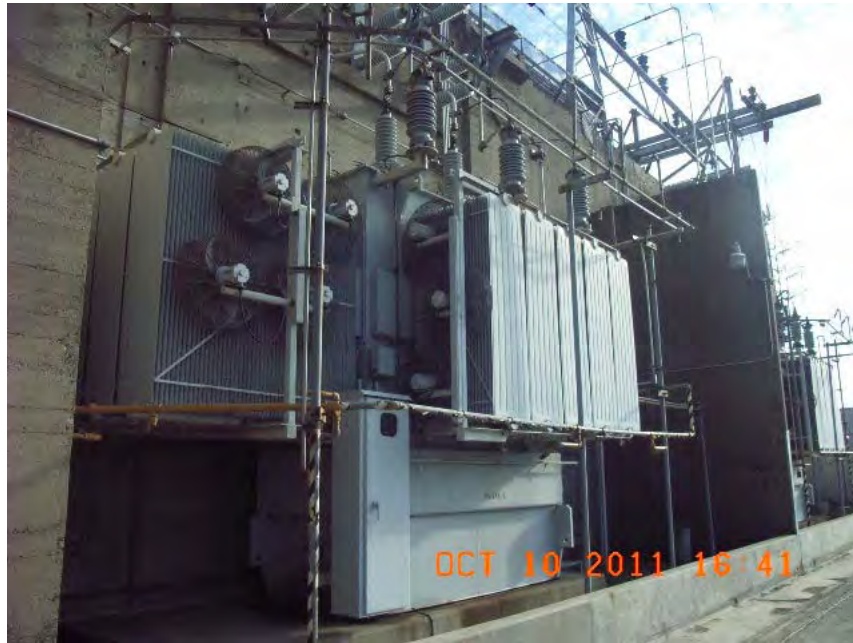
Transformer at Oho Falls Hydro Plant
