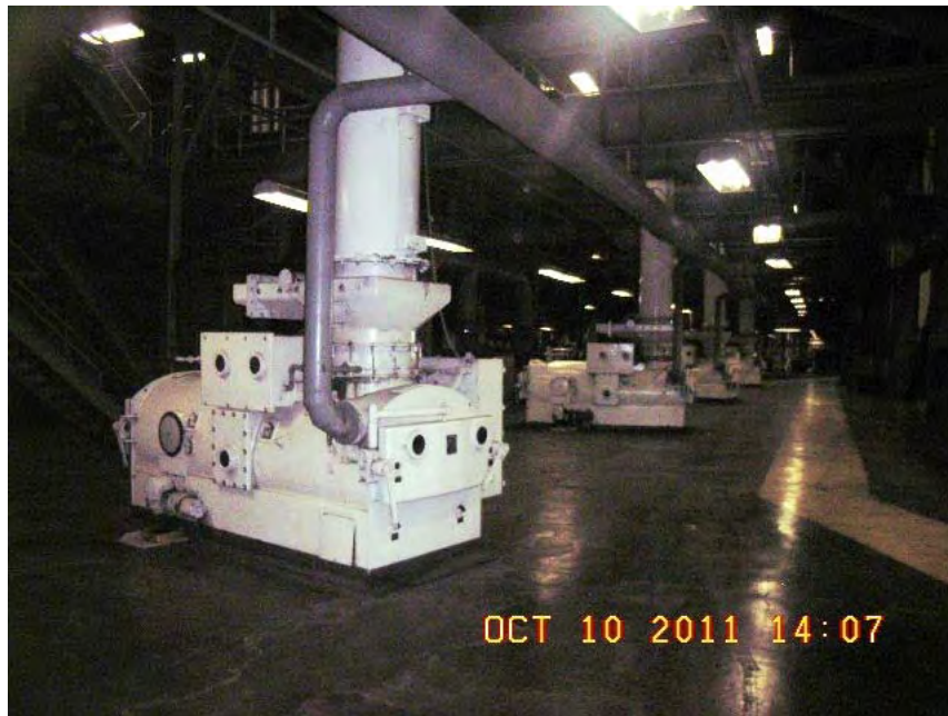
Unit 3 Coal Feeders at Mill Creek Generating Station
