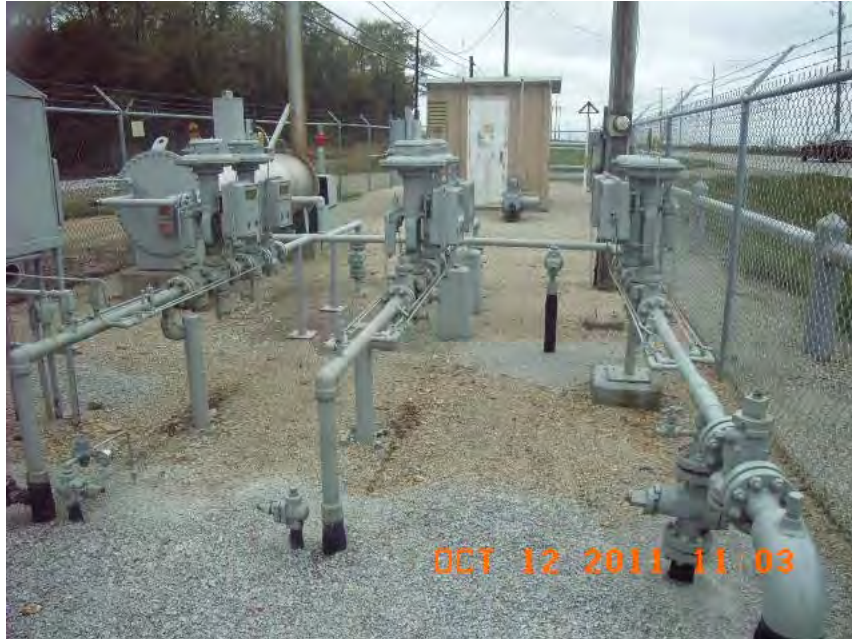
Regulator Runs at LaGrange City Gate Station
