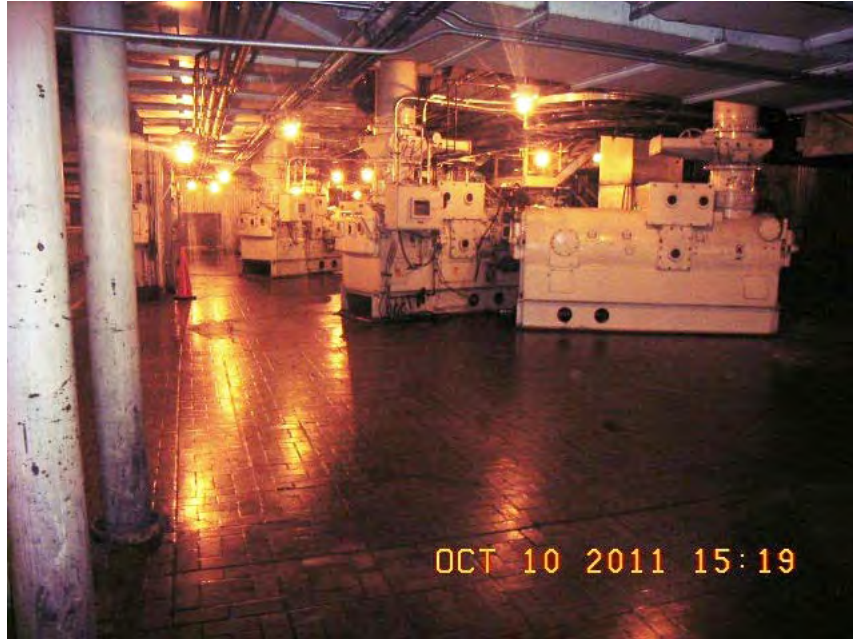
Coal Feeders for Unit 5 at Cane Run Generating Station
