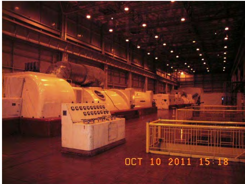
Turbines 4 and 5 at Cane Run Generating Station
