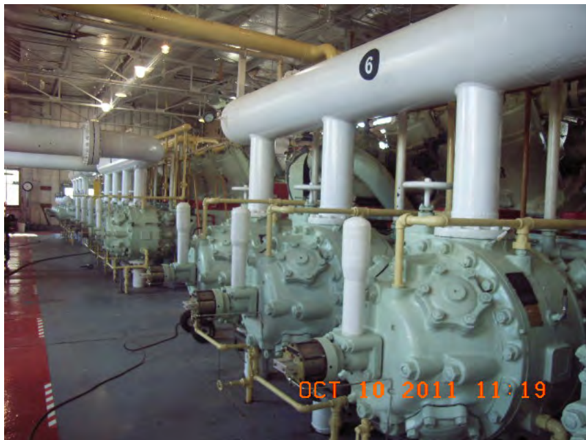
Compressors 6, 7 & 8 at Muldraugh Compressor Station
