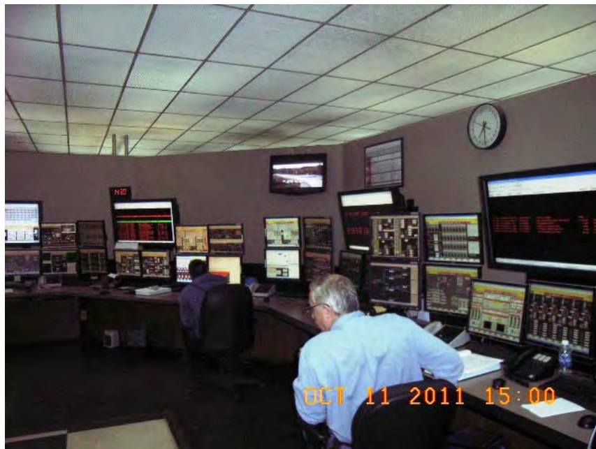
Unit 1 & 2 Controls at Ghent Generating Station
