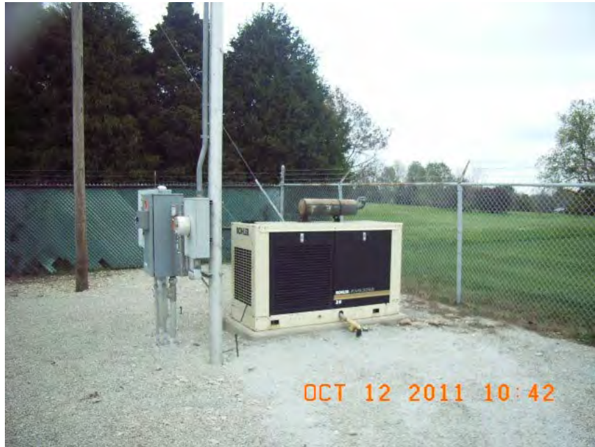
Emergency Generator at Elder Park City Gate Station
