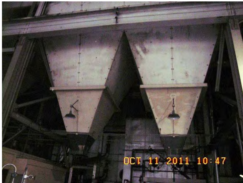
Boiler at Tyrone Generating Station
