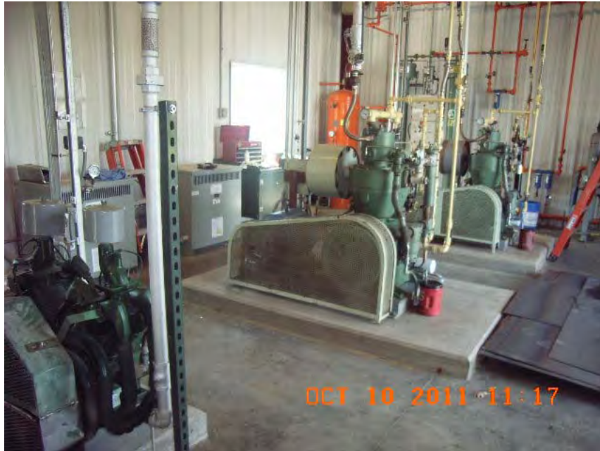
3 New Air Compressors at Muldraugh Compressor Station
