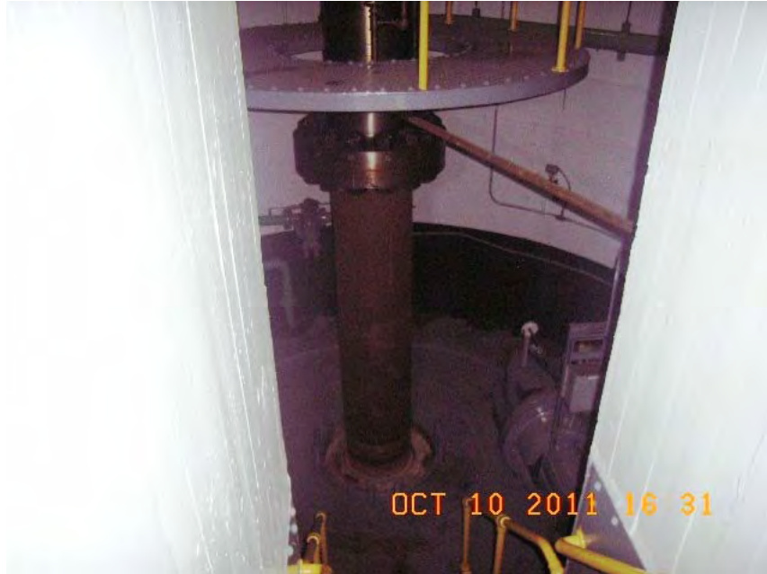
Turbine Shaft and Wicket Gates Unit 6 at Ohio Falls Hydro Plant
