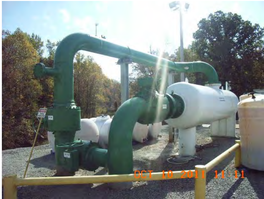
Filter Separator at Muldraugh Compressor Station
