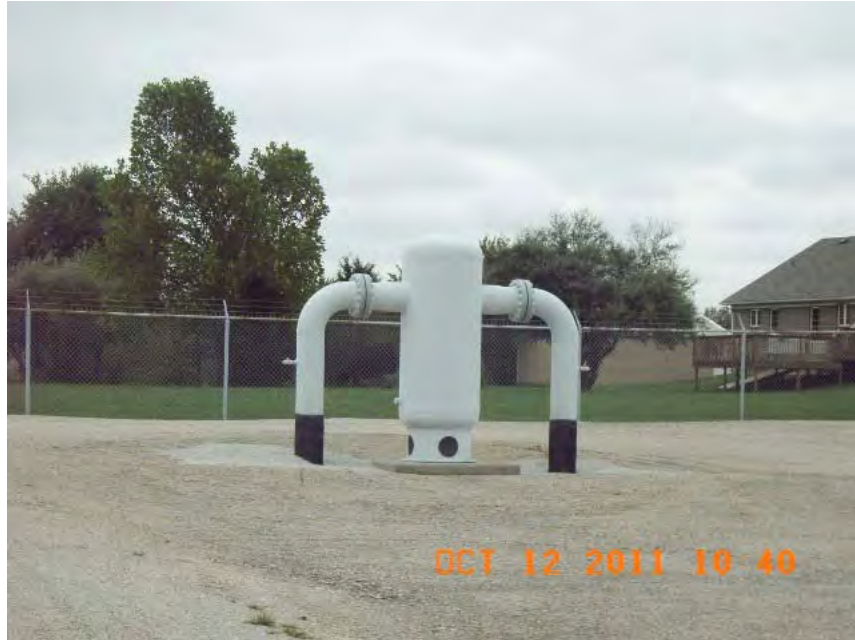
Separator at Elder Park City Gate Station
