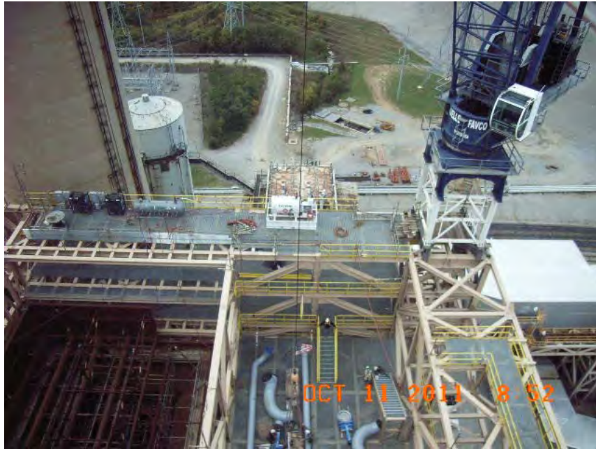
Unit 3 SCR AT Brown Generating Station
