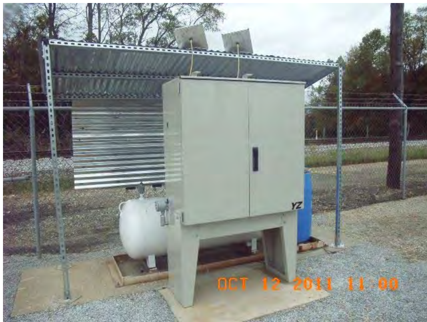
Odorant Equipment at LaGrange City Gate Station
