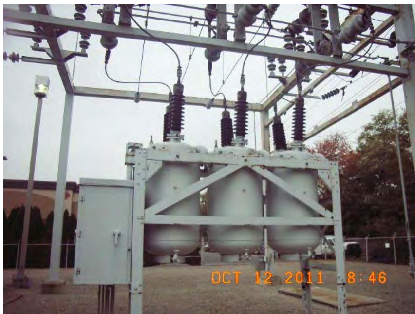
Oil Breakers at Frey's Hill Substation
