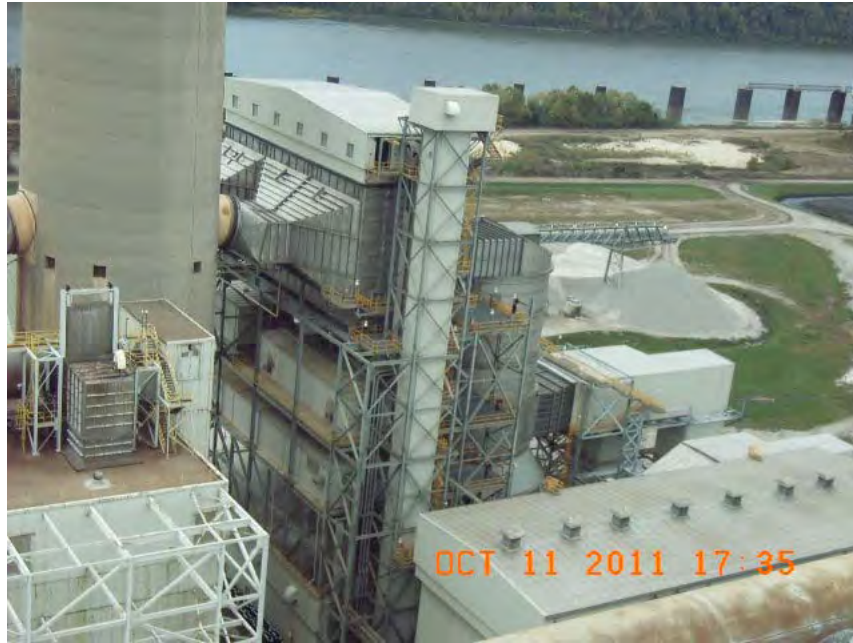
Unit 2 Scrubber at Trimble County Generating Station
