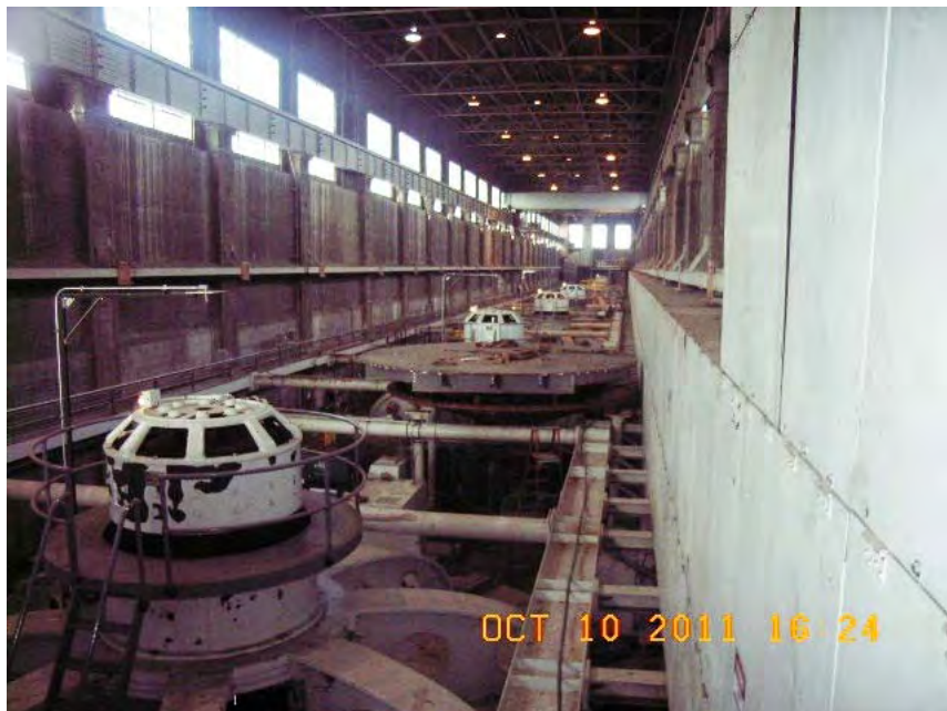
8 Generators at Ohio Falls Hydro Plant
