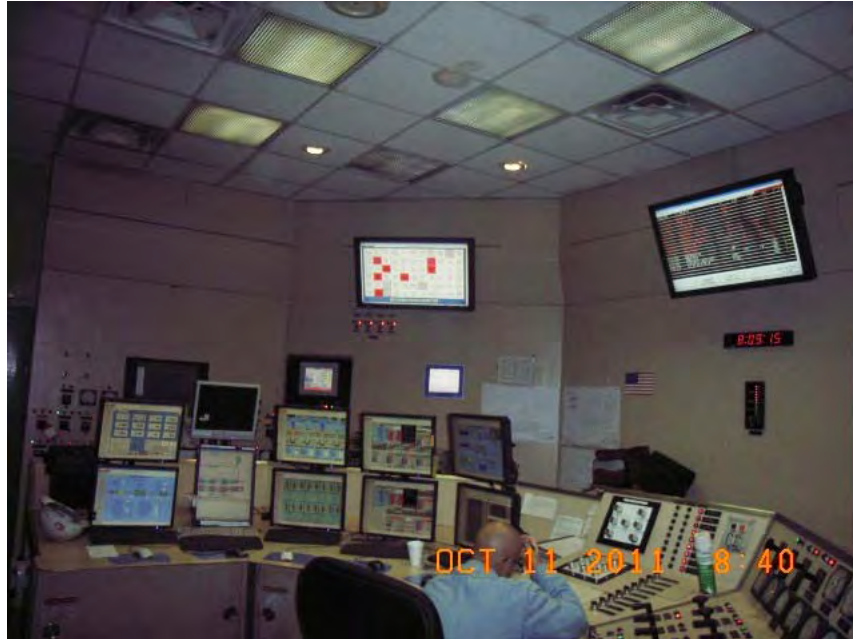
Unit 1 Controls at Brown Generating Station
