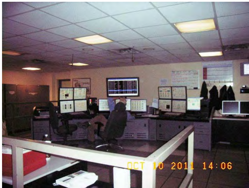
Unit 3 Controls at Mill Creek Generating Station
