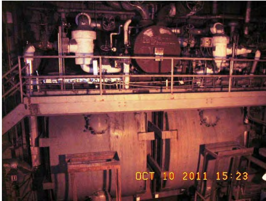
Unit 5 Condenser and Feed Water Heater at Cane Run Generating Station
