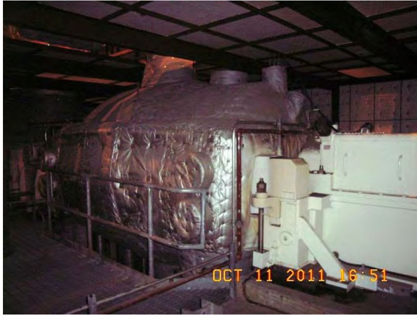
Unit 2 Generator/Exciter at Trimble County Generating Station
