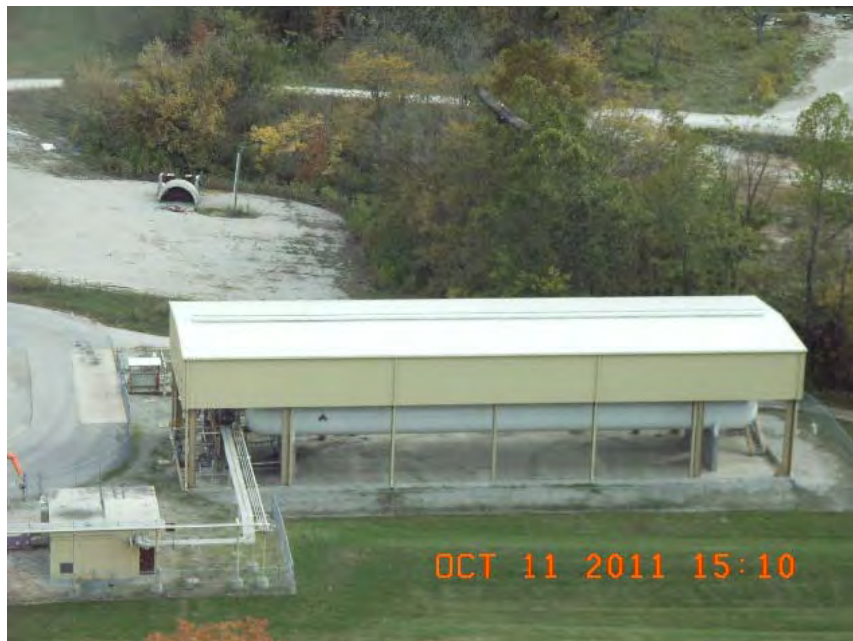
Ammonia Equipment at Ghent Generating Station
