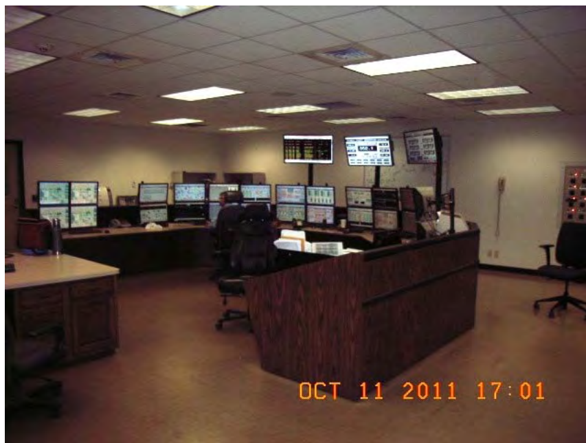
Unit 2 Controls at Trimble County Generating Station
