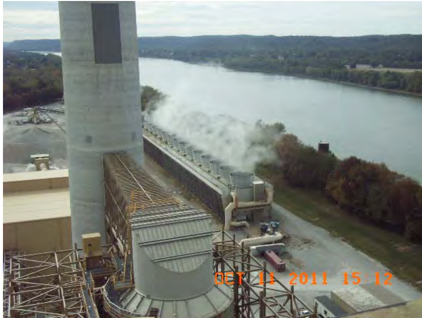
Cooling Tower and Scrubber at Ghent Generating Station
