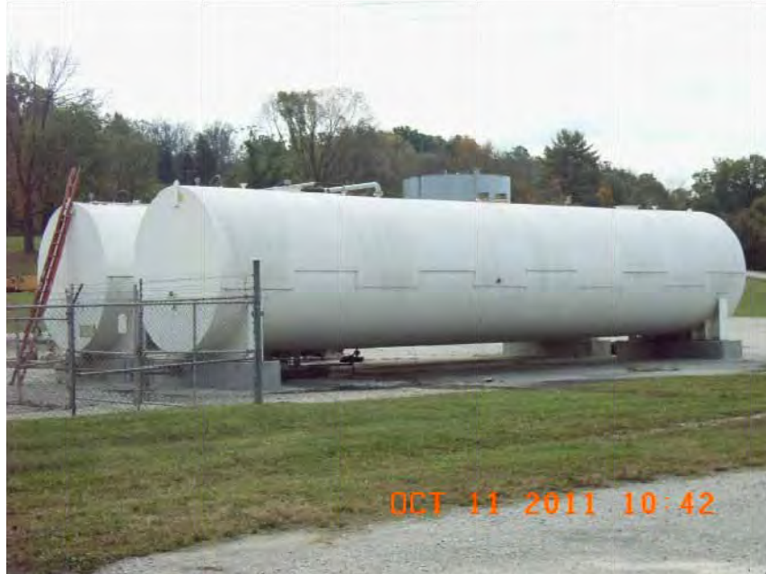
Fuel Tanks at Tyrone Generating Station
