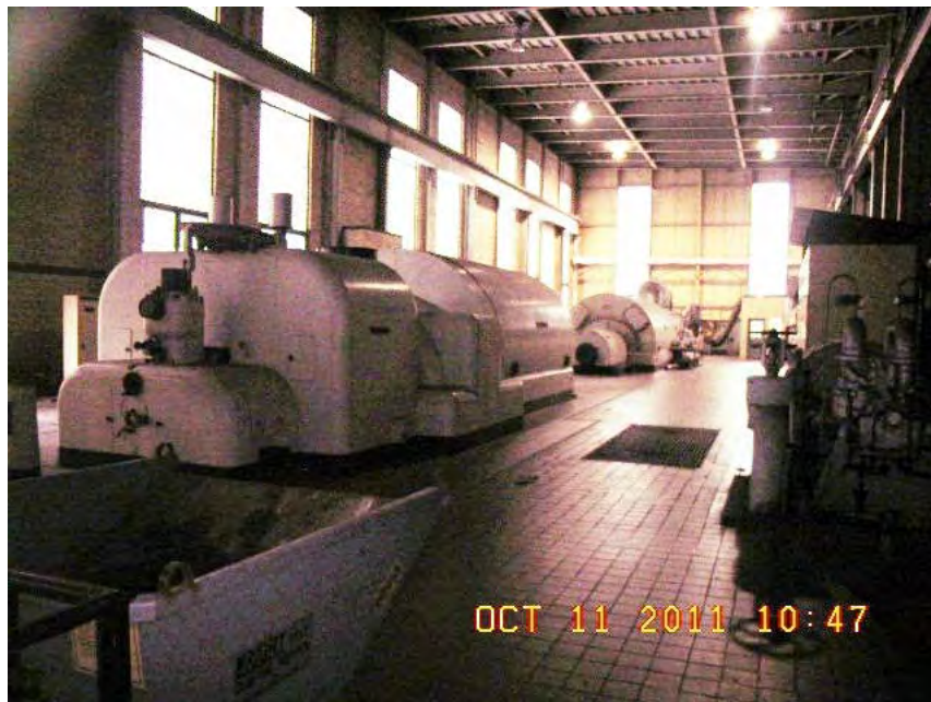
Units 2 and 3 Turbines at Tyrone Generating Station
