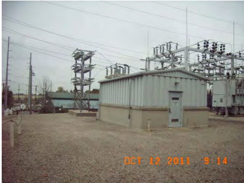
Control Building and Capacitor B__ at Collins Substation
