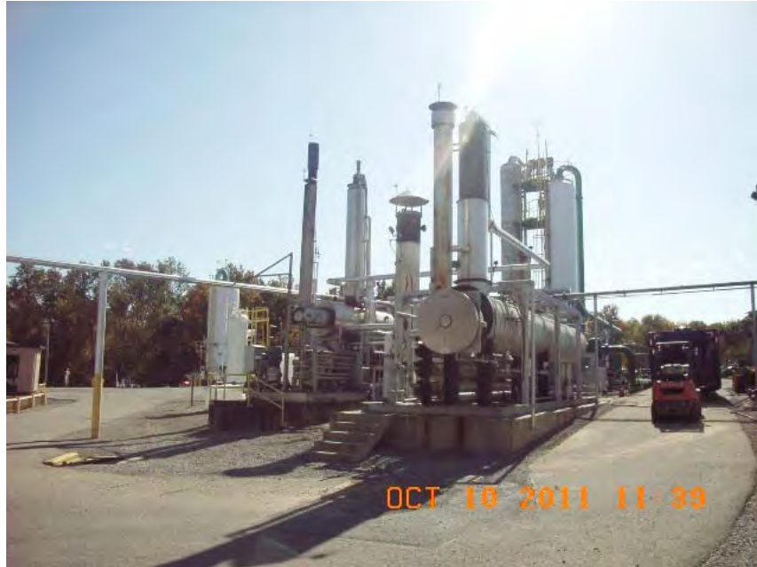
Dehydration Facility at Muldraugh Compressor Station
