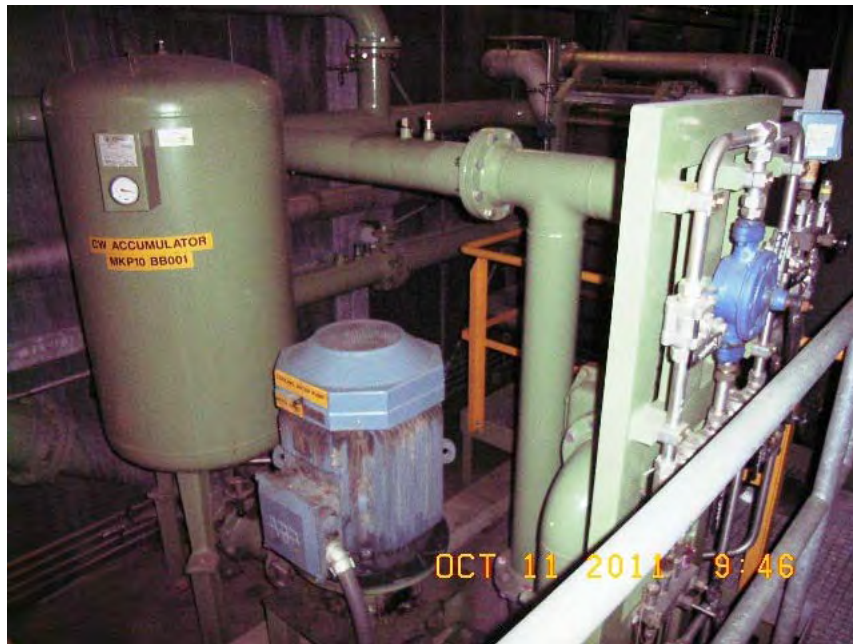
Unit 5 Pumps at Brown CT Generating Station
