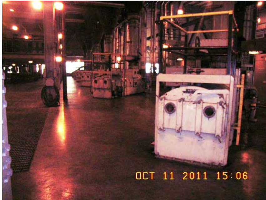
Unit 3 Coal Feeders at Ghent Generating Station
