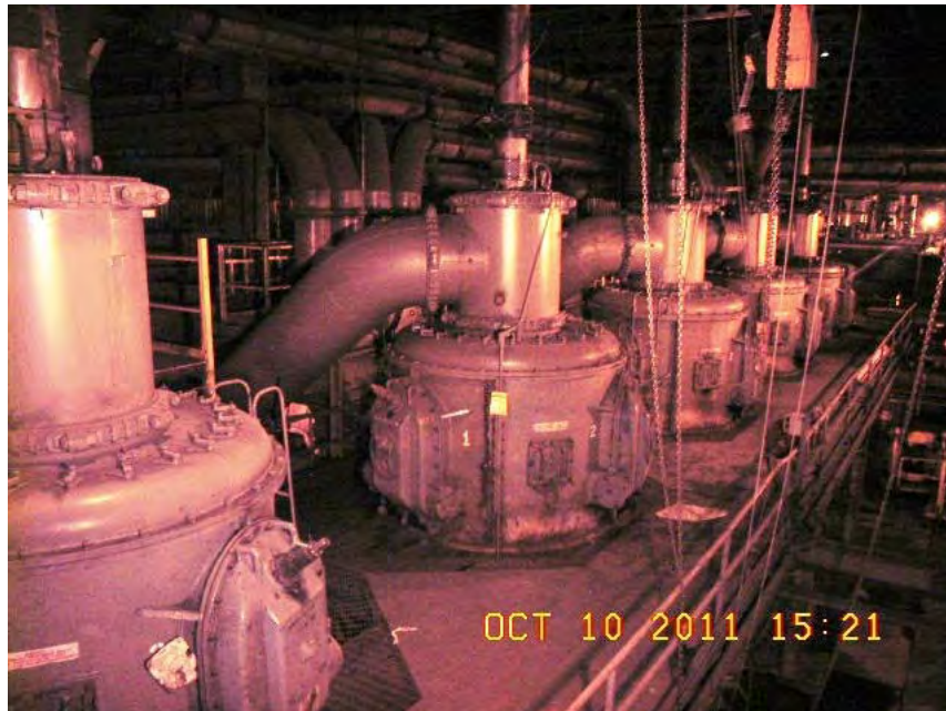
Unit 6 Pulverizers at Cane Run Generating Station
