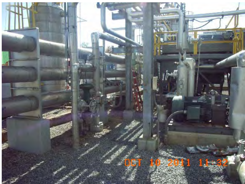
Pumps and Heat Exchangers at Muldraugh Compressor Station
