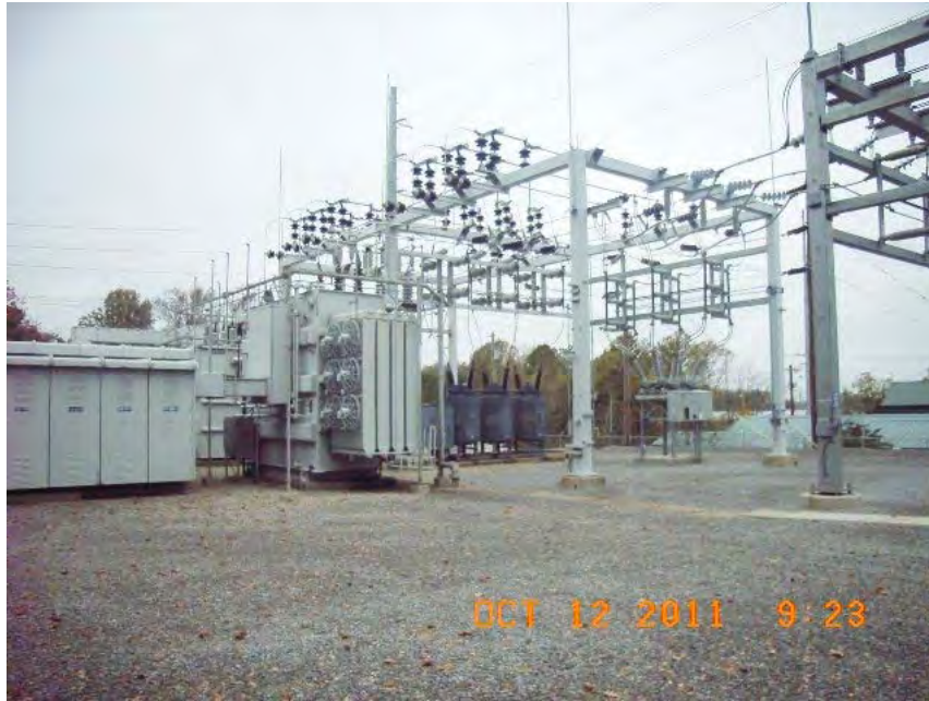
69kV Transformer and Oil Breakers at Collins Substation
