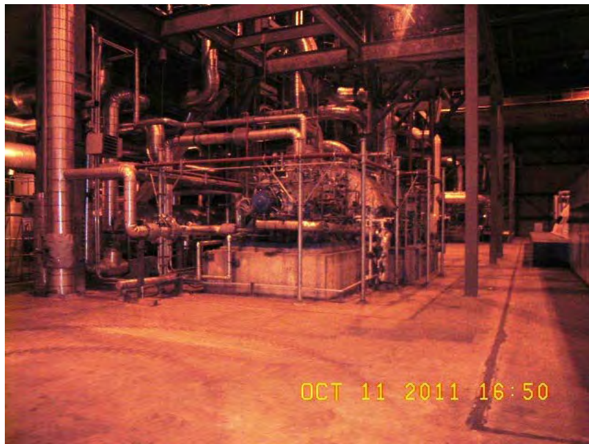
Steam Driven Boiler Feed Pump for Unit 2 at Trimble County Generating Station
