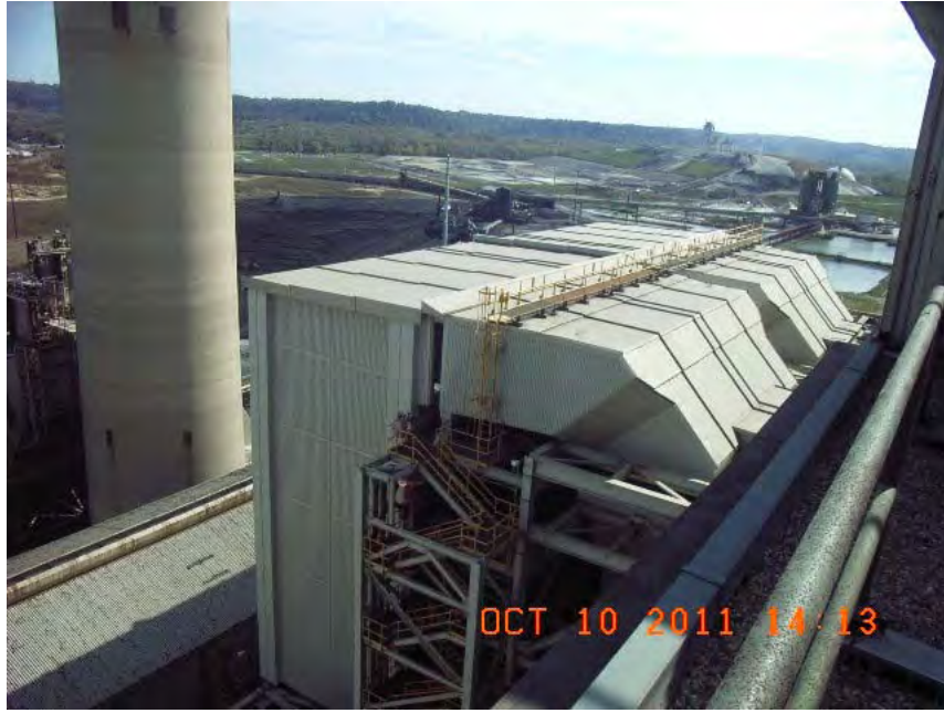
Unit 4 SCR AT Mill Creek Generating Station
