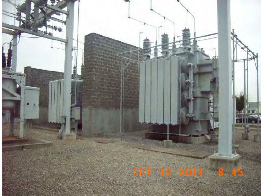
Transformers at Frey's Hill Substation
