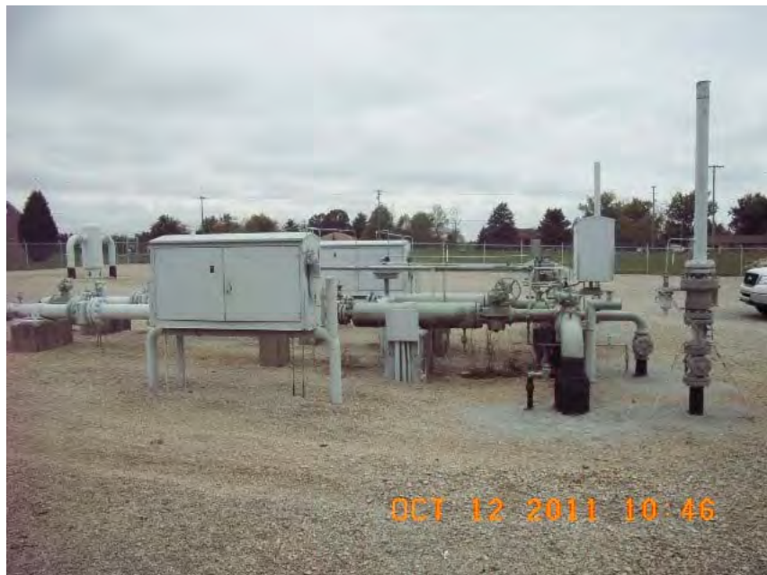
Regulator Runs at Elder Park City Gate Station
