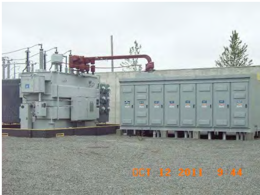
Transformer and Switchgear at Old Henry Substation
