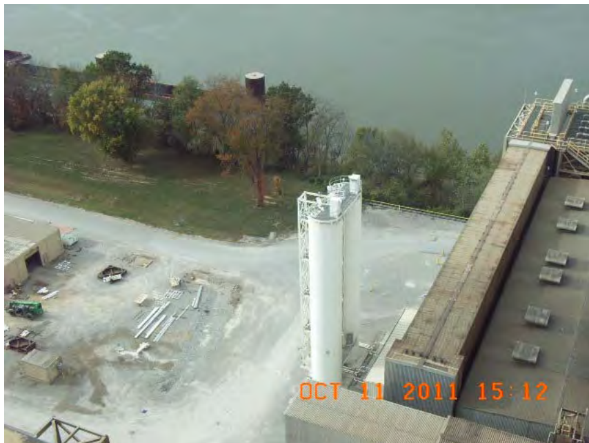
SO 3 Tanks at Ghent Generating Station
