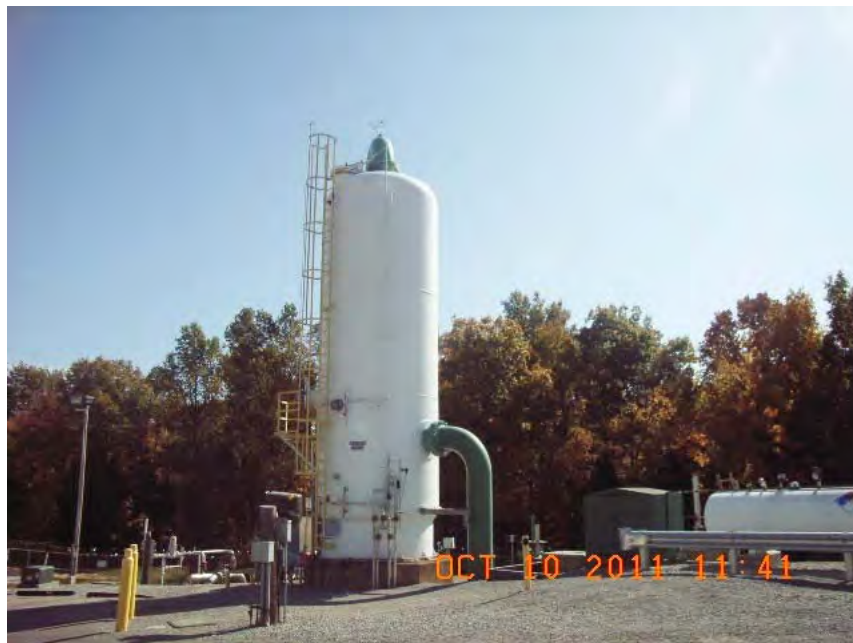
Dehydrator/Absorber at Muldraugh Compressor Station
