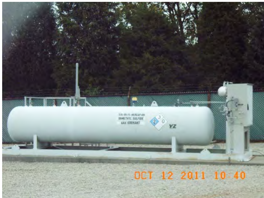
YZ Odorant Tank and Equipment at Elder Park City Gate Station
