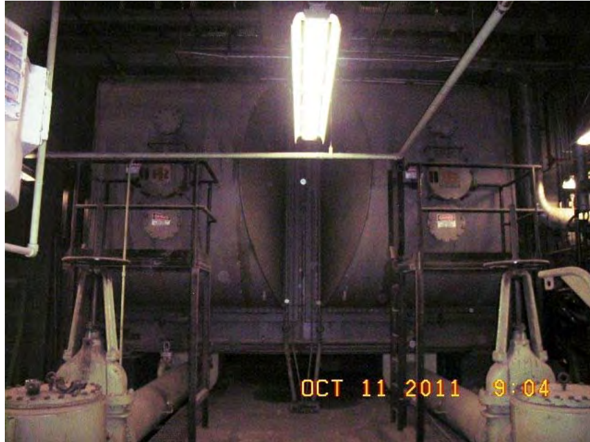
Unit 5 Condenser at Brown Generating Station
