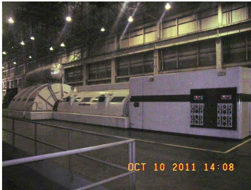
Unit 3 Turbine at Mill Creek Generating Station
