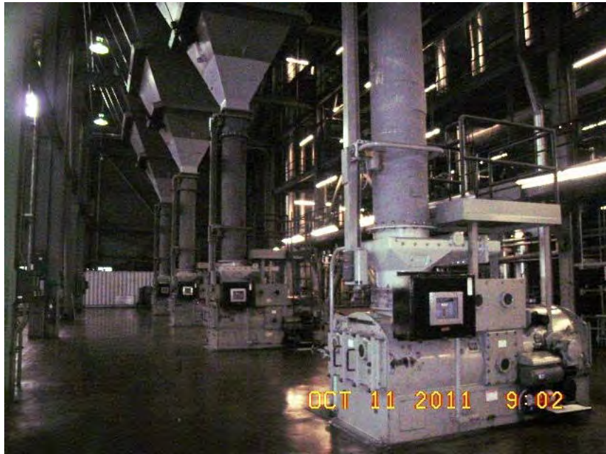
Unit 3 Coal Feeders at Brown Generating Station
