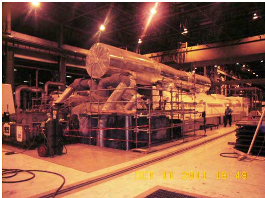
Unit 1 Turbine at Trimble County Generating Station
