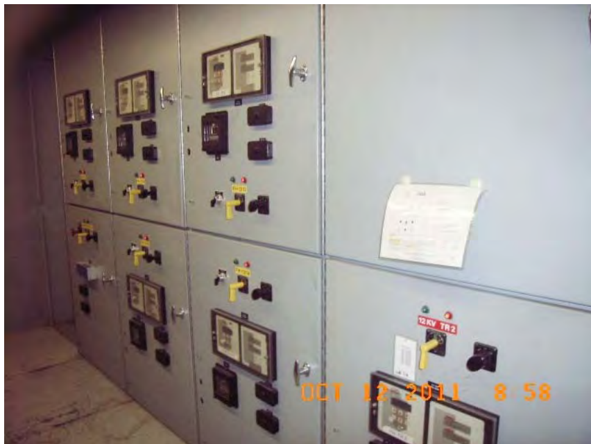
Switchgear at Frey's Substation
