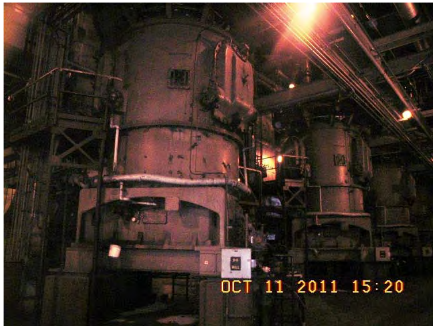
2 of 6 Pulverizers for Unit 3 at Ghent Generating Station
