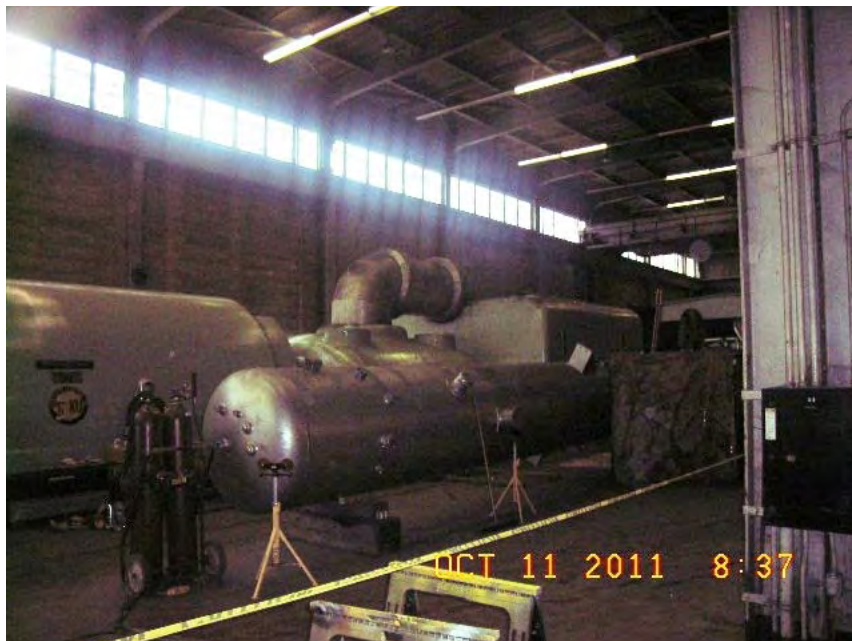
Unit 1 Turbine and LP Heater at Brown Generating Station
