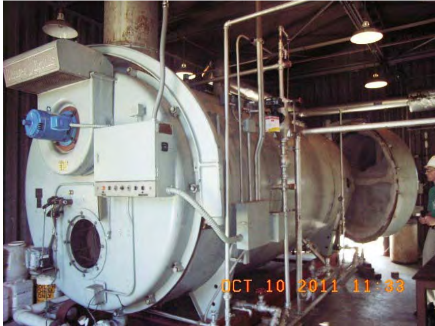
Unit 3 Steam Boiler at Muldraugh Compressor Station
