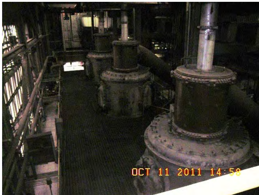
3 of 6 Pulverizers for Unit 1 at Ghent Generating Station
