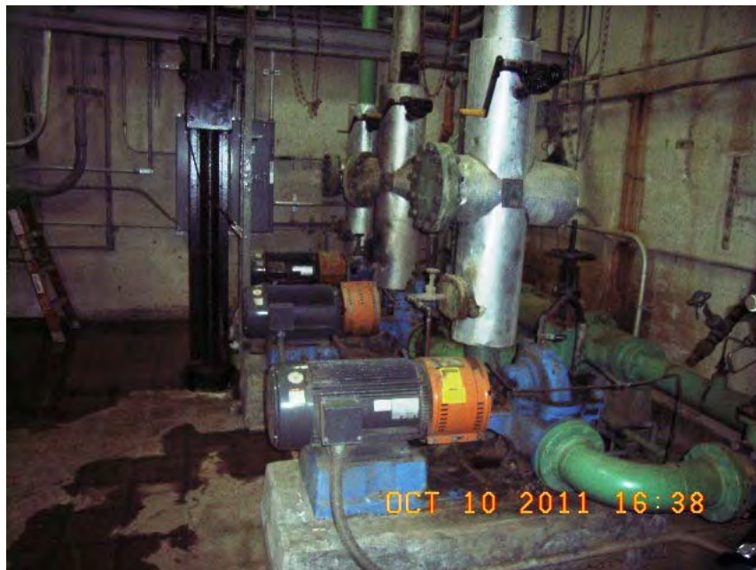
Pumps for All Units at Ohio Falls Hydro Plant
