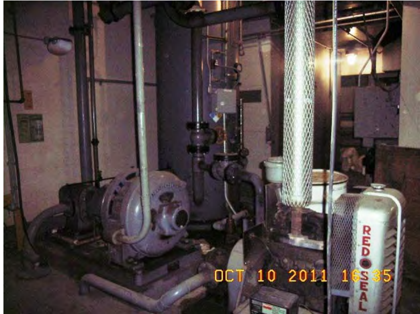
Unit 5 Governor at Ohio Falls Hydro Plant
