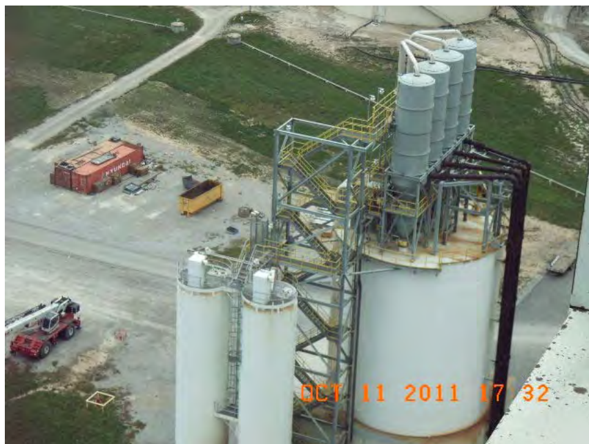
SO 3 Tanks and Fly Ash at Trimble County Generating Station
