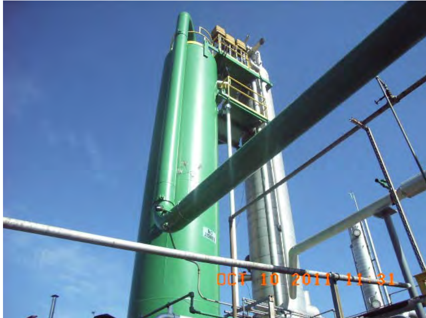
Unit 3 Absorber at Muldraugh Compressor Station
