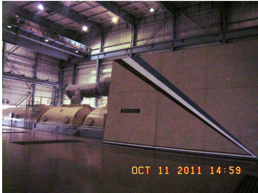
Unit 1 Turbine at Ghent Generating Station
