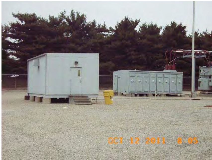
Control Building and Switchgear at Worthington Substation
