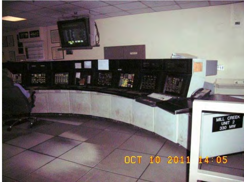
Unit 2 Controls at Mill Creek Generating Station
