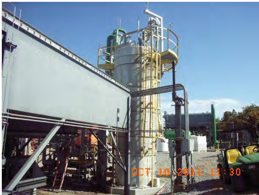
Carbon Filter at Muldraugh Compressor Station
