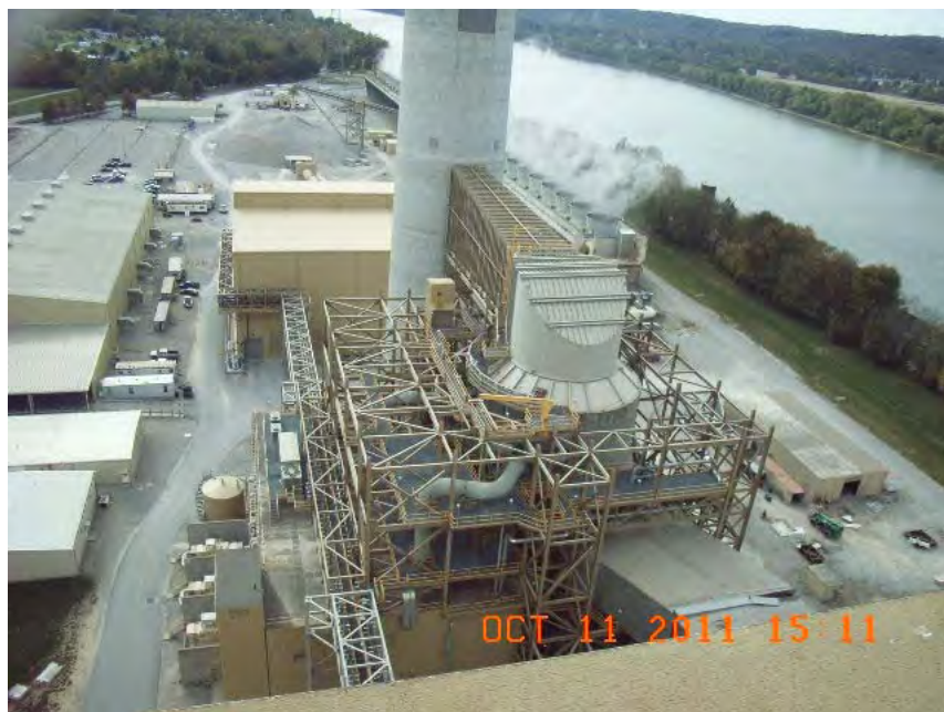
Unit 4 Scrubber at Ghent Generating Station
