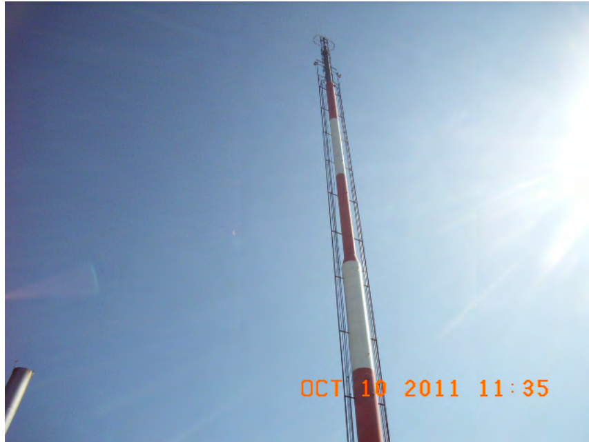
H 2 S Flare/Exhaust at Muldraugh Compressor Station
