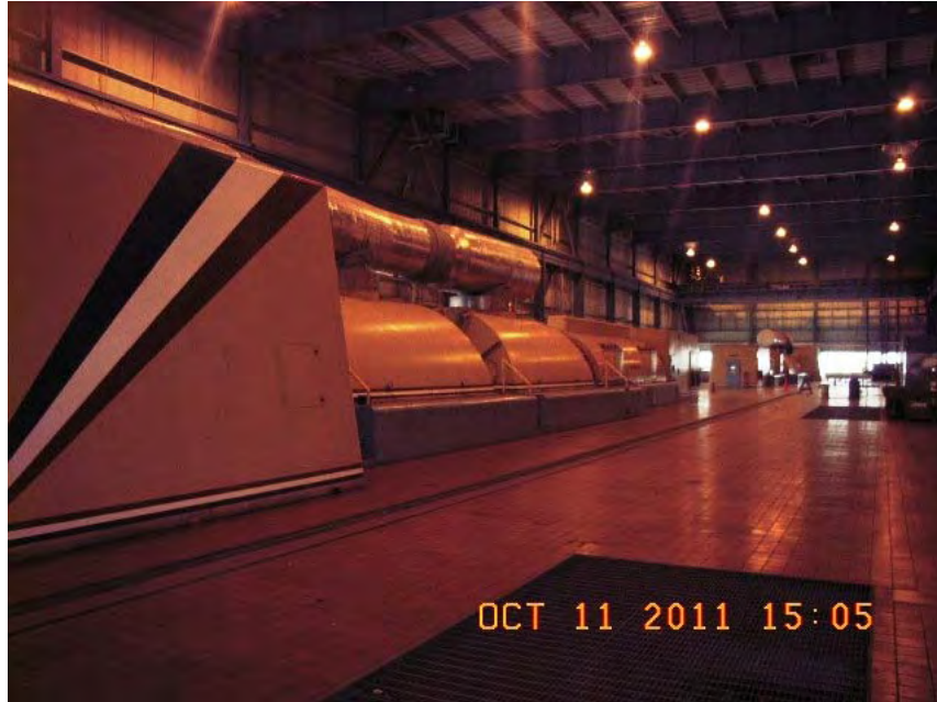
Unit 3 & 4 Turbines at Ghent Generating Station
