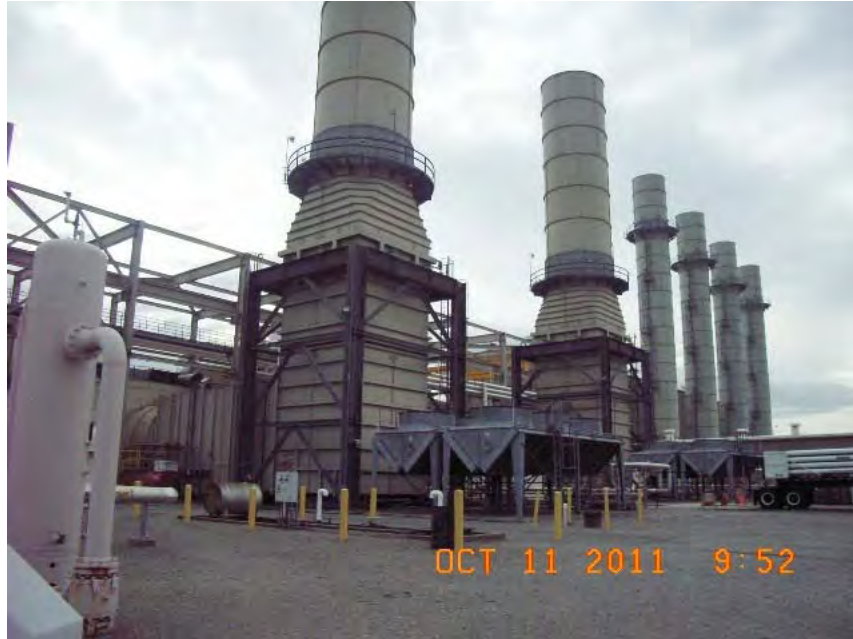
Units 6 through 11 at Brown CT Generating Station
