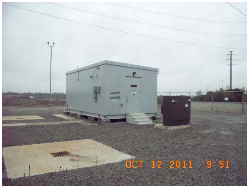
Control Building at Old Henry Substation
