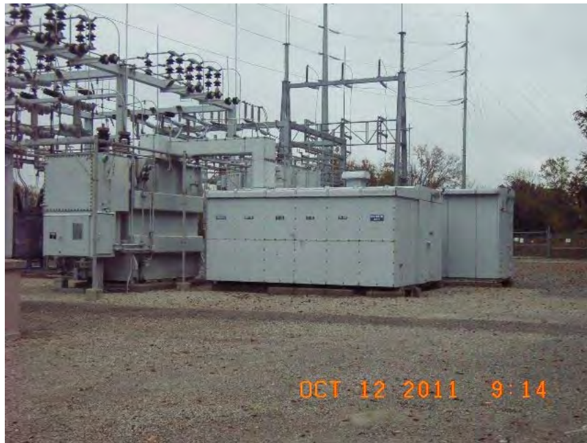
Switchgear and Transformer at Collins Substation
