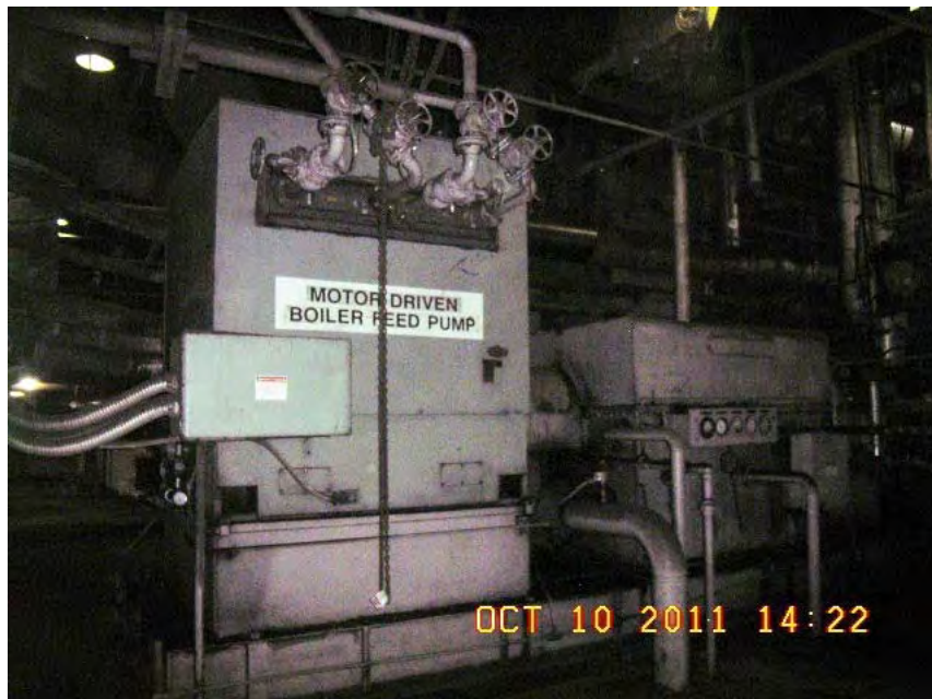
Motor Driven Boiler Feed Pump at Mill Creek Generating Station
