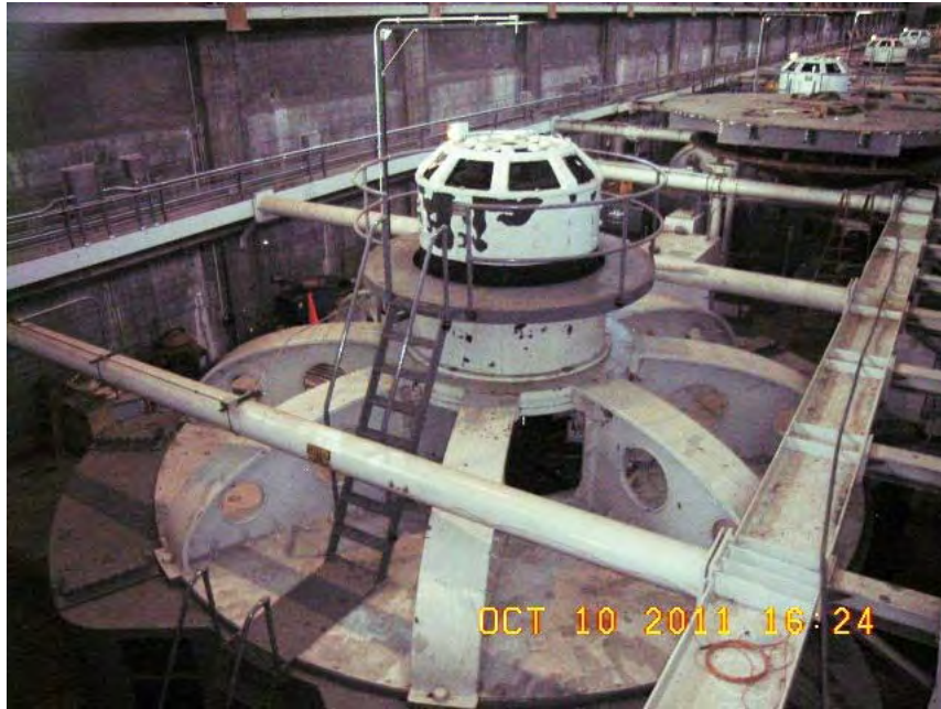
Unit 1 Generator at Ohio Falls Hydro Plant
