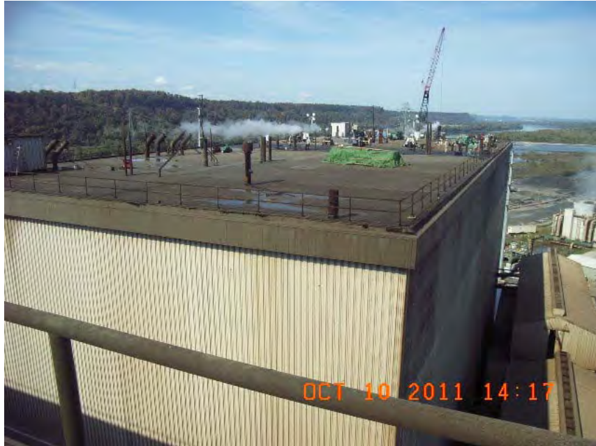
Top of Unit 2 Boiler at Mill Creek Generating Station
