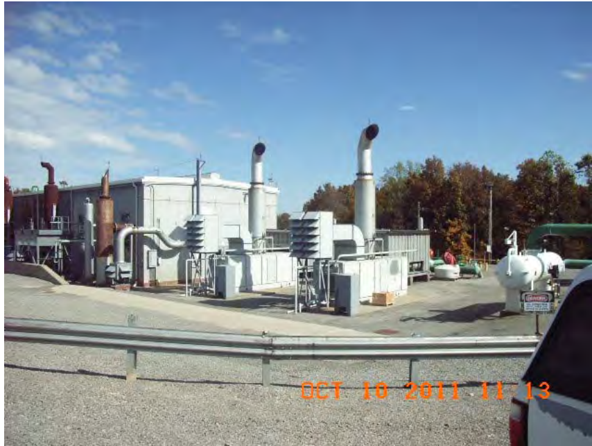
Turbine 9 & 10 Compressors at Muldraugh Compressor Station
