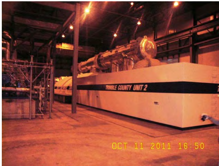
Unit 2 Turbine at Trimble County Generating Station
