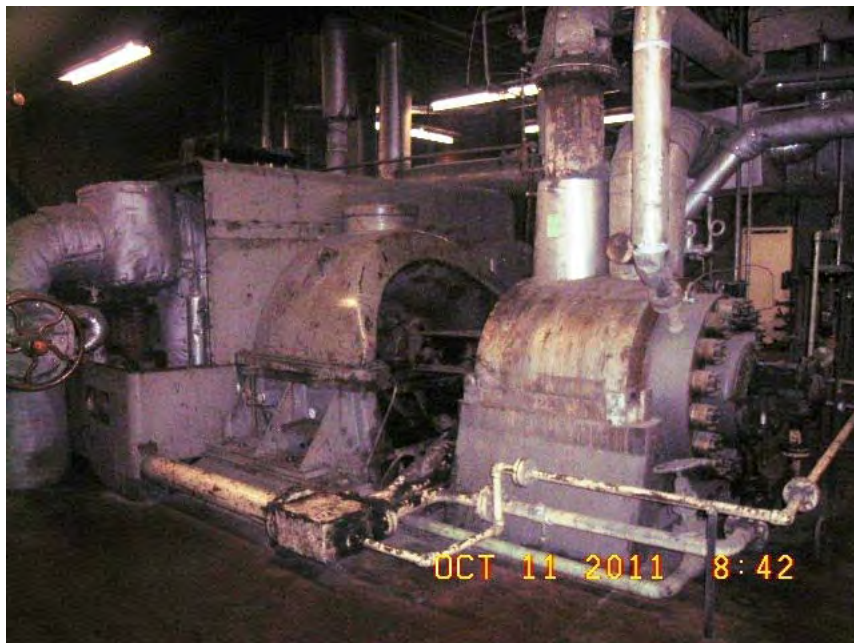
1 of 2 Boiler Feed Pumps for Unit 3 at Brown Generating Station
