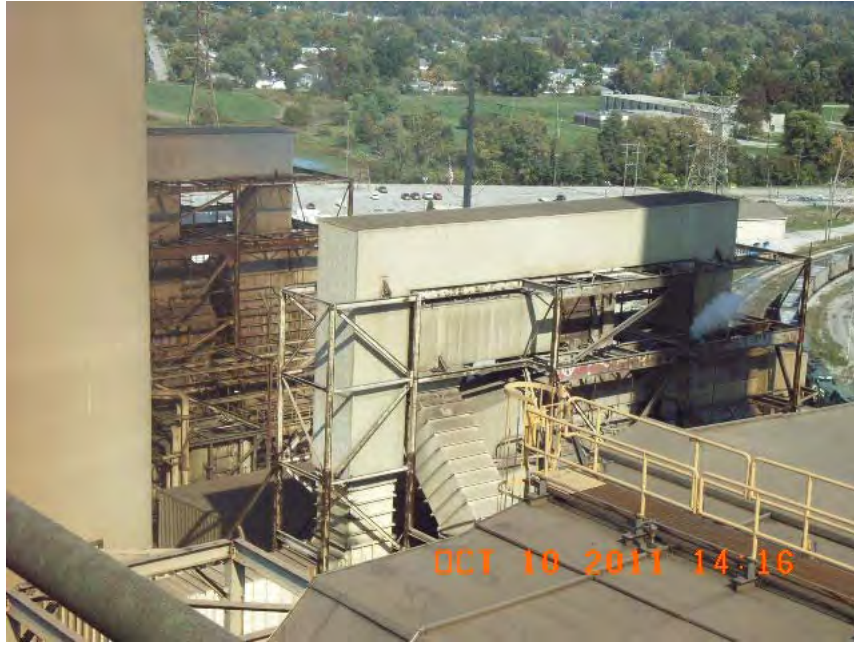
1 & 2 Scrubber at Mill Creek Generating Station
