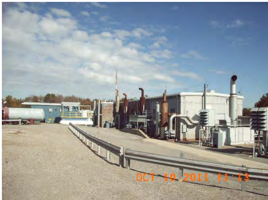
Exhaust for Compressors at Muldraugh Compressor Station
