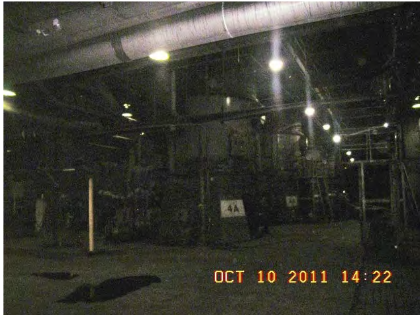
1 of 5 Pulverizers for Unit 4 at Mill Creek Generating Station
