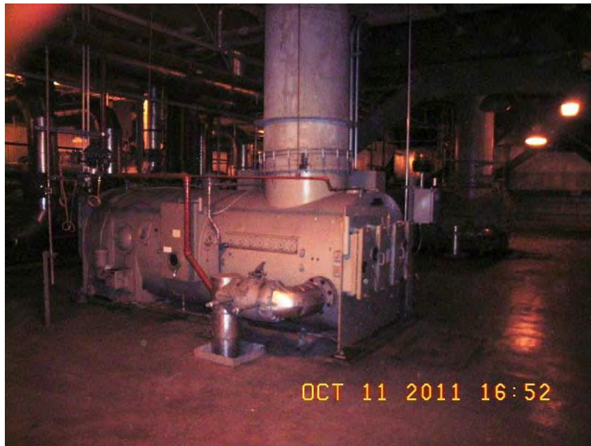
Coal Feeders at Trimble County Generating Station
