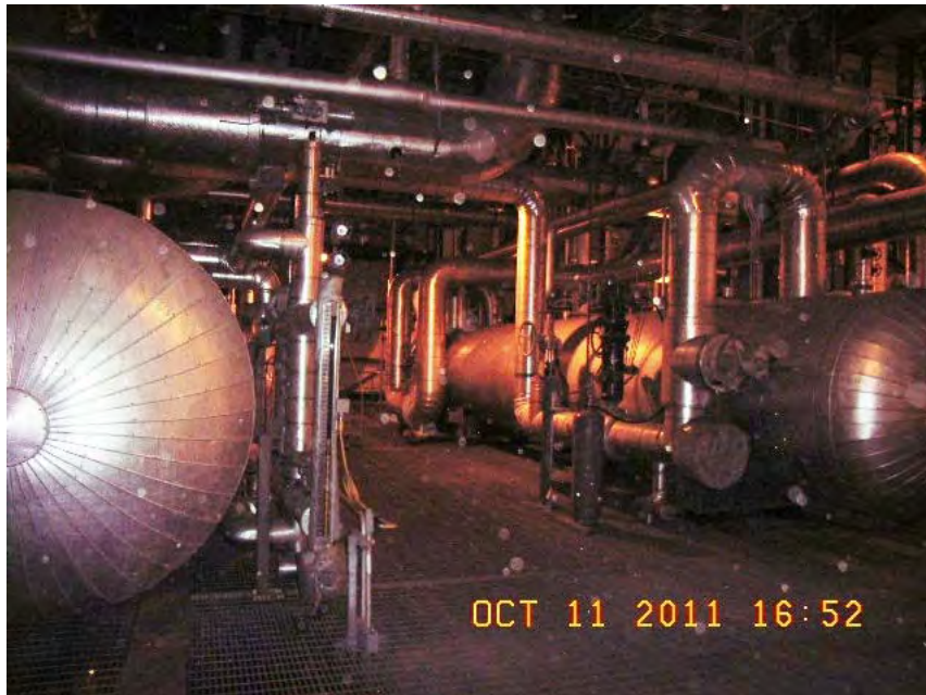
Feed Water Heaters at Trimble County Generating Station
