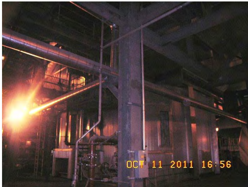
1 of 2 Air Heaters for Unit 2 at Trimble County Generating Station
