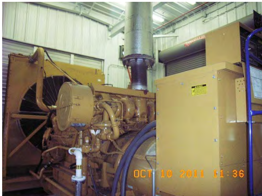
Emergency Generator (1996) at Muldraugh Compressor Station
