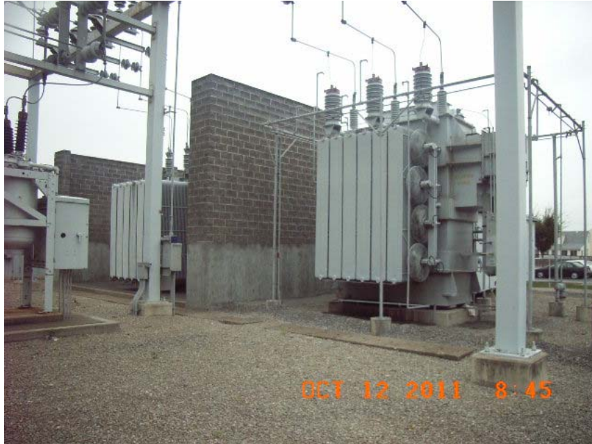
Transformers at Frey's Hill Substation
