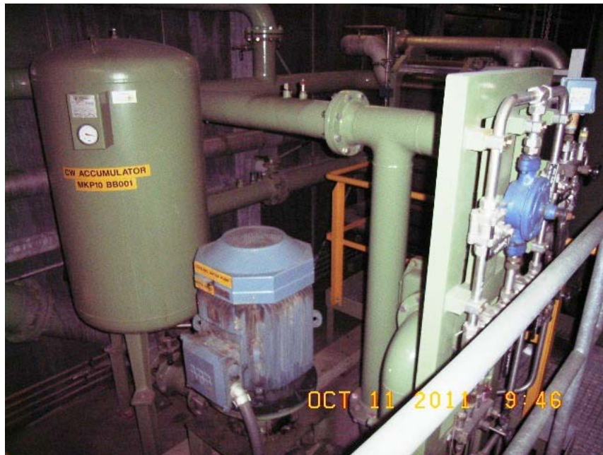
Unit 5 Pumps at Brown CT Generating Station
