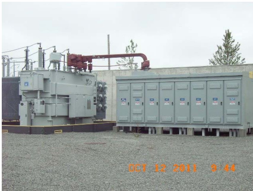
Transformer and Switchgear at Old Henry Substation
