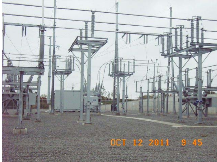
SF 6 Breakers and Bus Work at Old Henry Substation
