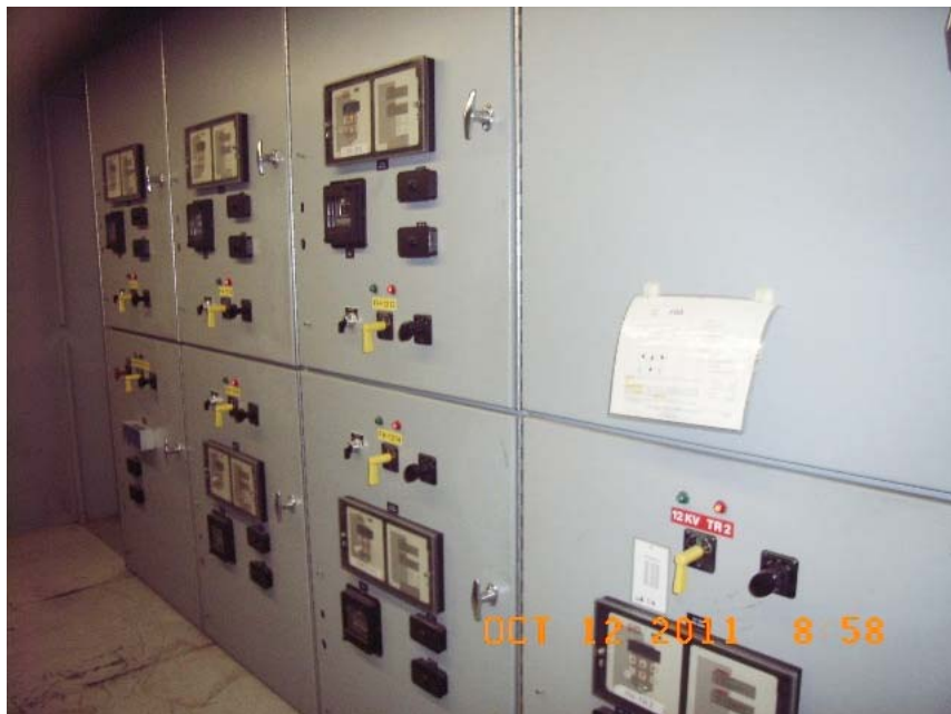
Switchgear at Frey's Substation
