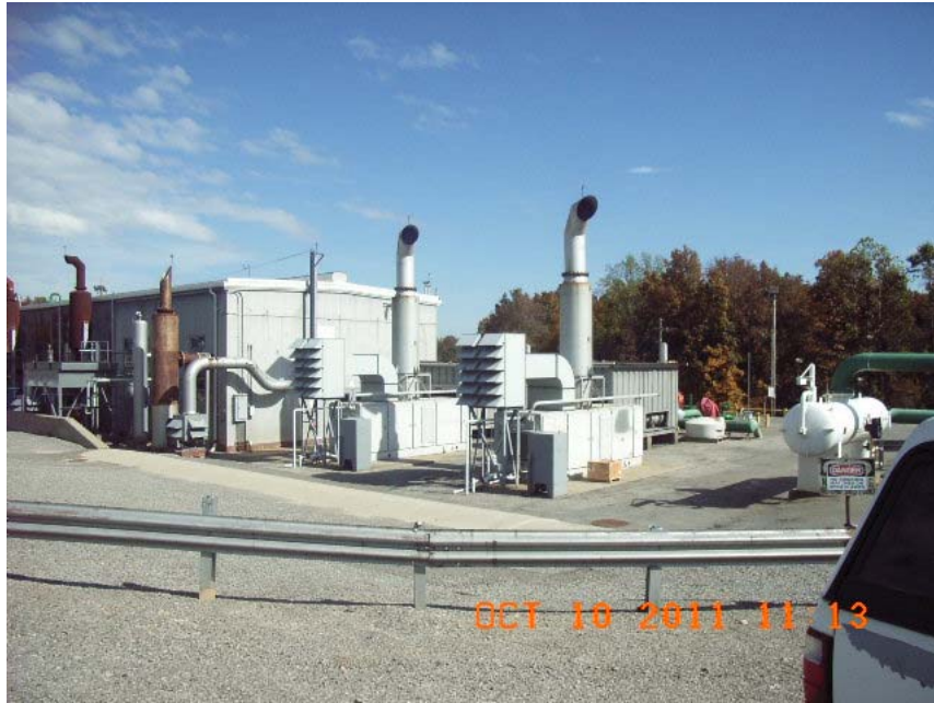
Turbine 9 & 10 Compressors at Muldraugh Compressor Station
