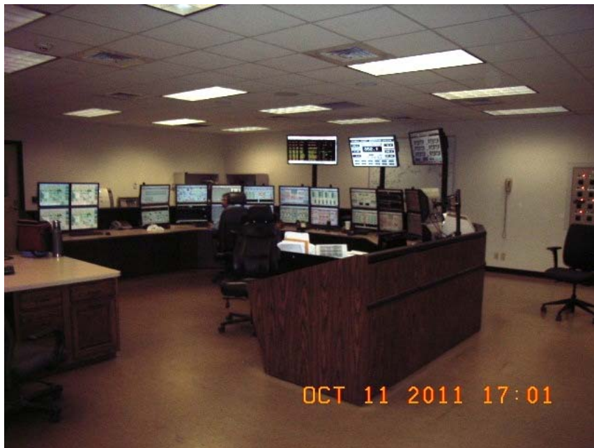
Unit 2 Controls at Trimble County Generating Station
