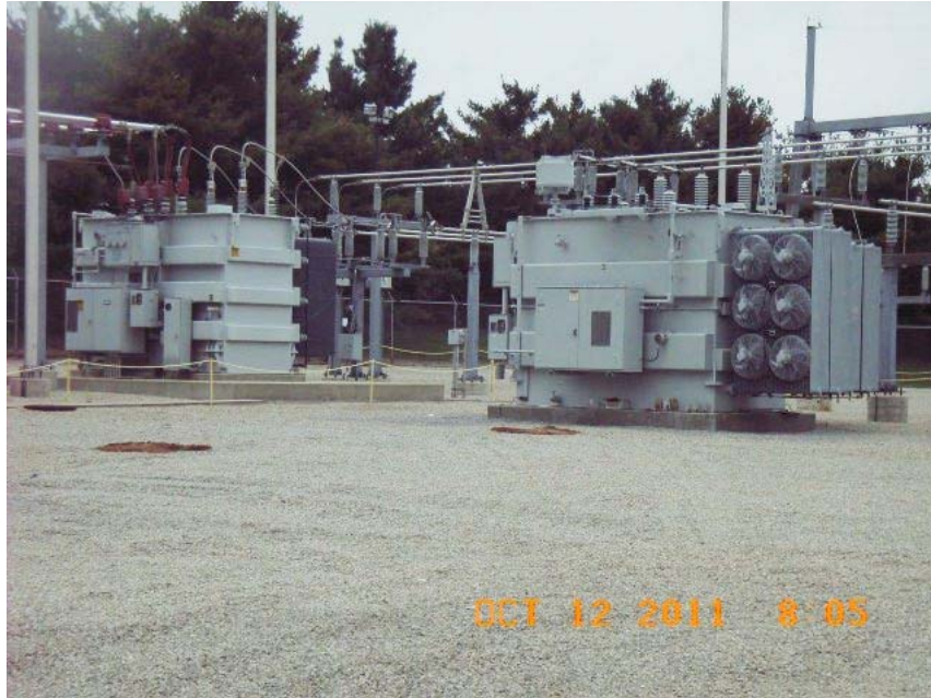
Transformers at Worthington Substation
