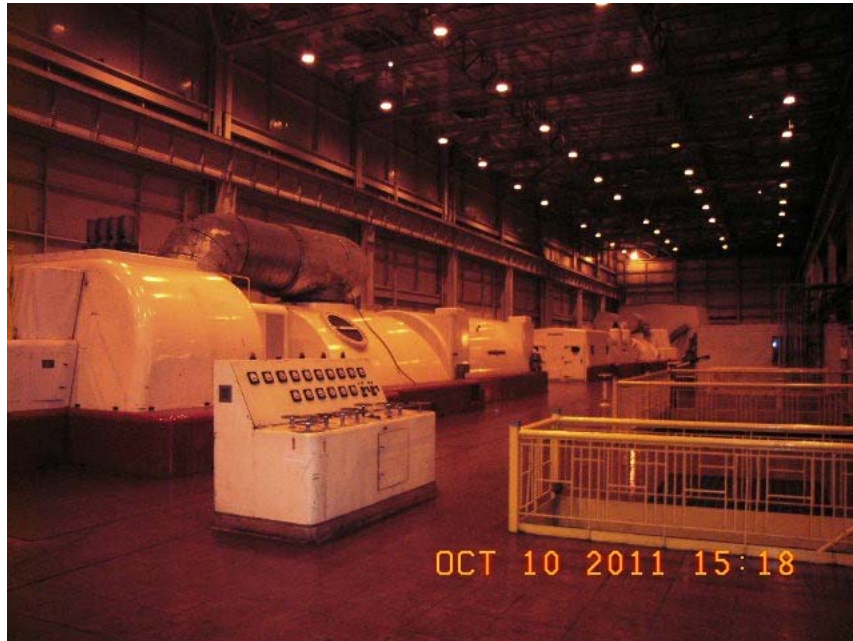
Turbines 4 and 5 at Cane Run Generating Station
