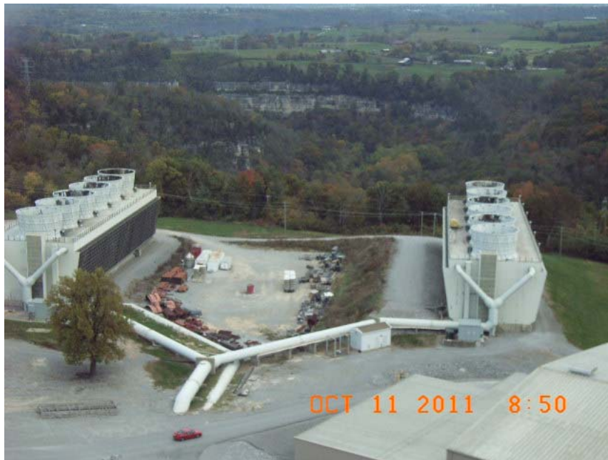
Cooling Towers for Unit 3 at Brown Generating Station
