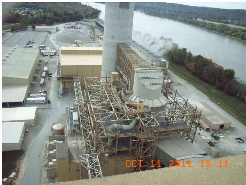
Unit 4 Scrubber at Ghent Generating Station
