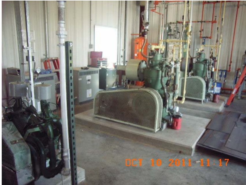
3 New Air Compressors at Muldraugh Compressor Station
