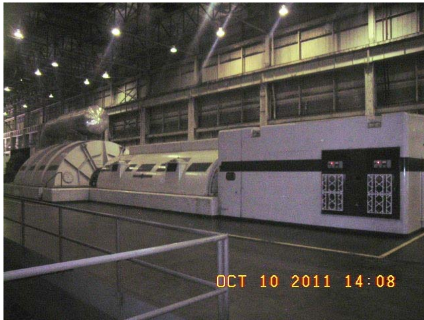
Unit 3 Turbine at Mill Creek Generating Station
