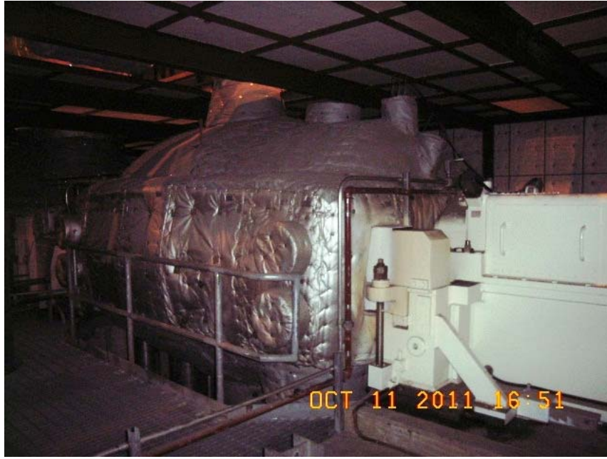
Unit 2 Generator/Exciter at Trimble County Generating Station
