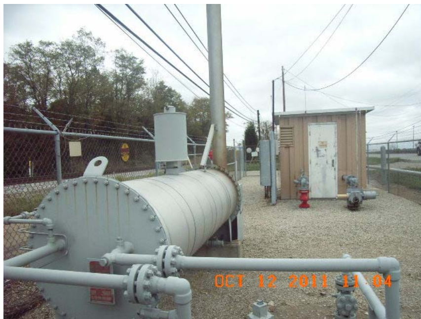
Heater and Measurement Building at LaGrange City Gate Station
