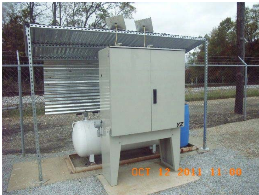
Odorant Equipment at LaGrange City Gate Station
