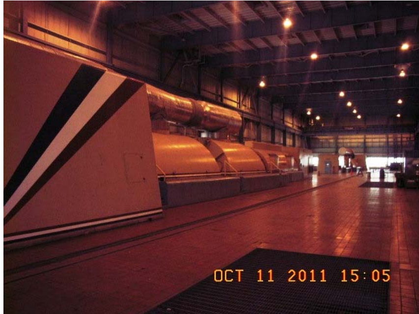
Unit 3 & 4 Turbines at Ghent Generating Station
