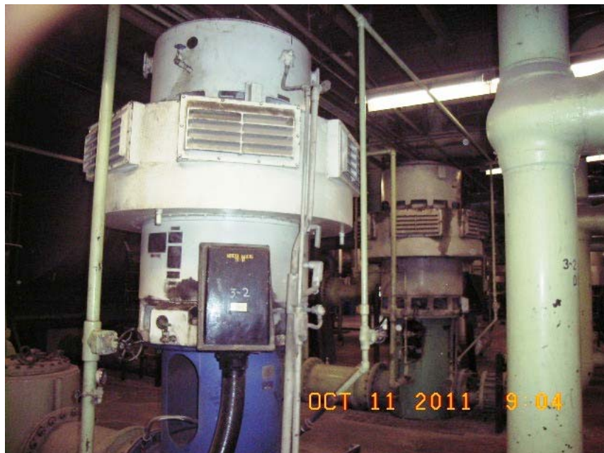
Unit 5 Condensate Pumps at Brown Generating Station
