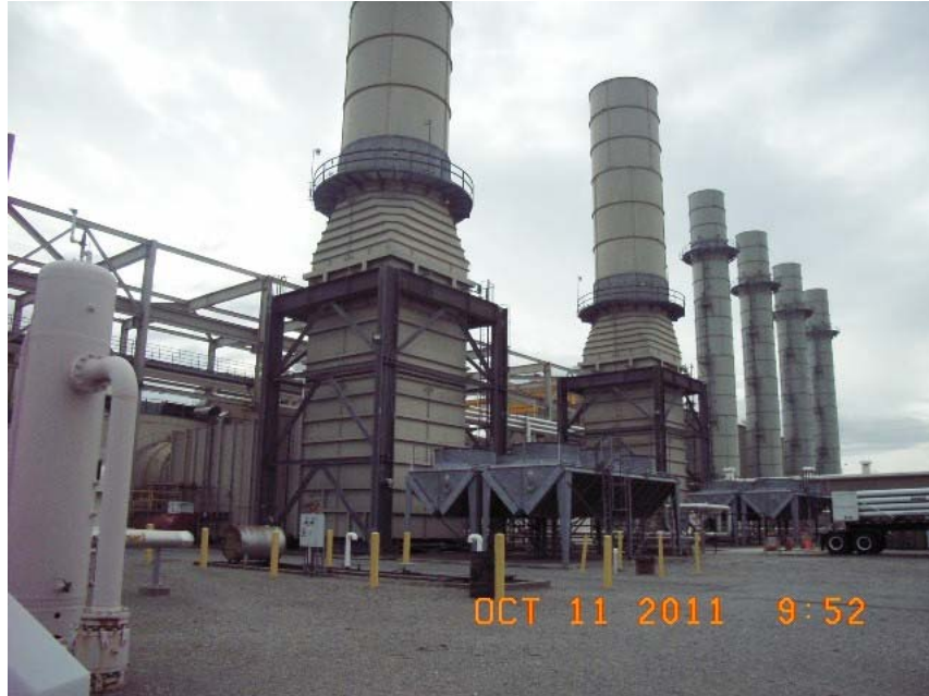
Units 6 through 11 at Brown CT Generating Station
