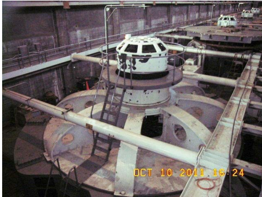
Unit 1 Generator at Ohio Falls Hydro Plant
