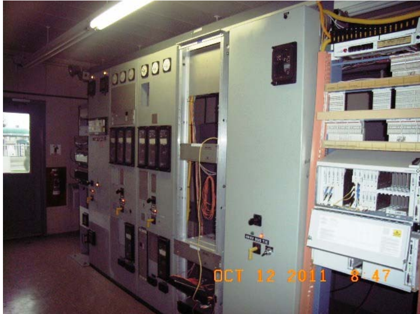
Controls at Frey's Hill Substation
