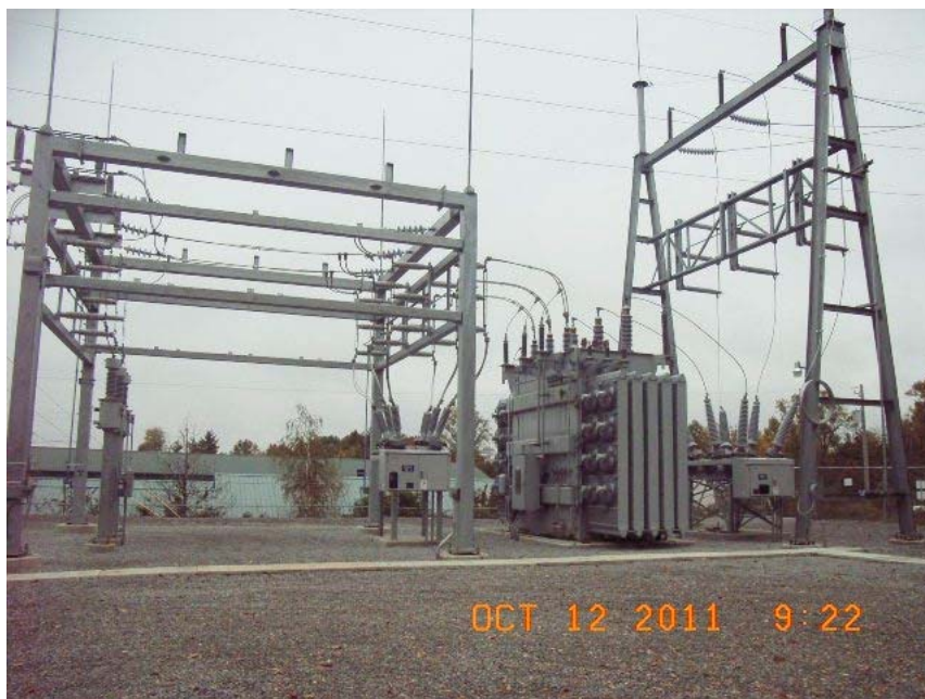
138kV Transformer and SF 6 Breakers at Collins Substation
