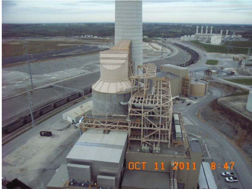
Scrubber at Brown Generating Station
