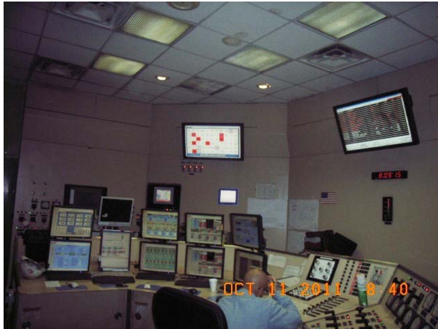
Unit 1 Controls at Brown Generating Station
