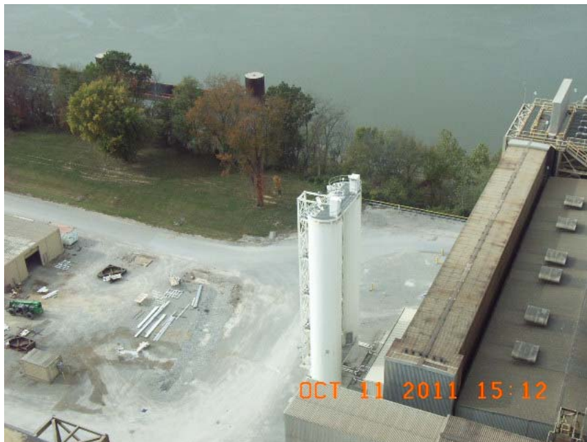
SO 3 Tanks at Ghent Generating Station
