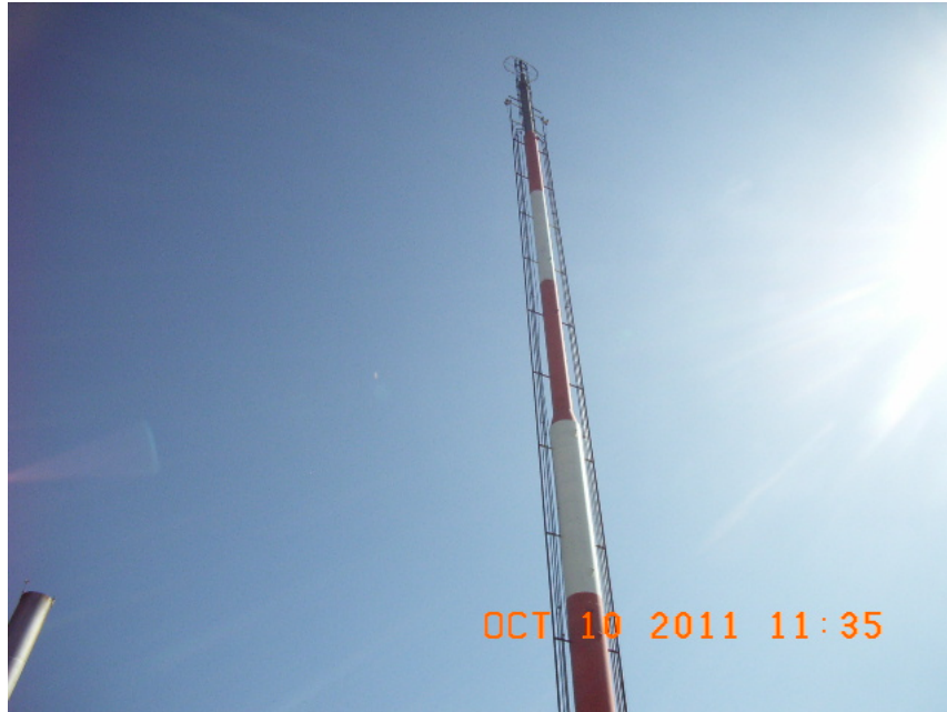
H 2 S Flare/Exhaust at Muldraugh Compressor Station
