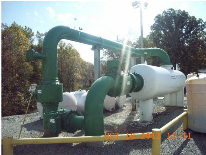
Filter Separator at Muldraugh Compressor Station
