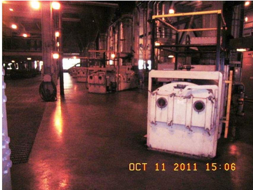
Unit 3 Coal Feeders at Ghent Generating Station
