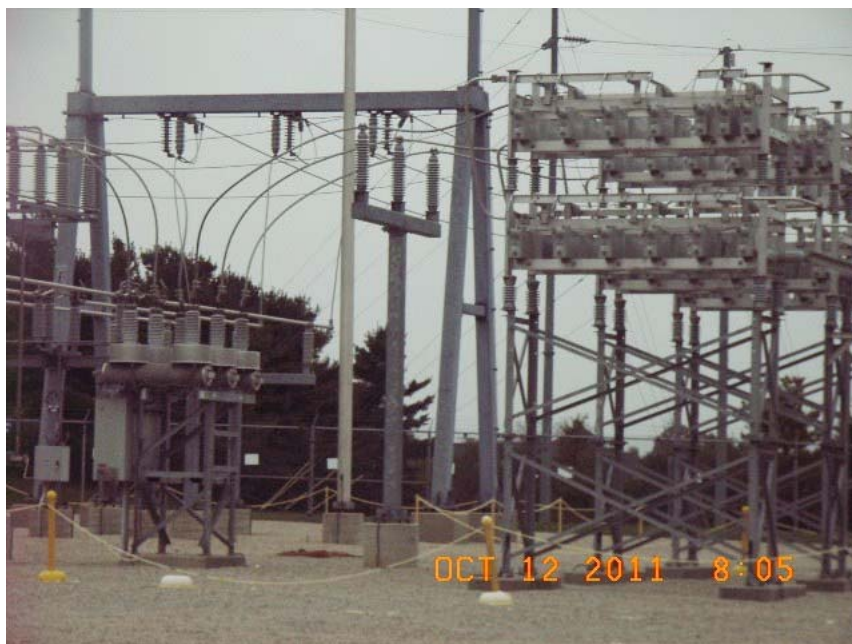
Capacitor Bank and SF 6 Breakers at Worthington Substation
