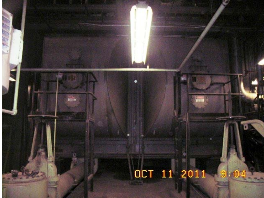
Unit 5 Condenser at Brown Generating Station
