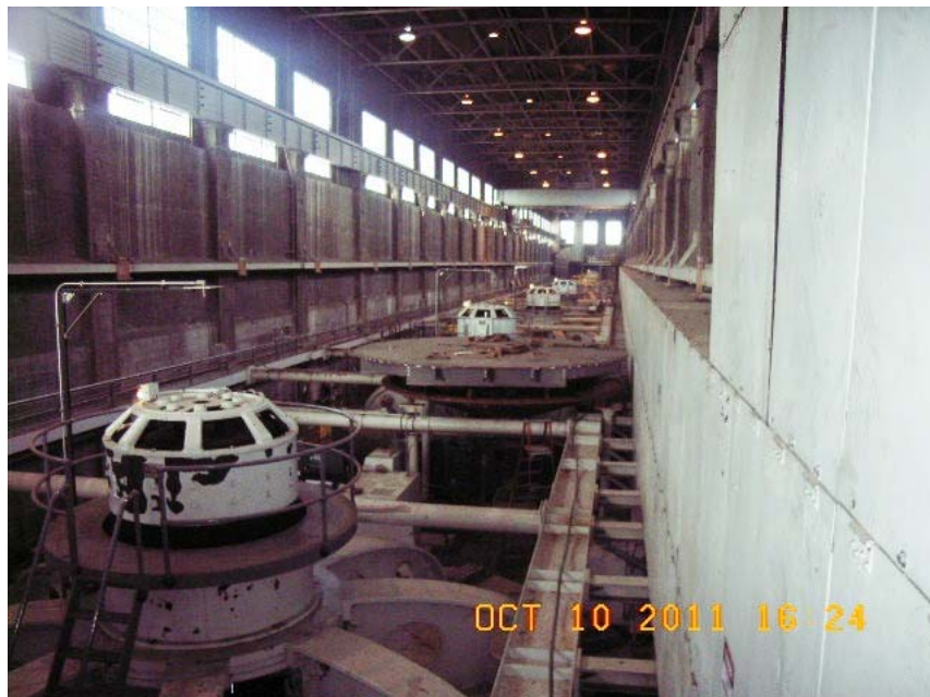
8 Generators at Ohio Falls Hydro Plant
