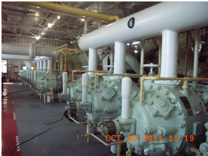
Compressors 6, 7 & 8 at Muldraugh Compressor Station
