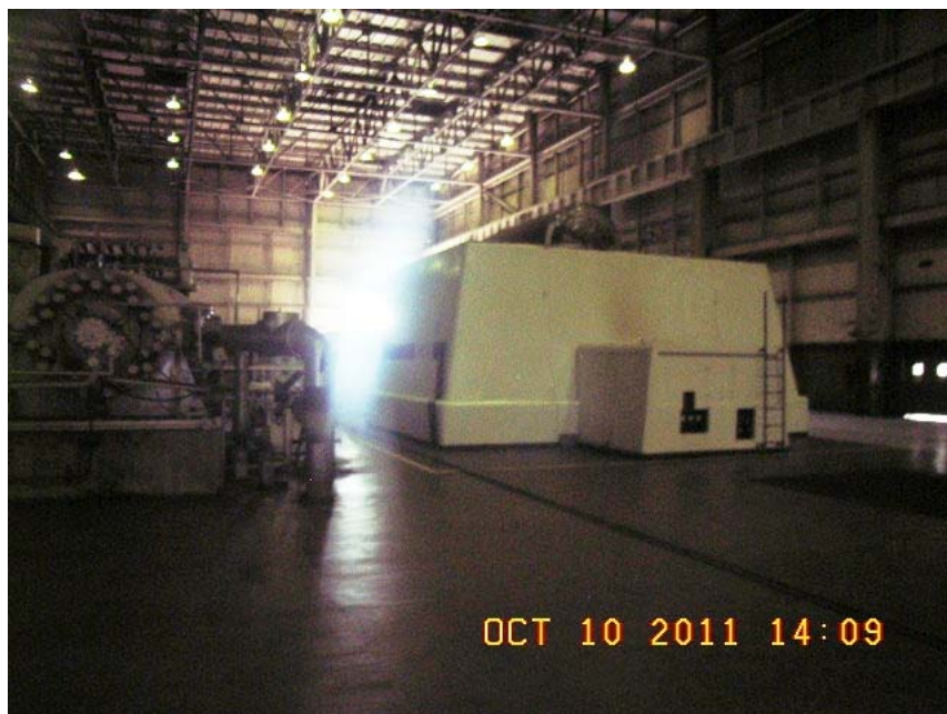
Unit 4 Turbine and Feed Pump at Mill Creek Generating Station
