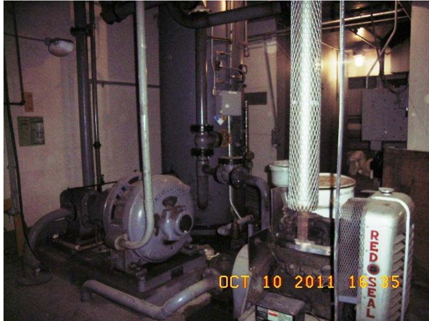
Unit 5 Governor at Ohio Falls Hydro Plant
