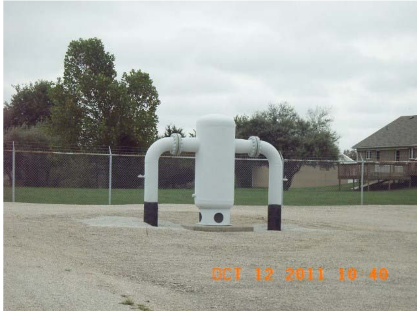
Separator at Elder Park City Gate Station
