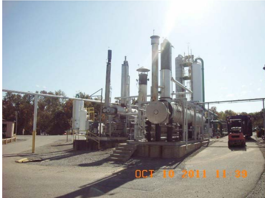
Dehydration Facility at Muldraugh Compressor Station
