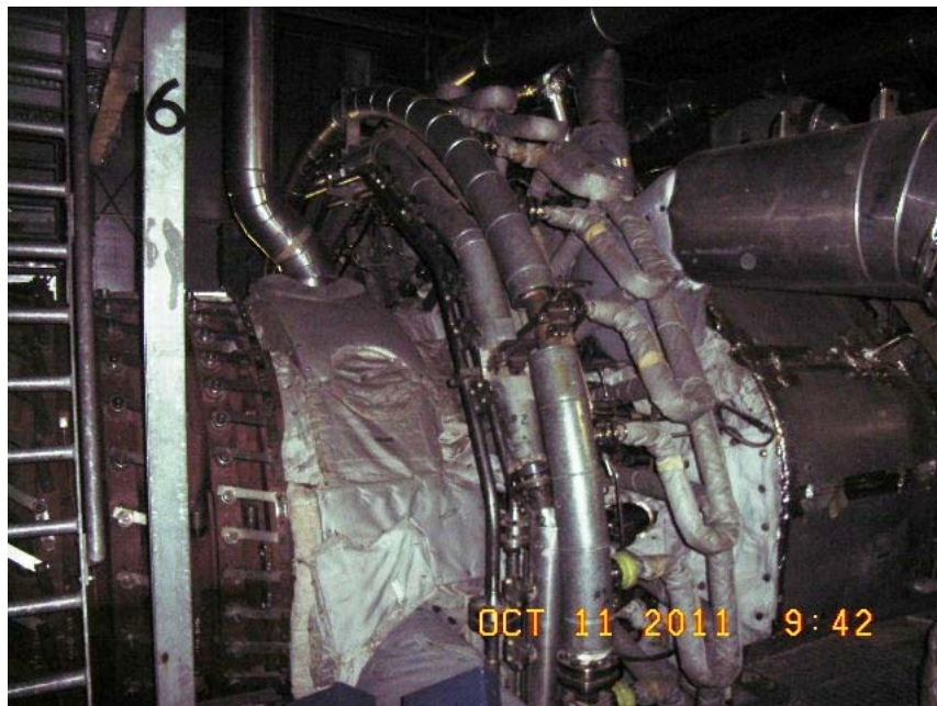
Unit 6 Turbine at Brown CT Generating Station
