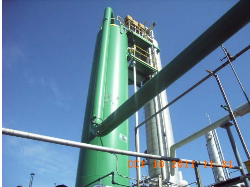
Unit 3 Absorber at Muldraugh Compressor Station
