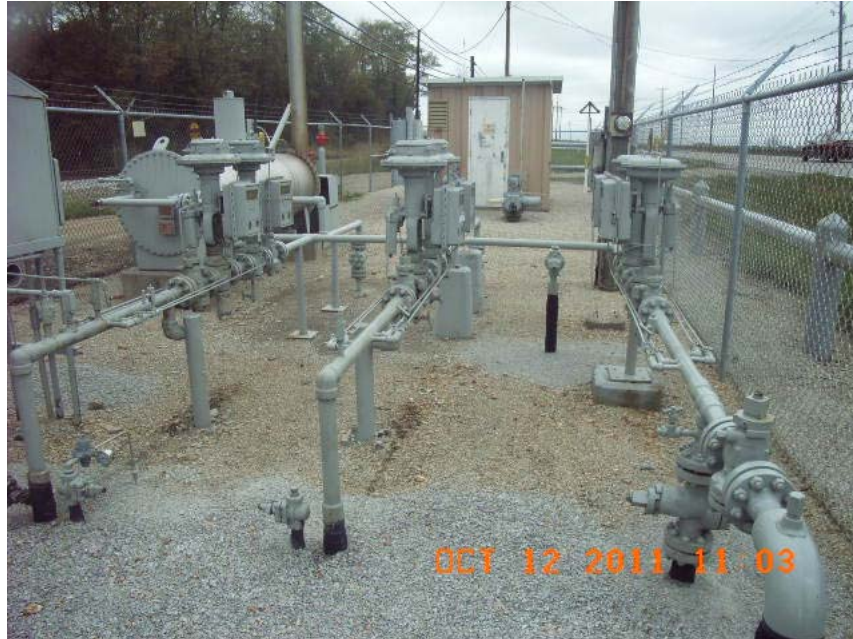
Regulator Runs at LaGrange City Gate Station
