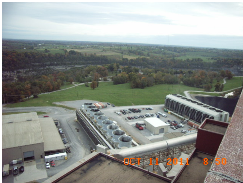
Cooling Towers for Units 1 & 2 at Brown Generating Station
