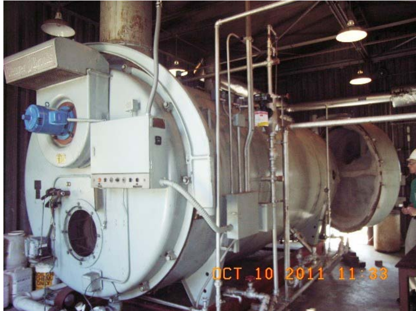
Unit 3 Steam Boiler at Muldraugh Compressor Station
