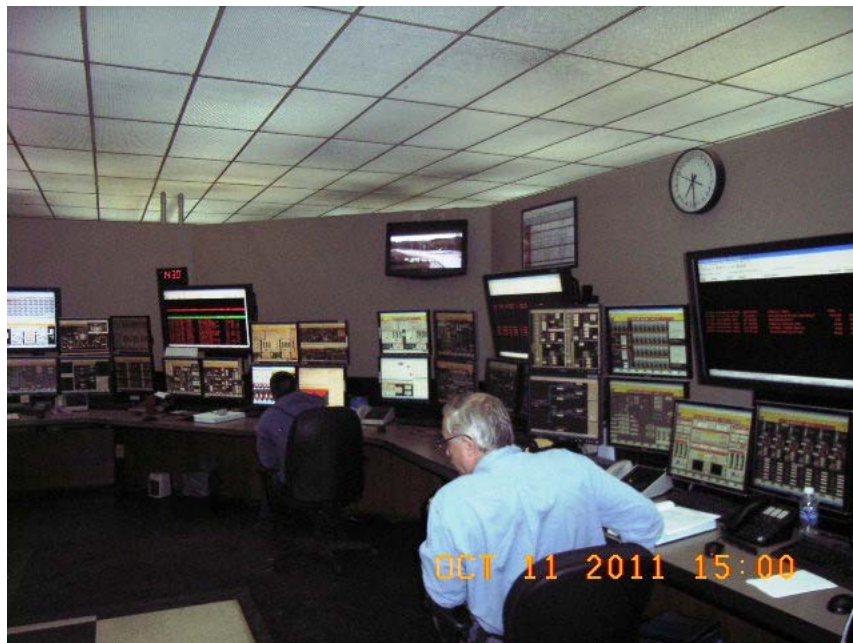
Unit 1 & 2 Controls at Ghent Generating Station
