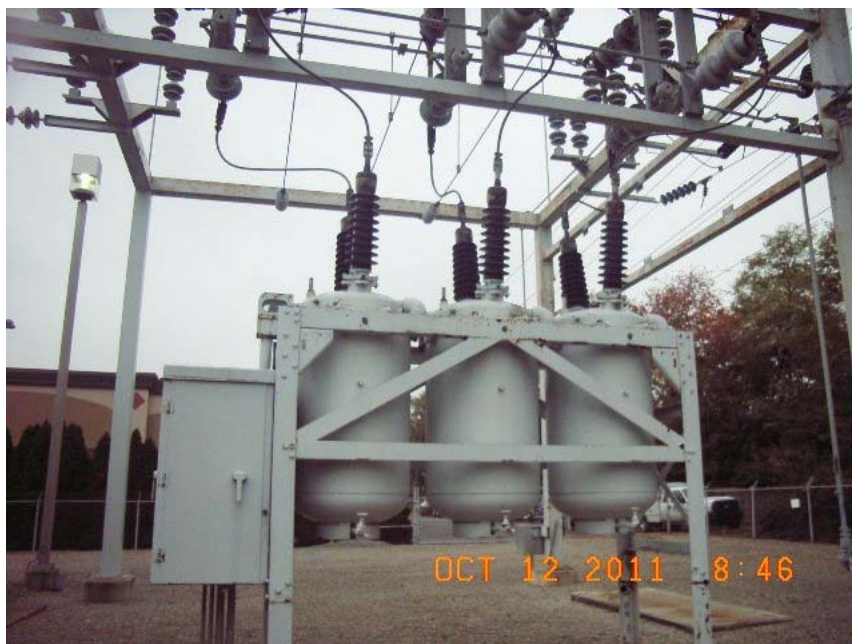
Oil Breakers at Frey's Hill Substation
