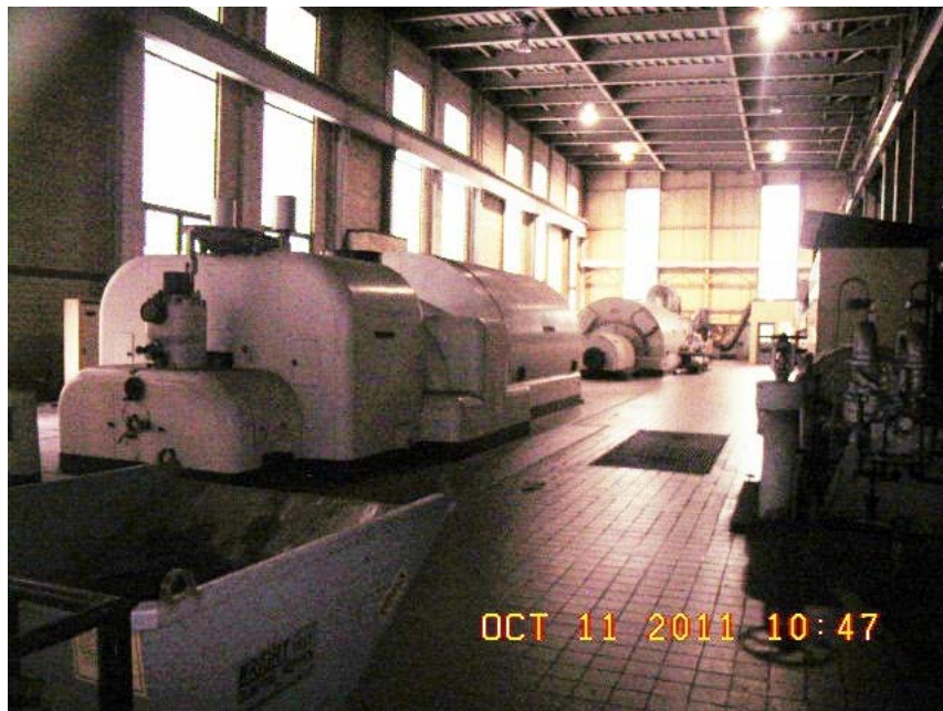
Units 2 and 3 Turbines at Tyrone Generating Station
