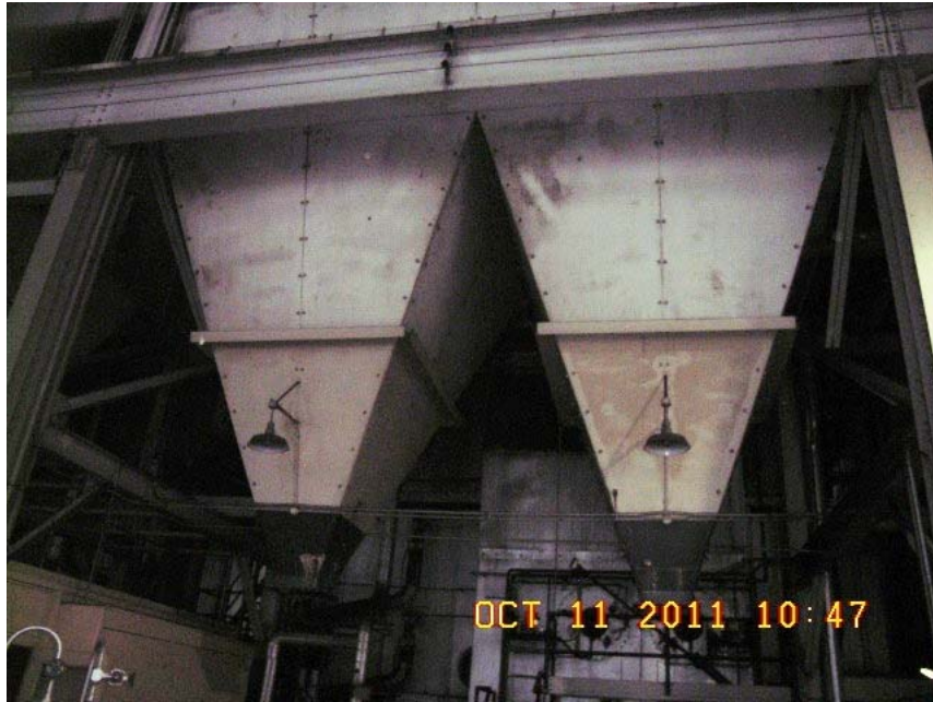
Boiler at Tyrone Generating Station
