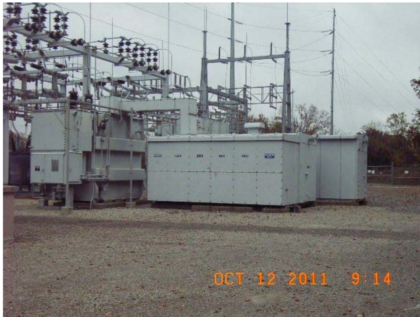
Switchgear and Transformer at Collins Substation
