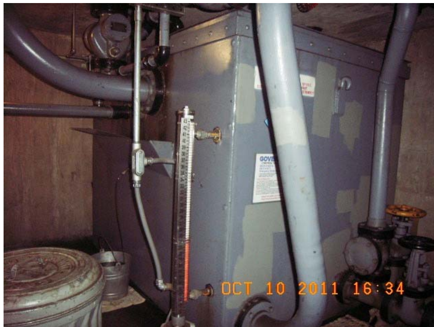
Unit 4 Governor Oil System at Ohio Falls Hydro Plant
