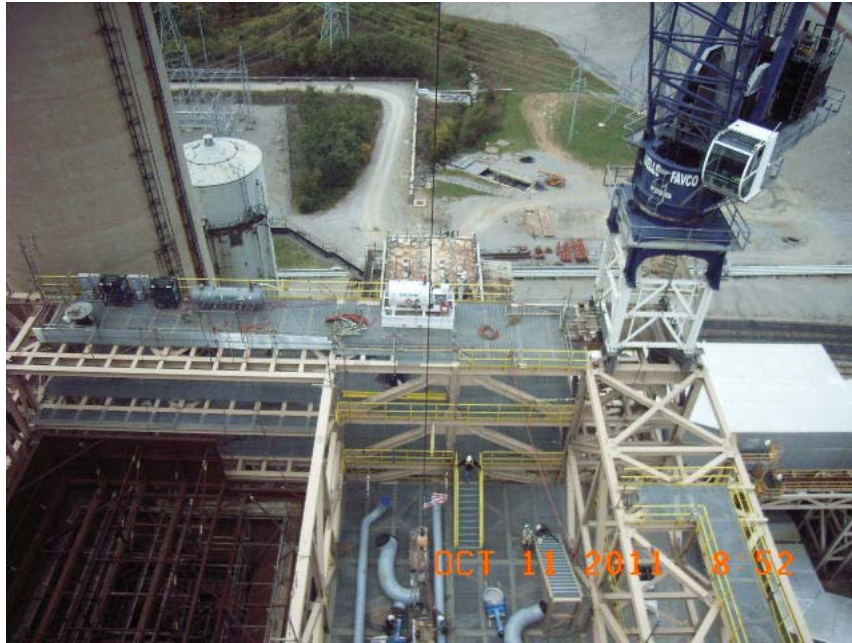
Unit 3 SCR AT Brown Generating Station
