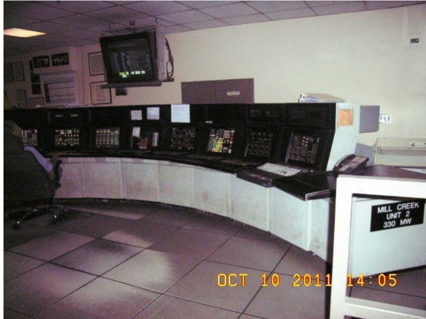
Unit 2 Controls at Mill Creek Generating Station
