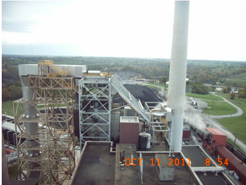
Unit 1 Stack and New Duct Work at Brown Generating Station
