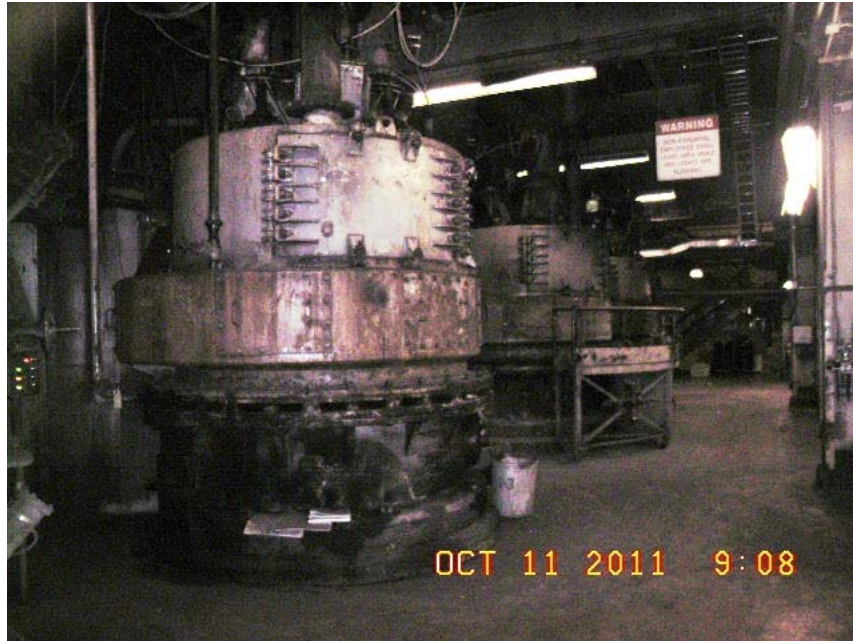
3 of 4 Pulverizers for Unit 1 at Brown Generating Station
