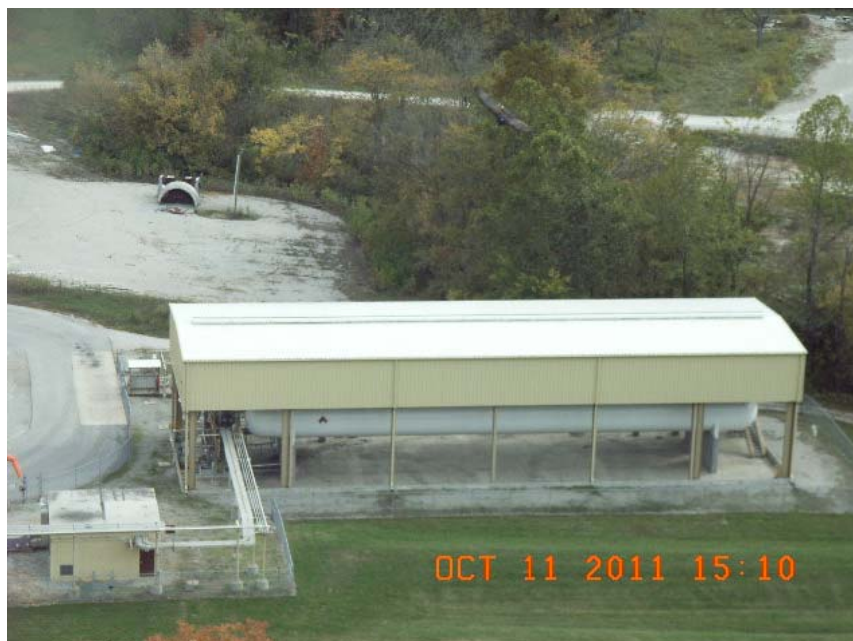
Ammonia Equipment at Ghent Generating Station
