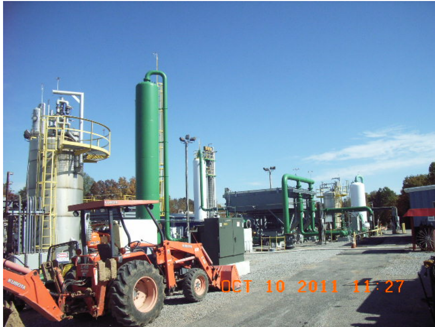
2 of 3 Gas Purification Units at Muldraugh Compressor Station
