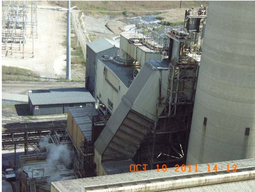
Unit 4 FGD at Mill Creek Generating Station
