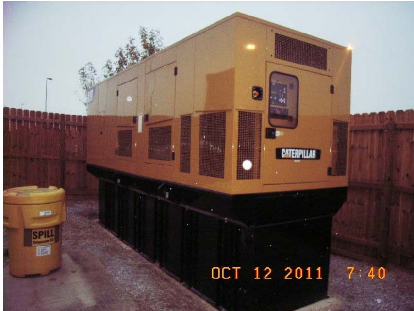
Emergency Generator at East Service Center
