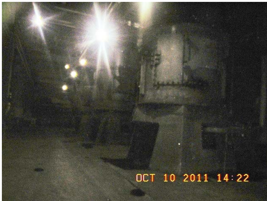
1 of 4 Pulverizers for Unit 3 at Mill Creek Generating Station
