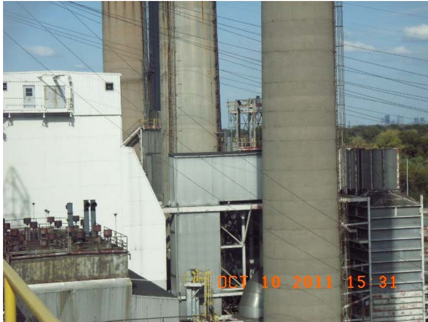
Precipitator and Scrubber at Cane Run Generating Station
