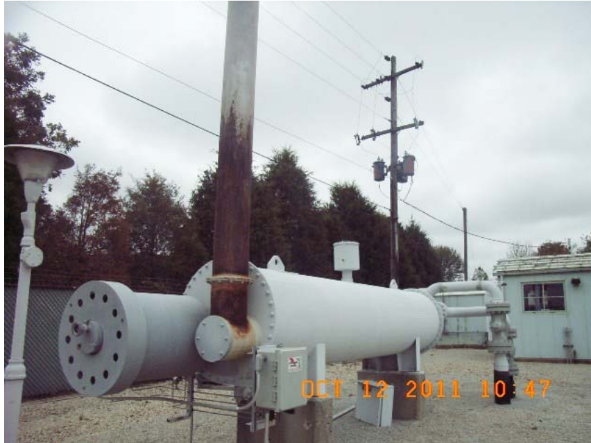
Water Bath Heater at Elder Park City Gate Station
