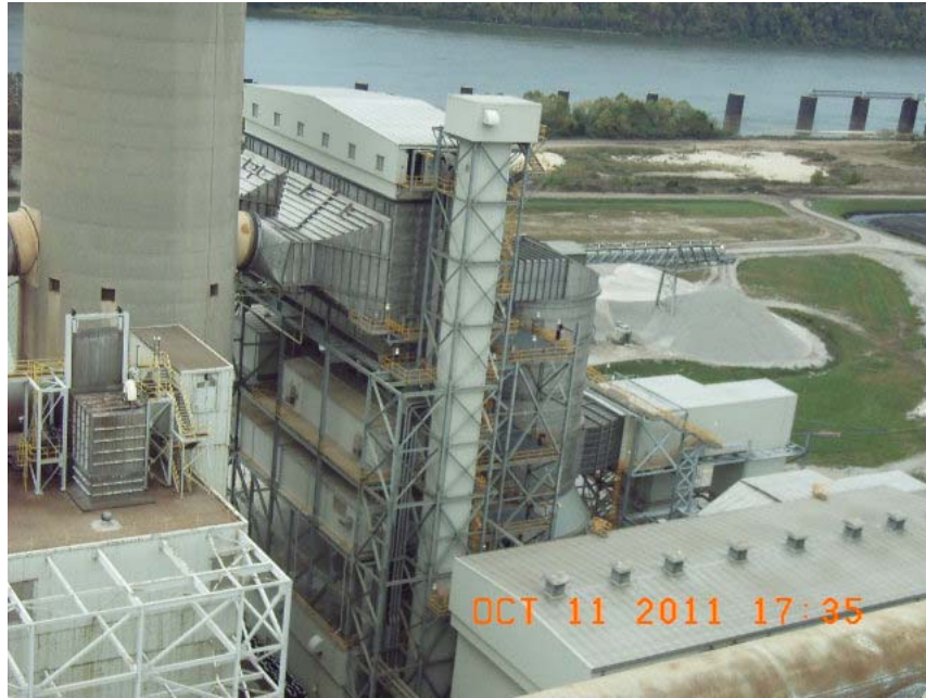
Unit 2 Scrubber at Trimble County Generating Station
