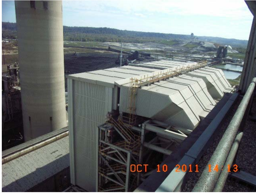
Unit 4 SCR AT Mill Creek Generating Station
