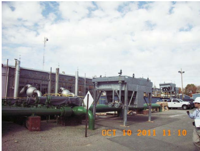
Compressor Building and Cooling Tower at Muldraugh Compressor Station
