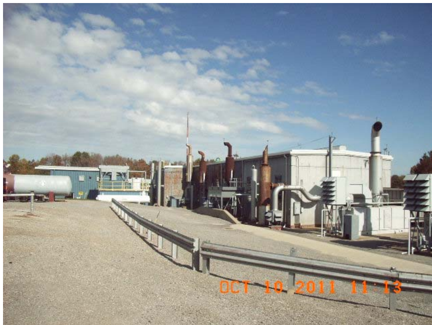
Exhaust for Compressors at Muldraugh Compressor Station
