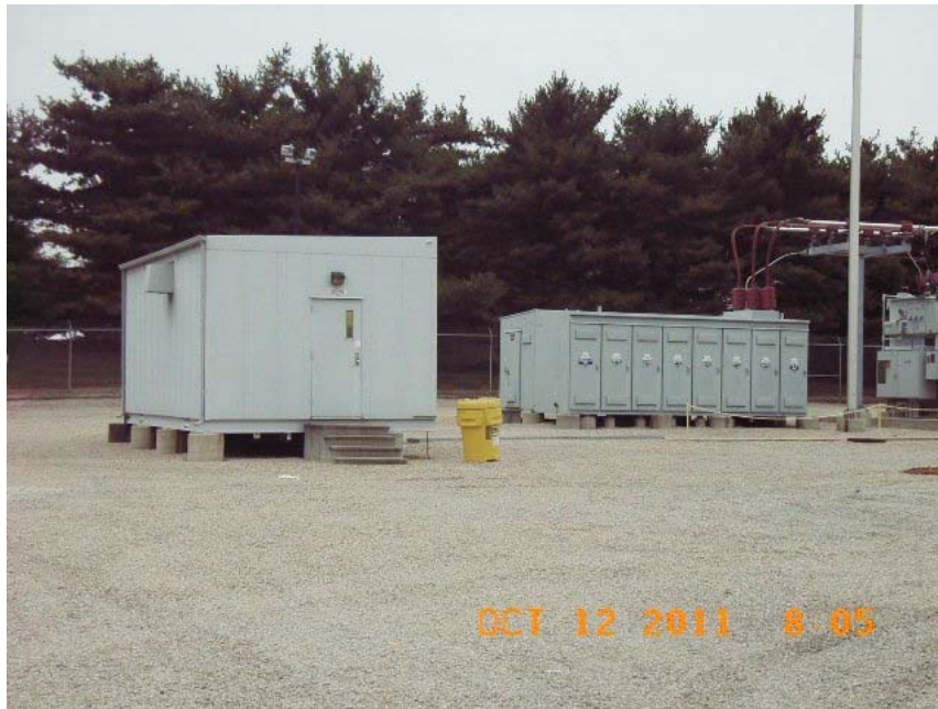
Control Building and Switchgear at Worthington Substation
