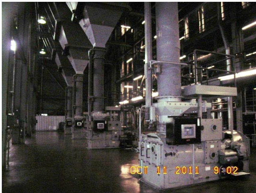
Unit 3 Coal Feeders at Brown Generating Station
