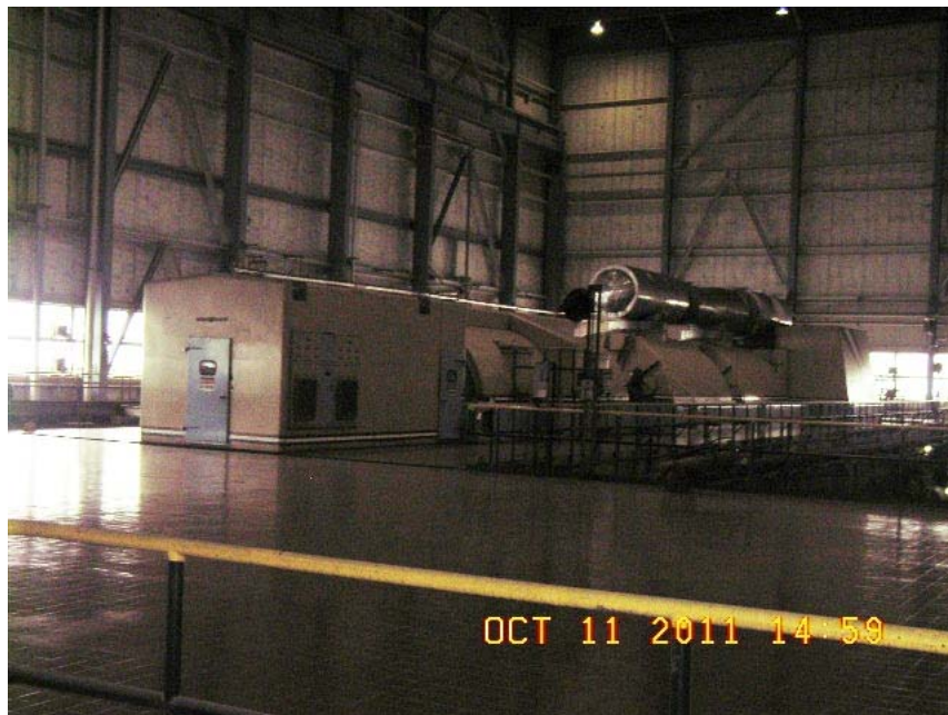
Unit 2 Turbine at Ghent Generating Station
