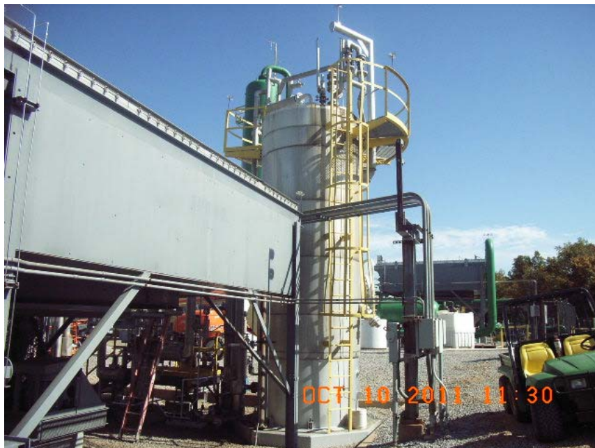
Carbon Filter at Muldraugh Compressor Station
