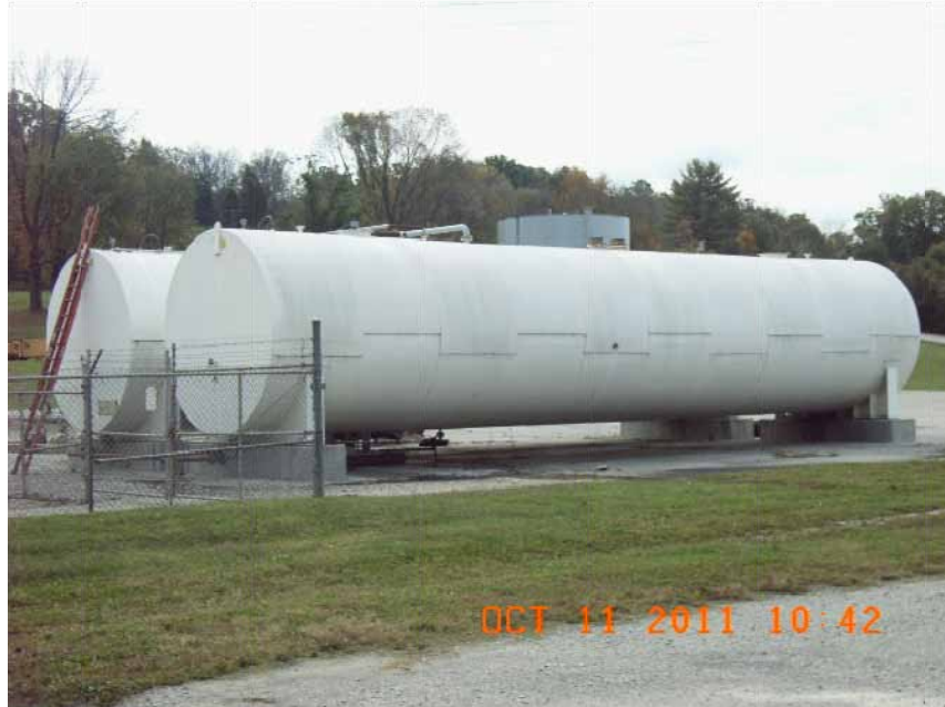
Fuel Tanks at Tyrone Generating Station
