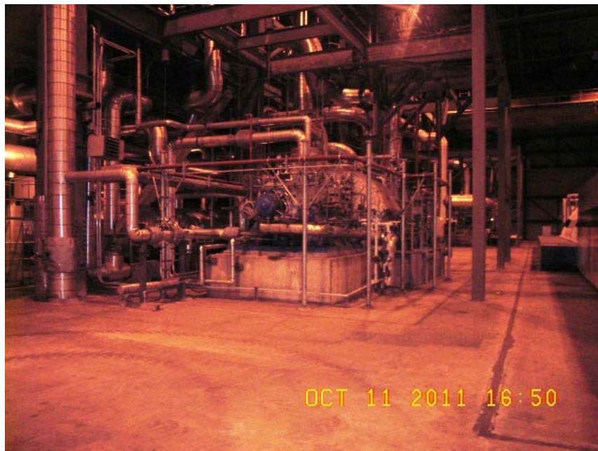
Steam Driven Boiler Feed Pump for Unit 2 at Trimble County Generating Station
