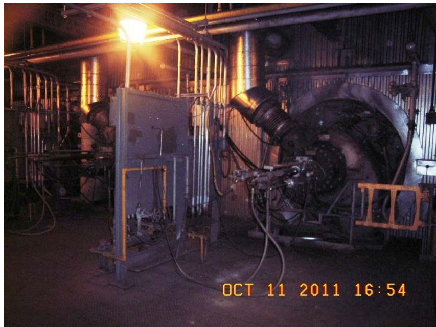
1 of 5 Burners for Unit 2 at Trimble County Generating Station
