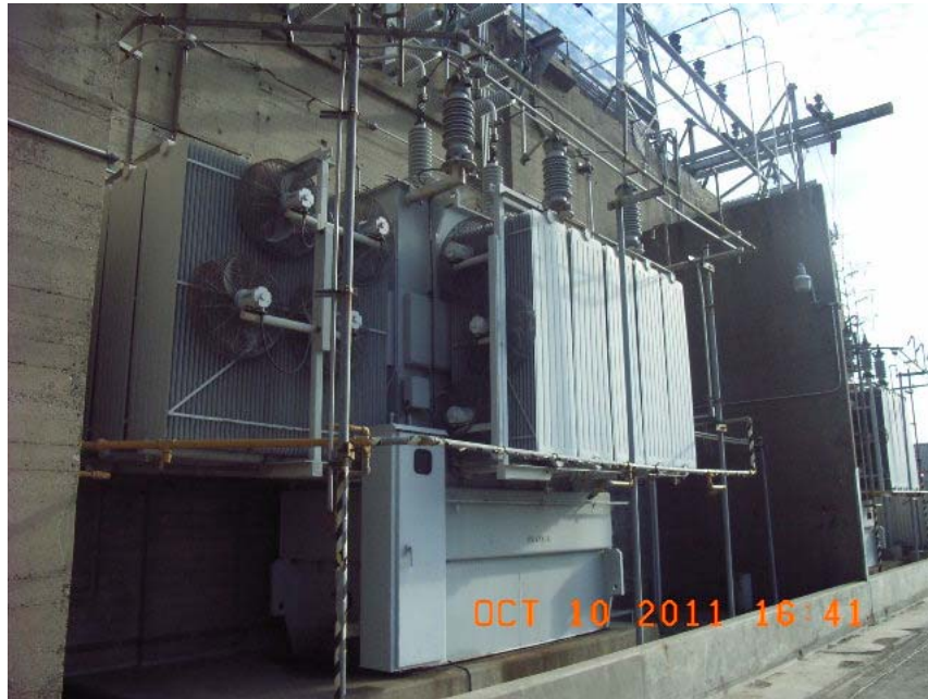
Transformer at Oho Falls Hydro Plant
