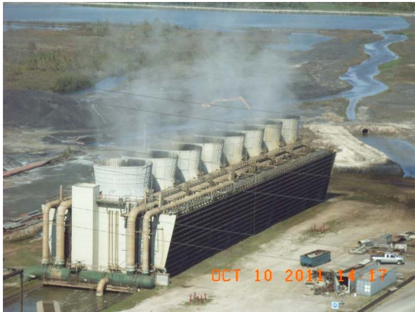
Unit 2 Cooling Tower at Mill Creek Generating Station
