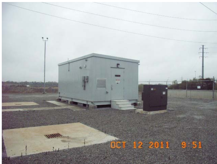
Control Building at Old Henry Substation
