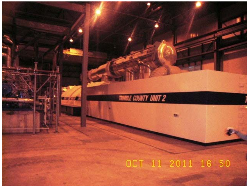
Unit 2 Turbine at Trimble County Generating Station
