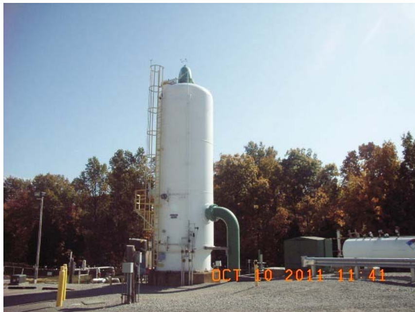
Dehydrator/Absorber at Muldraugh Compressor Station
