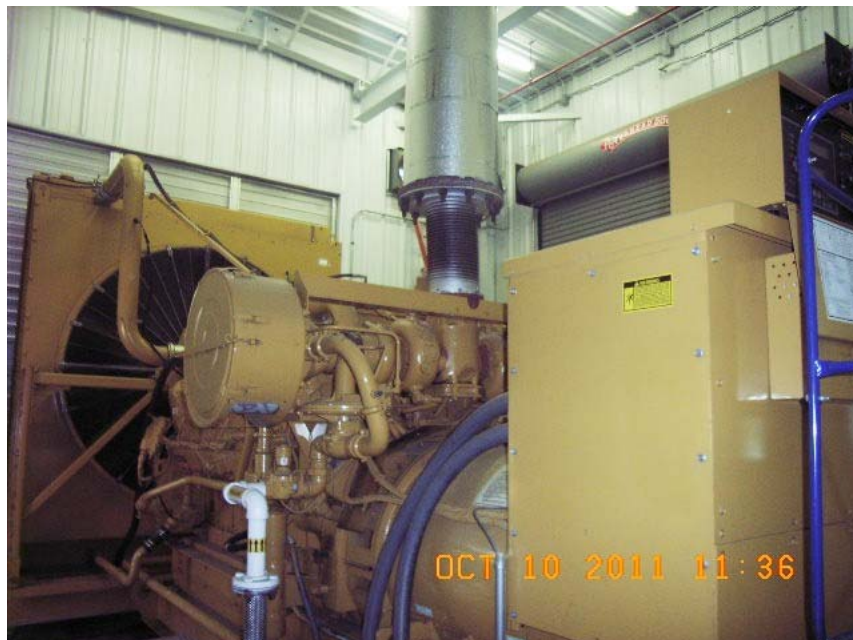
Emergency Generator (1996) at Muldraugh Compressor Station
