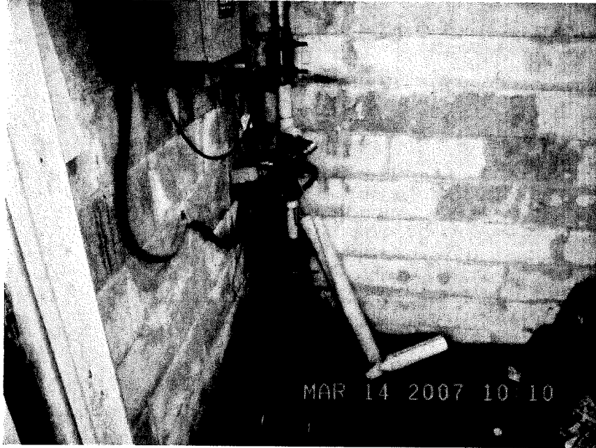
Chlorine Equipment at Chlorine Loading Station
