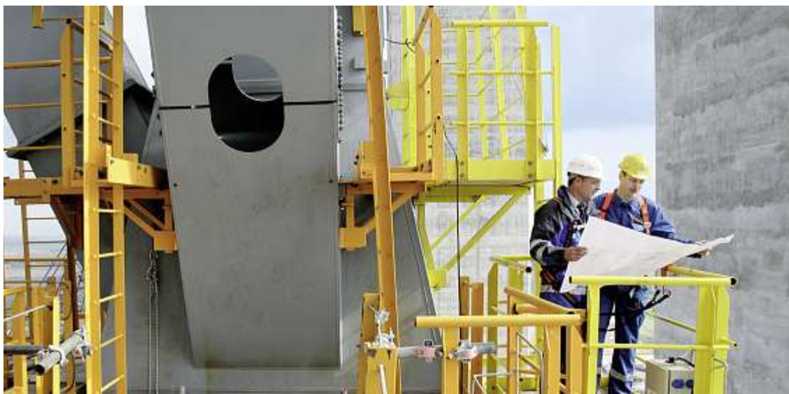
The future F unit of the new lignite-fired power plant, Neurath, Germany: on-site inspection on the boiler frame
