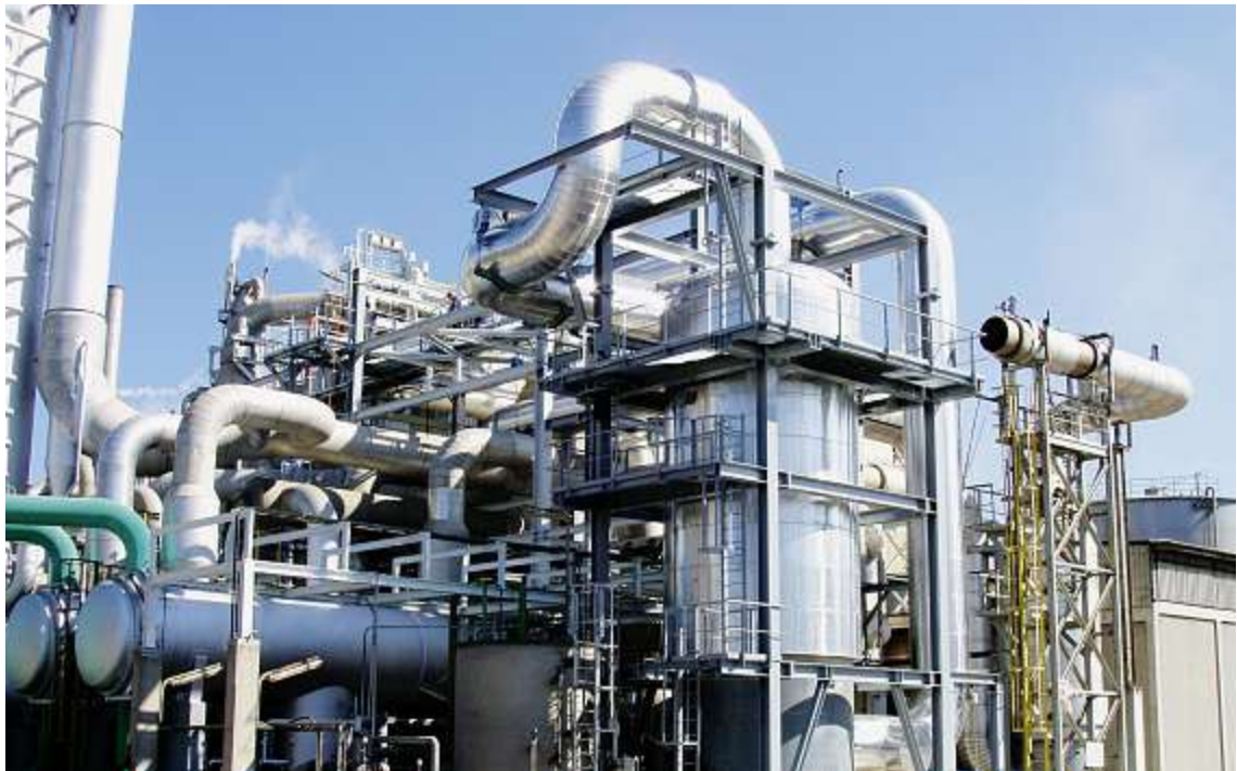
Abu Qir, Egypt: EnviNOx ® catalytic converter for the disposal of laughing gas (N 2 O) in a fertilizer production facility
