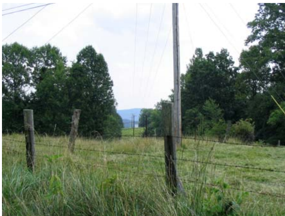
Photograph 9 - Point Near KOP DD, Jackson Energy Electric Transmission Line Photograph taken by Brighton A & E Inc. Dated June 29, 2004.
