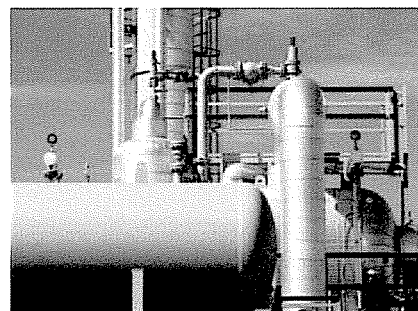
The Platteville facility is one of DEFS' newest gathering and processing plants, built to process increased natural gas production in the Denver-Julesburg Basin area of Colorado.
