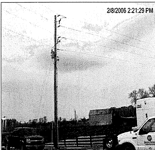
POLE SHOWING THE TAP LINE FUSE AND THE TRANSFORMER FUSE
