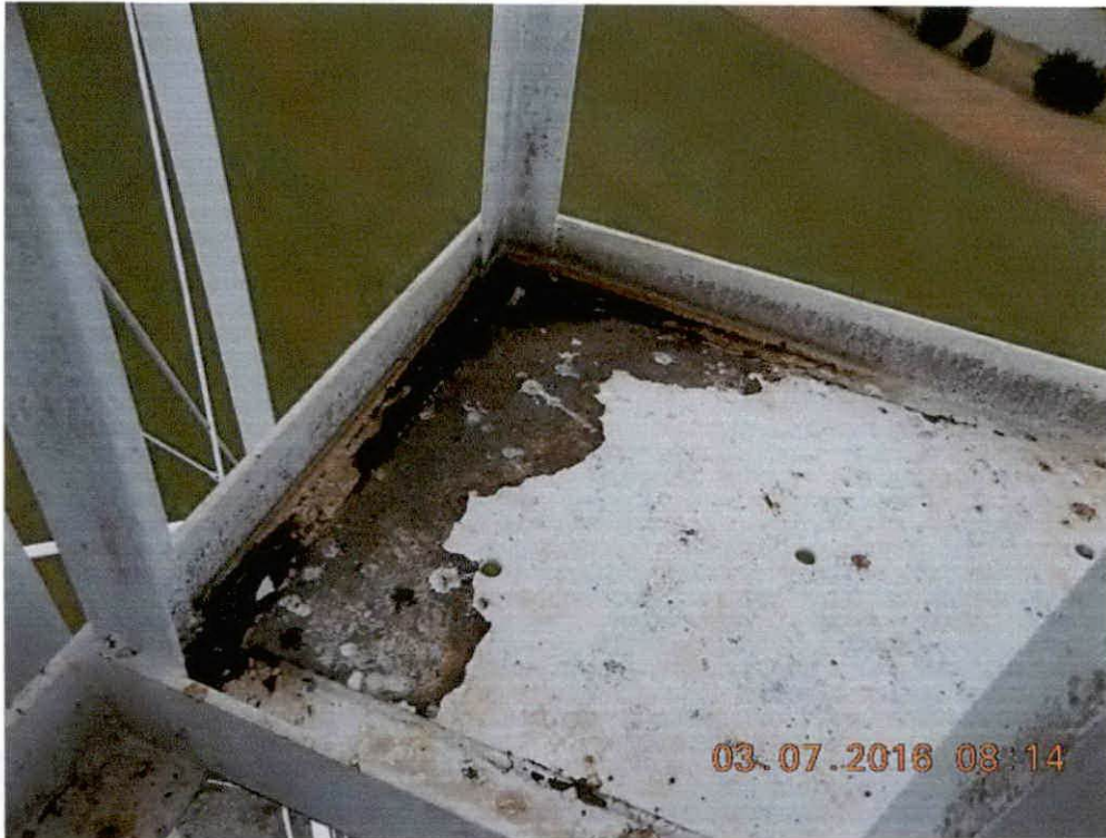
Failed coating ladder platforms
