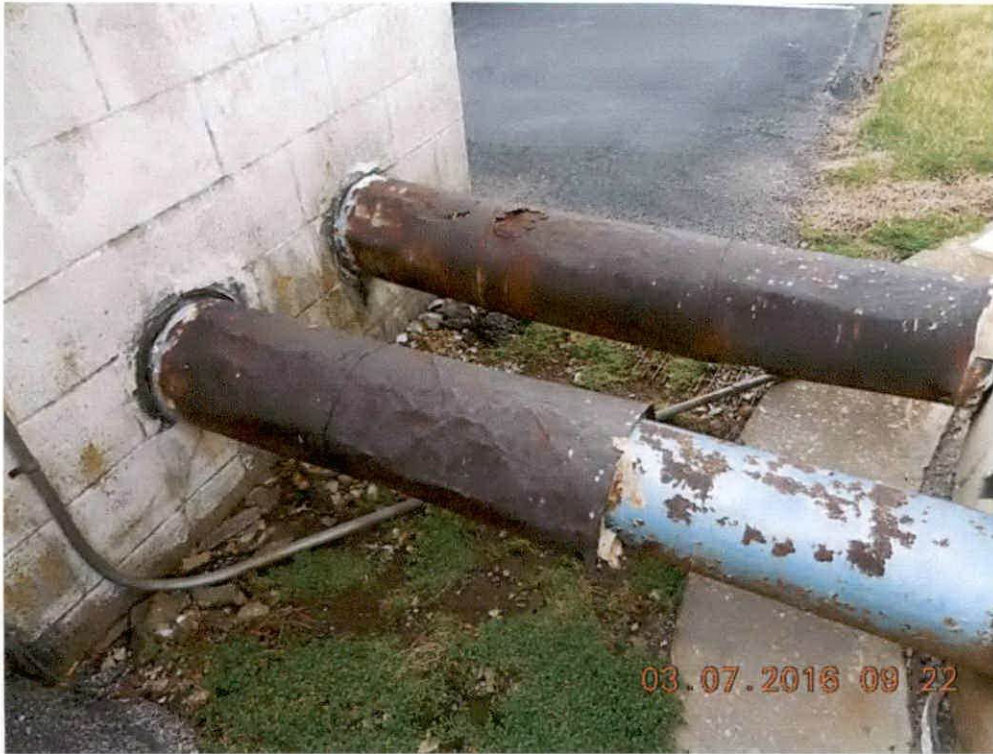
Inlet /outlet piping to valve house, most insulation damaged or missing
