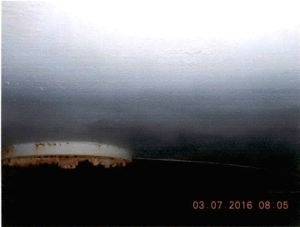
Failed coating interior roof vent
