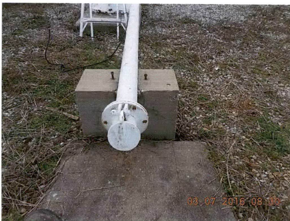
Overflow flap valve, not secured in place
