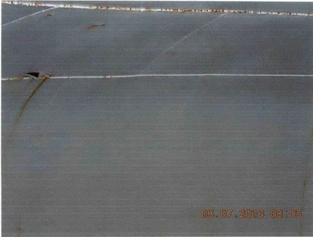
Rusing and failed coating interior roof
