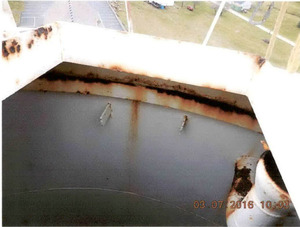
Roof manway, compression ring heavily rusted. Old ladder supports not removed, when ladder was removed. Overflow piping heavily rusted
