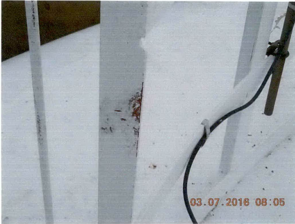
Failed coating roof corral
