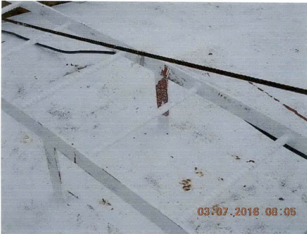
Failed coating roof and ladder
