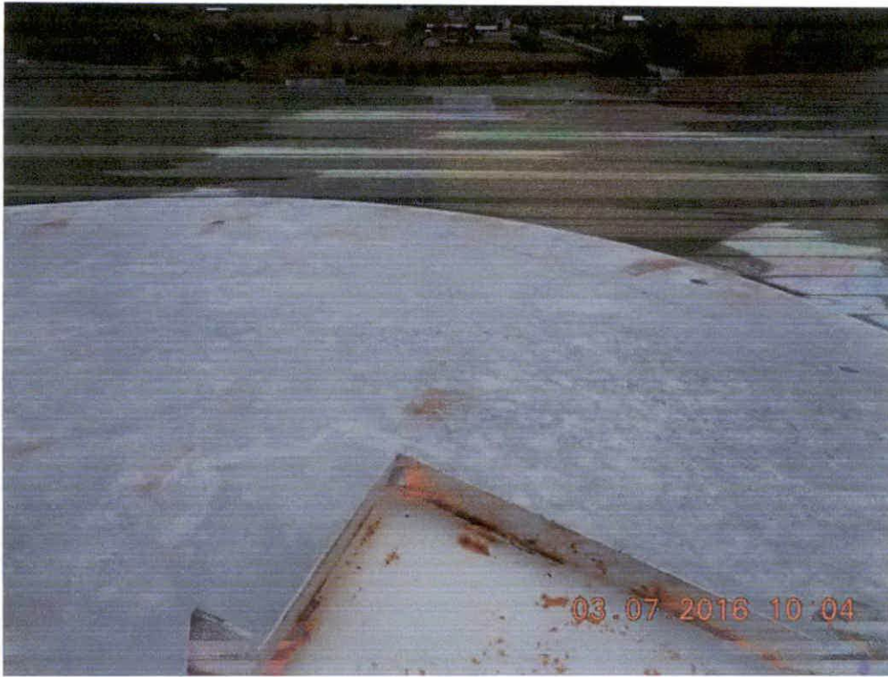
Failed coatings roof
