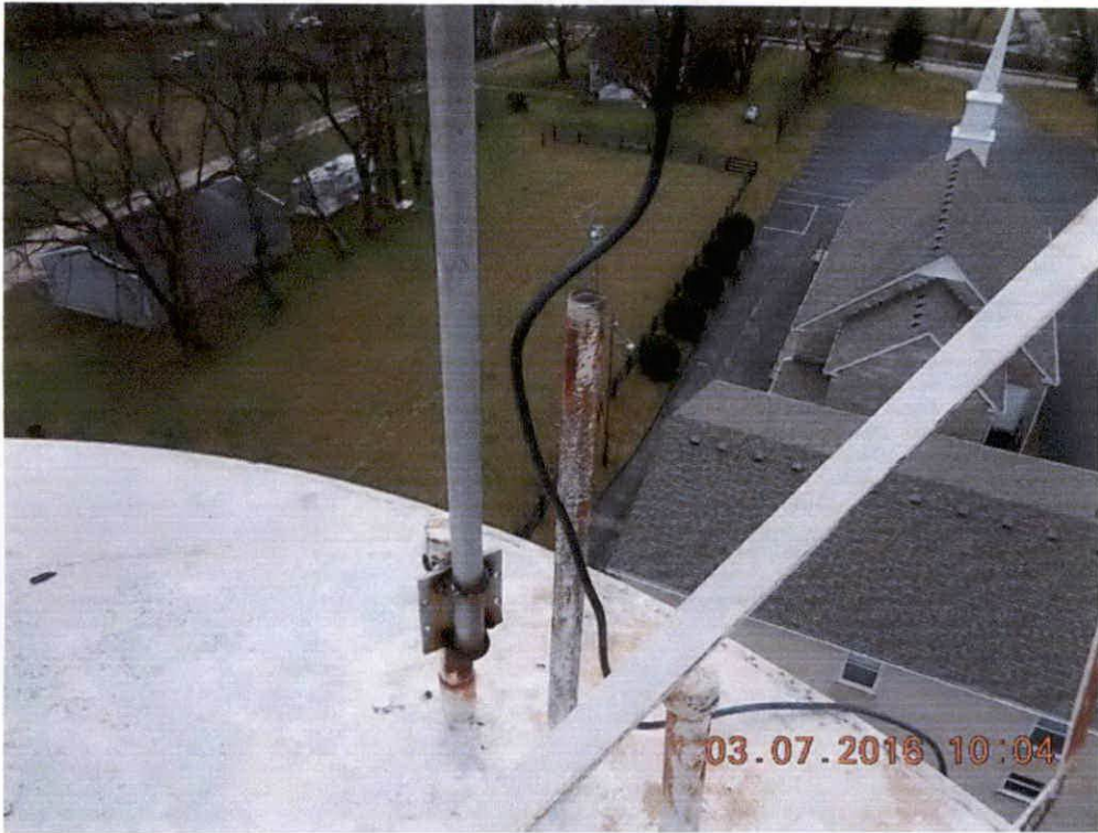
Unsecured comm cable
