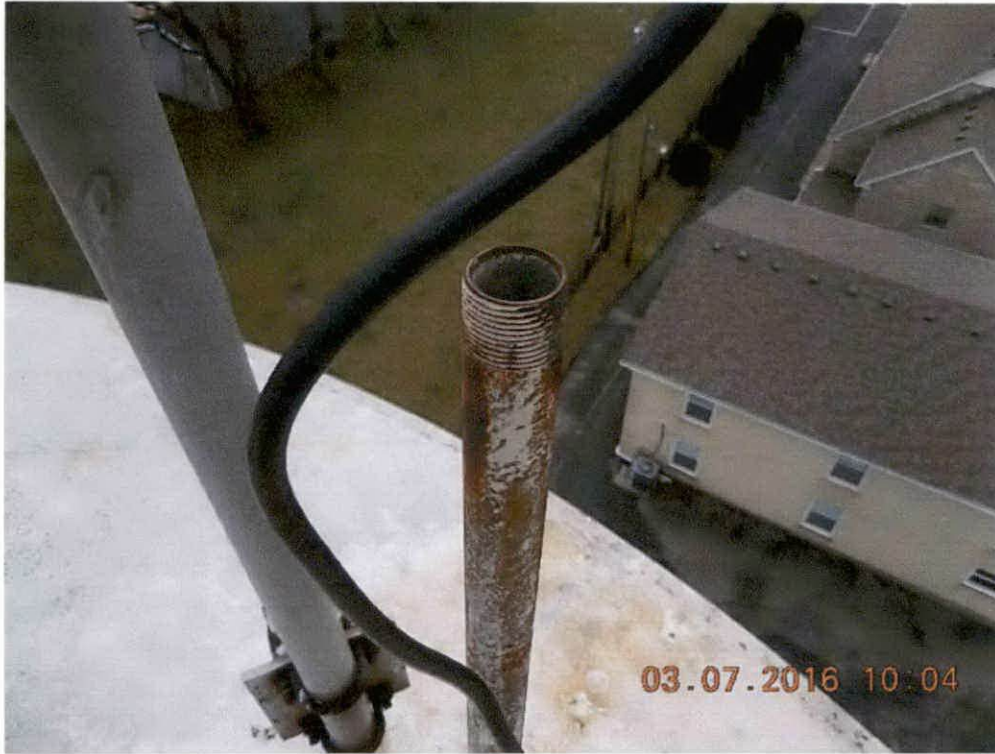
Comm antenna mast and wire not secured
