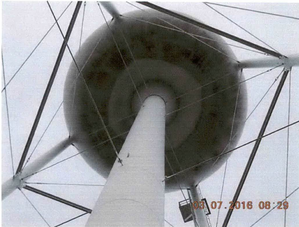
Belly of tank mildew
