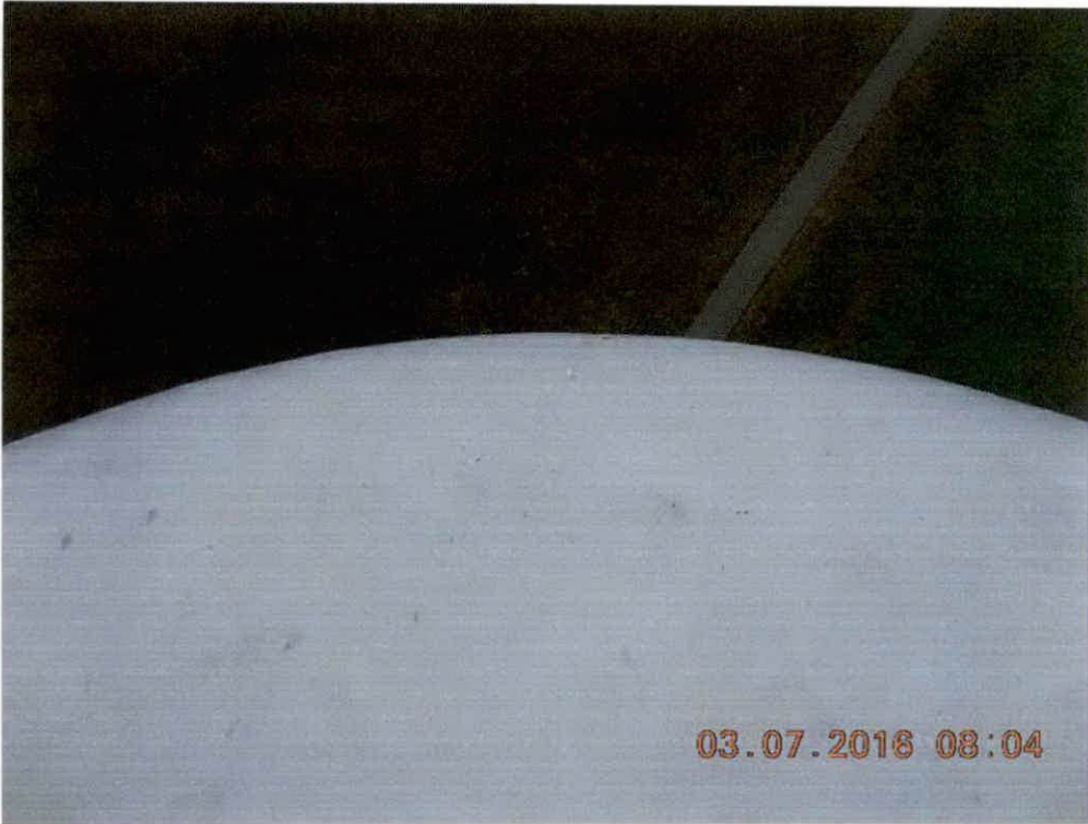
Roof coating thinning
