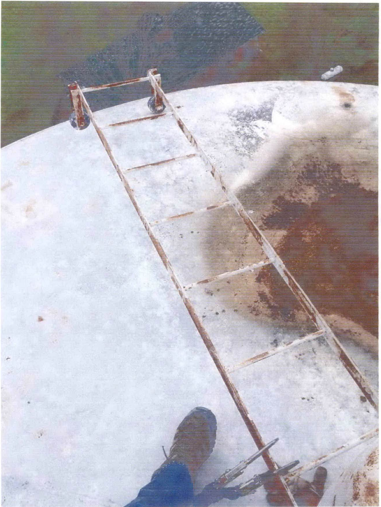
Ponding water on roof(where imploded), roof ladder(not secured, no
