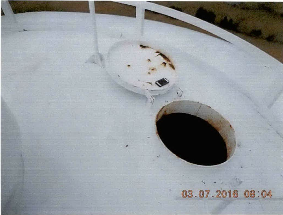
Roof manway failed coating
