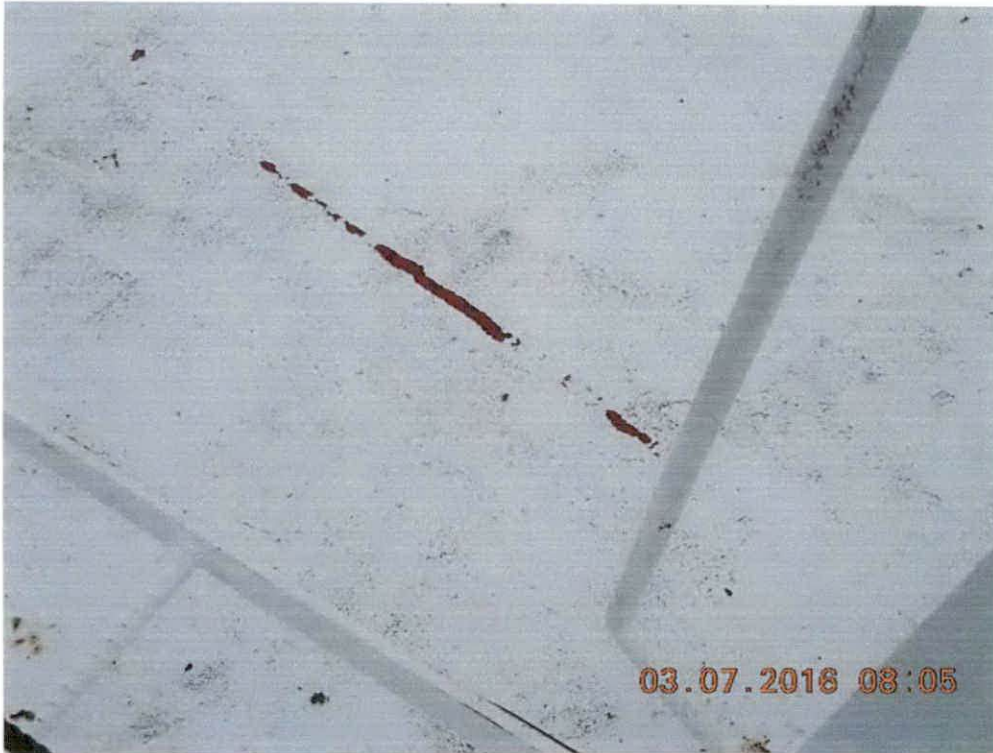
Failed coating roof
