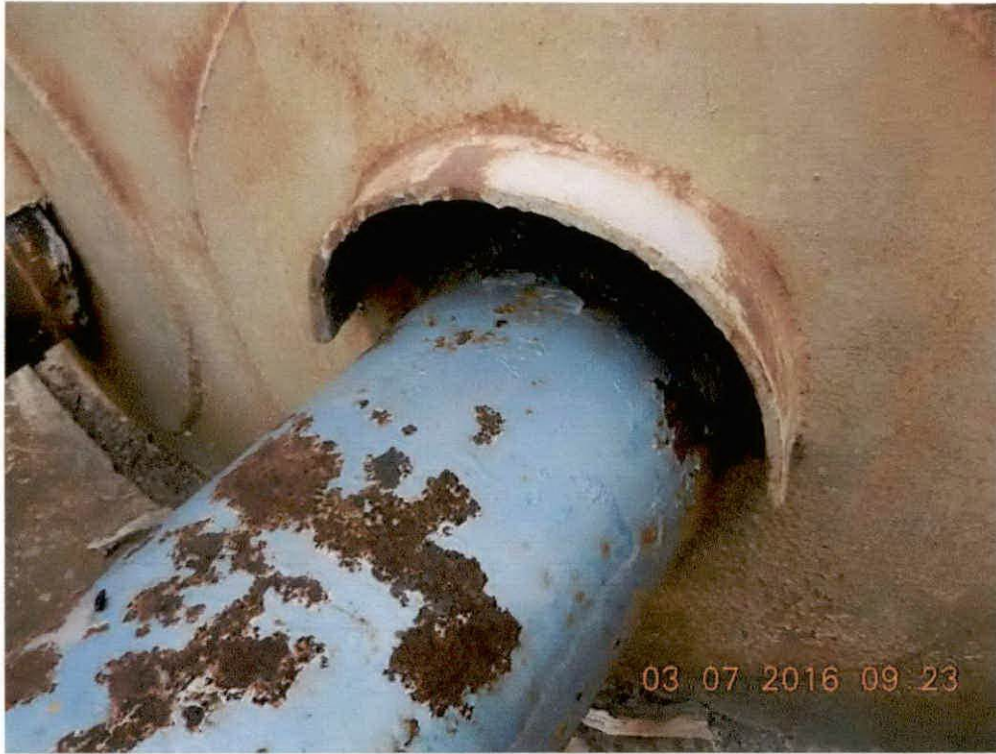
Inlet pipe no insulation
