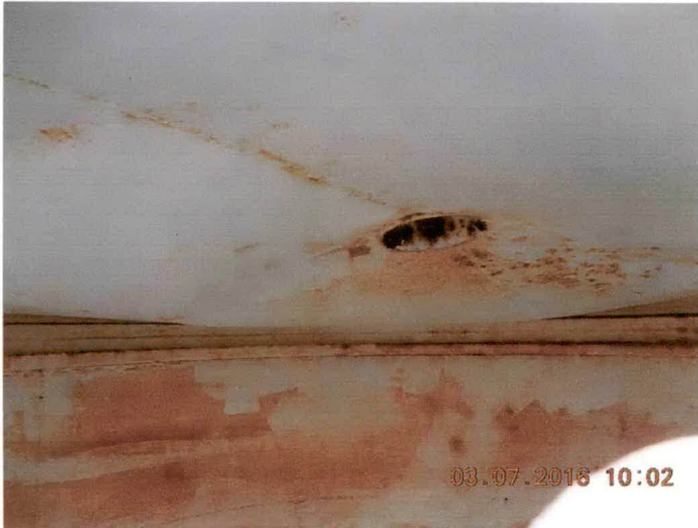
Interior roof and vent failed coatings, compression ring rusted heavily. Note that roof has a bow inward. This is from the imploded roof(see comments in report, about roof)
