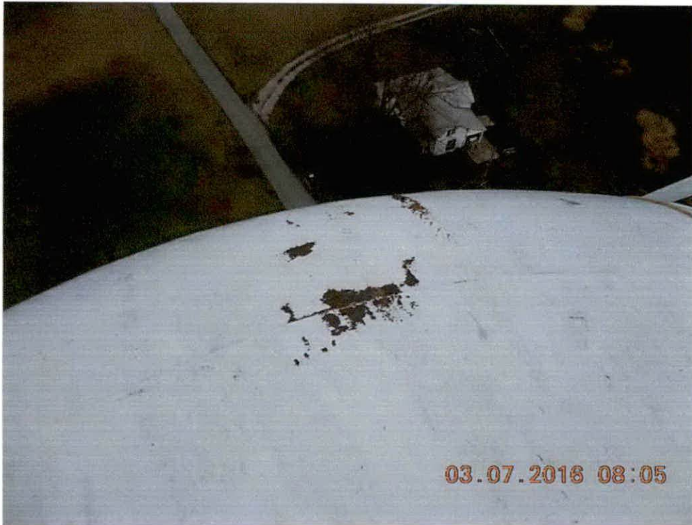
Failed coating roof
