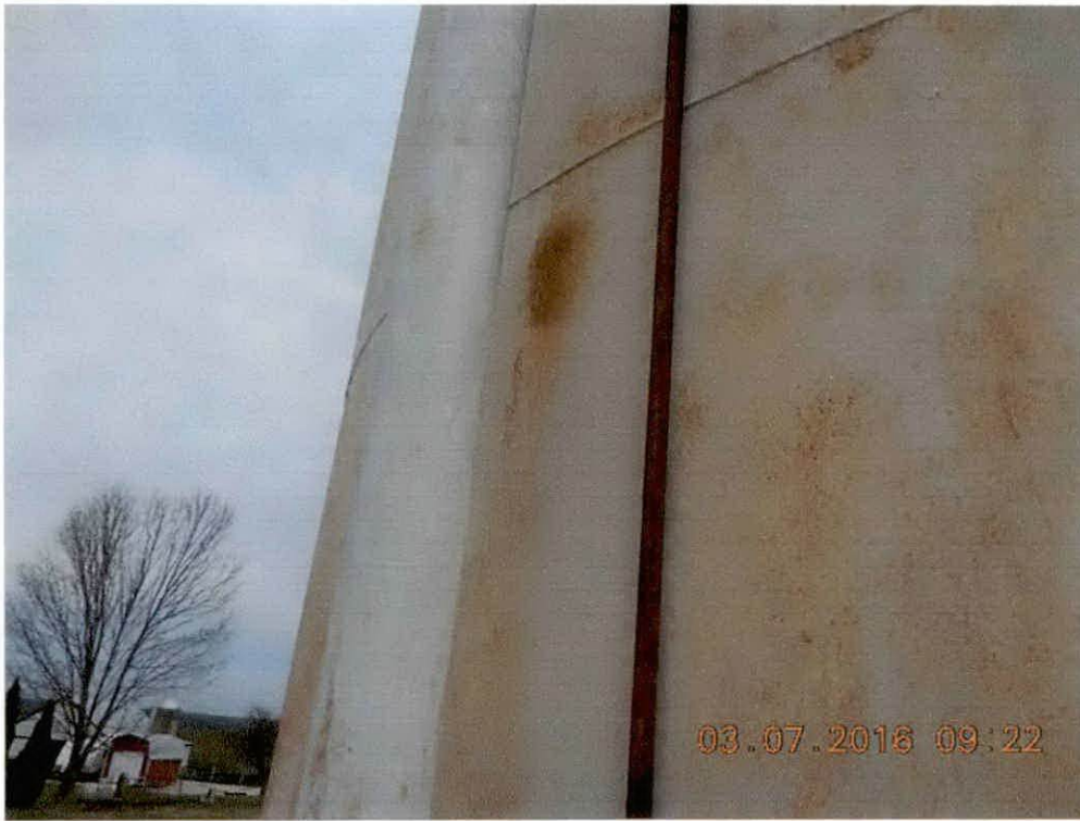
Failed coating tank exterior
