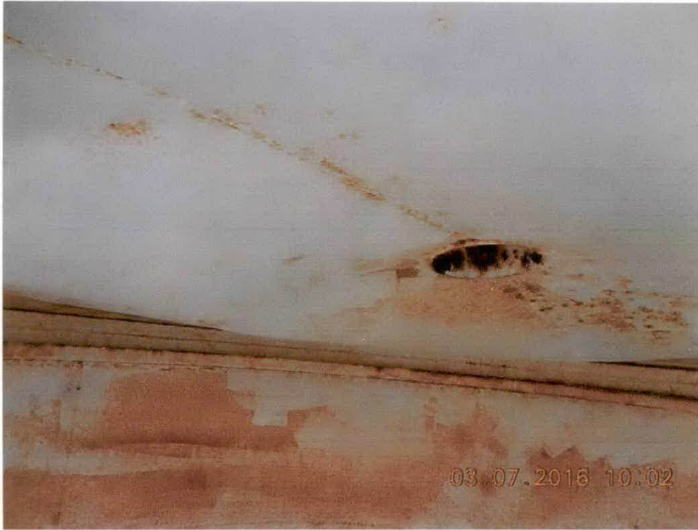
Roof vent interior heavily rusted
