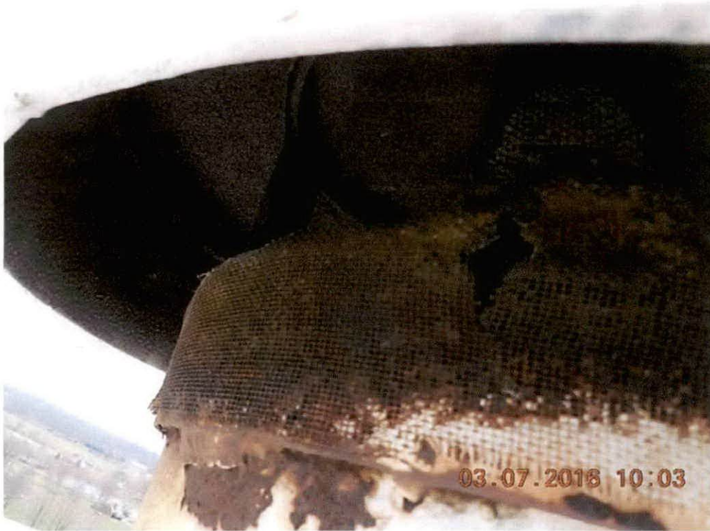
Roof vent with fine mesh screen. This screen is most likely the cause of the roof collapse/implosion. Most likely the screen frosted over during a cold period.
