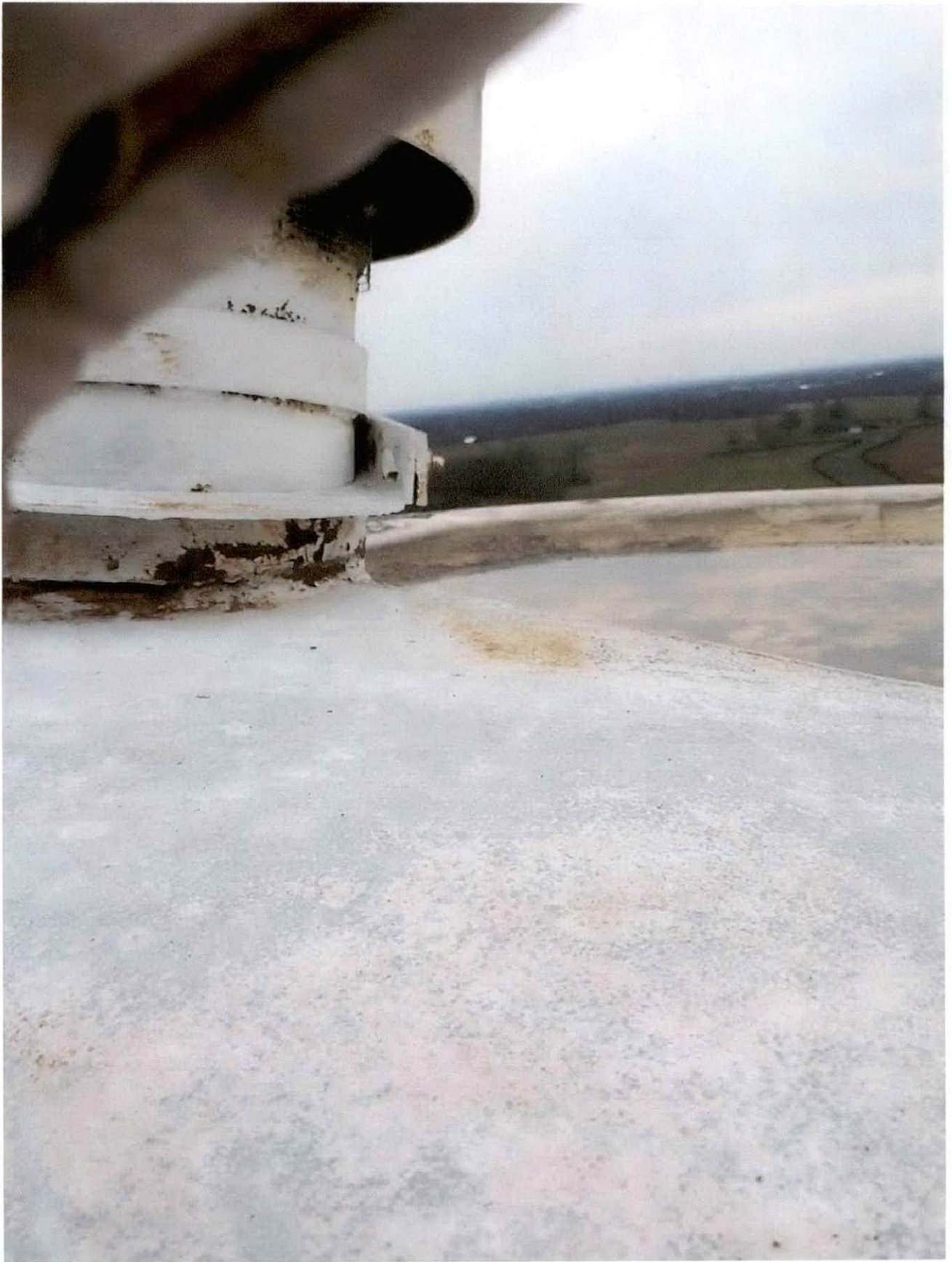
Another view of vent and roof with ponding water
