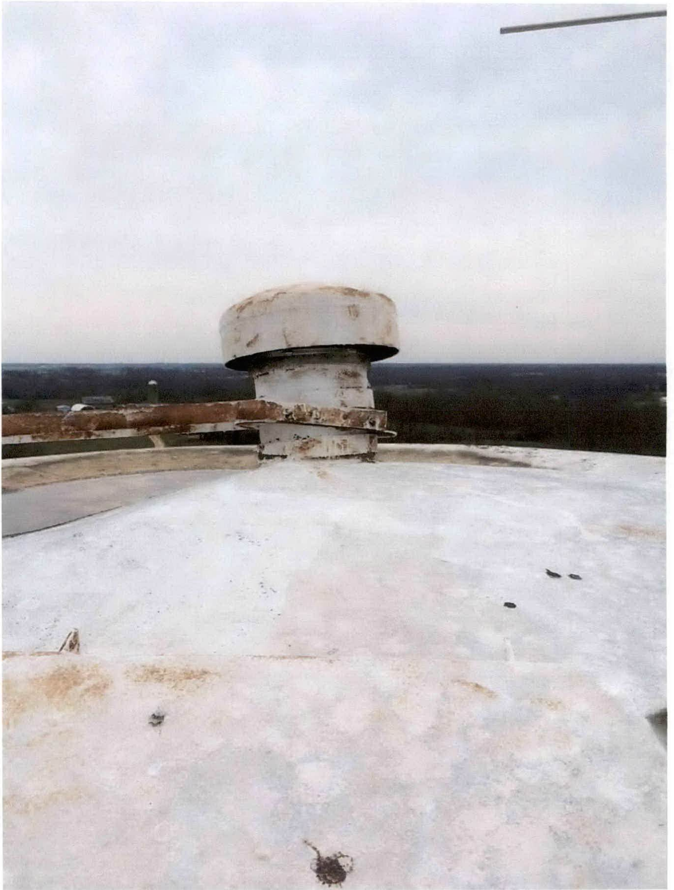
Roof vent and imploded roof. Note vent is no longer straight
