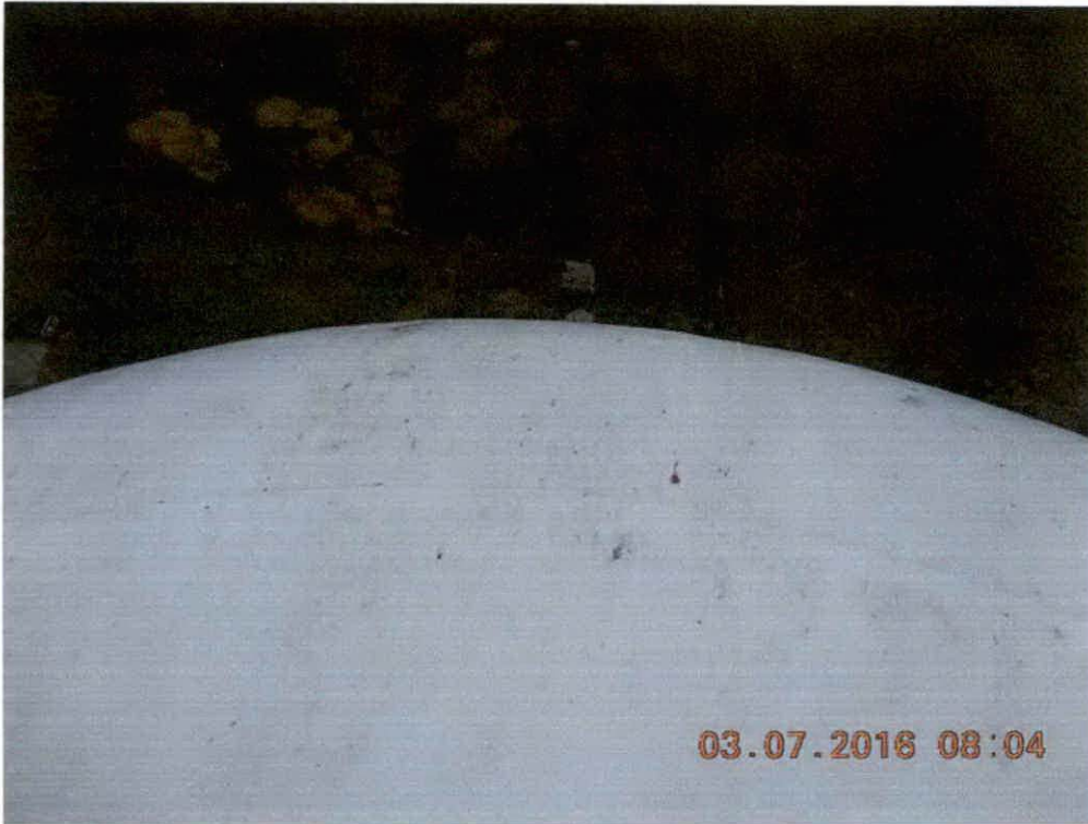
Roof coating thinning
