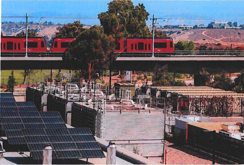
Solar panels and energy storage containers with lithium ion batteries on the campus of the University of California–San Diego on Sept. 16, 2022. (SANDY HUFFAKER/AFP via Getty Images)
