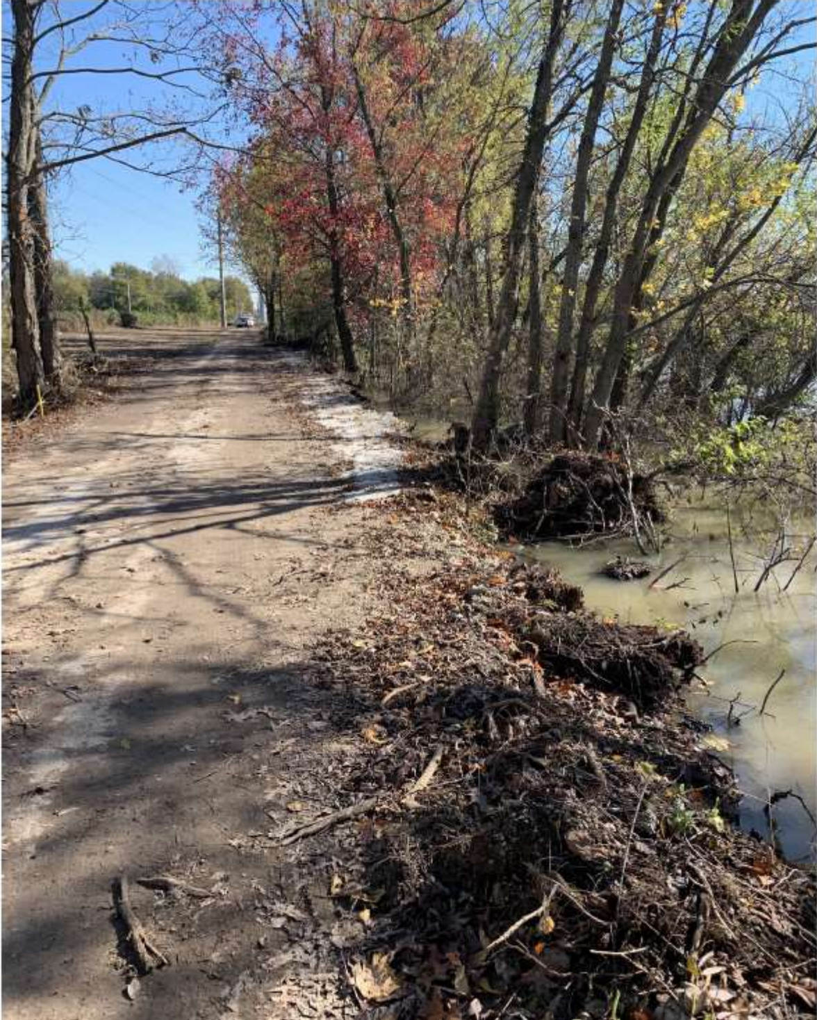
Area behind location of damage.
