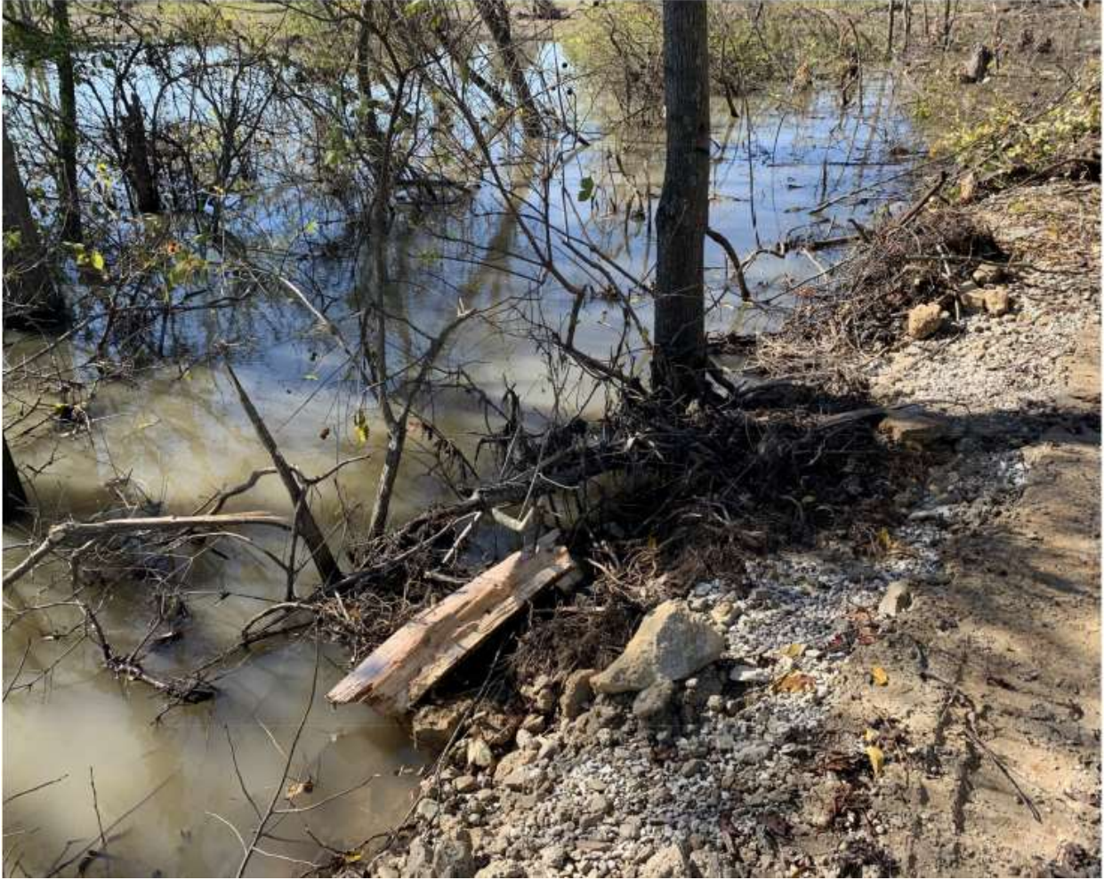
Approximate location of the damage.
