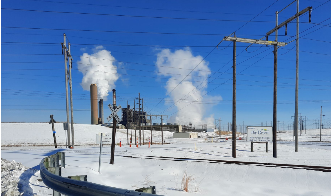
Figure 7. Terminus at Big Rivers Electric Corporation's Reid Substation
