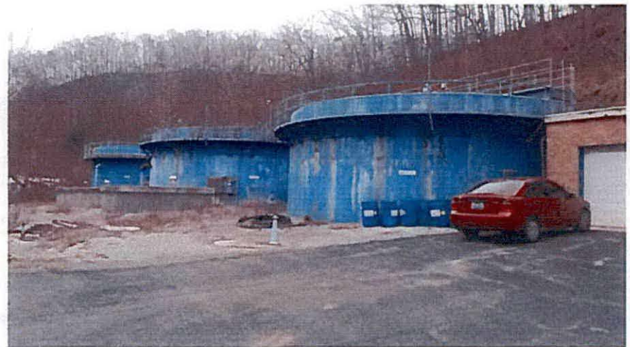
Clarifiers at Water Treatment Plant
