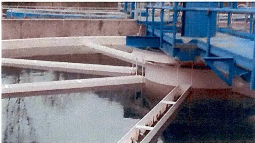
Clarifier #2 at Water Treatment Plant
