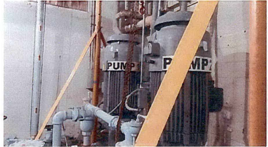
Water Plant Pumps
