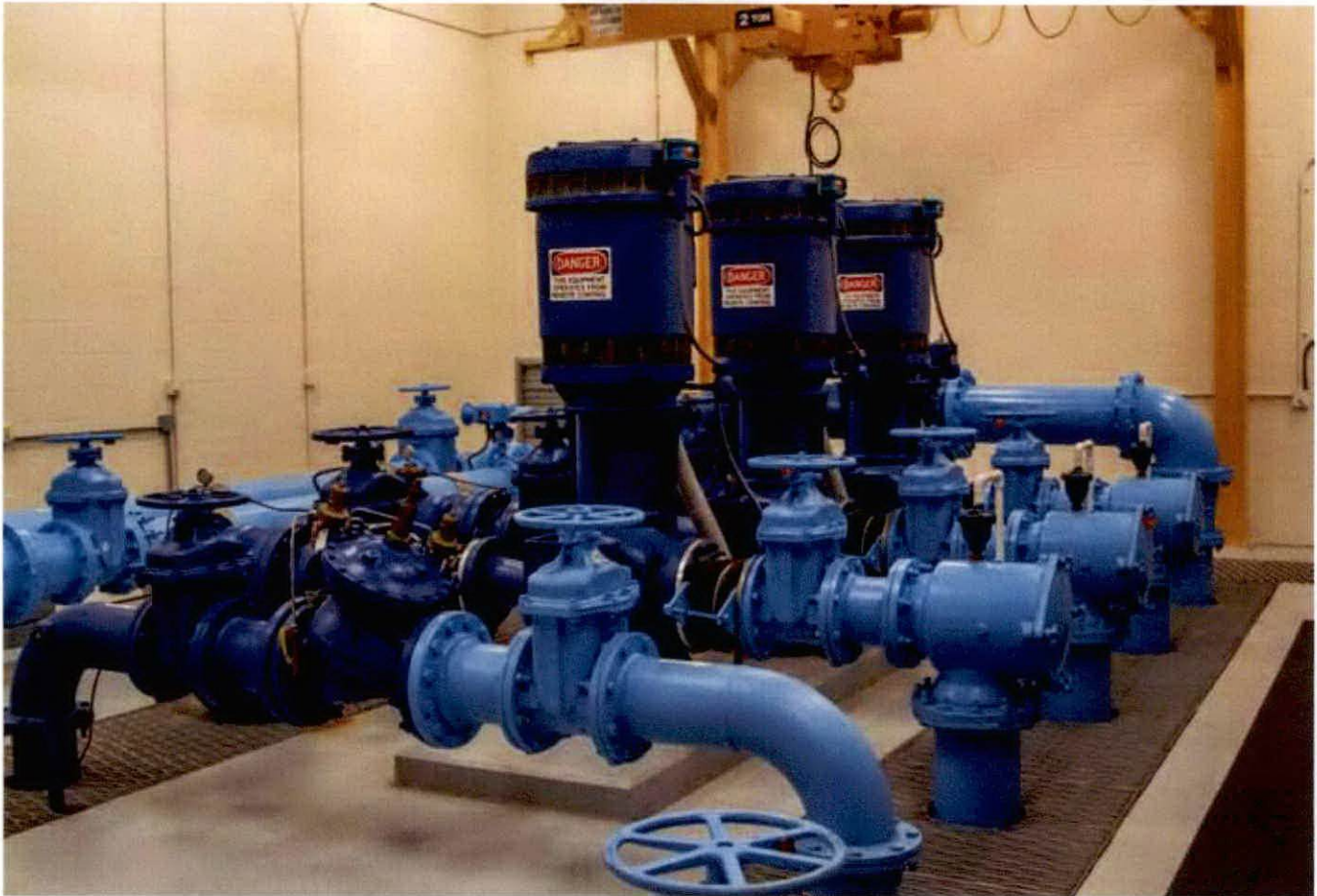
Several times, the Prichard Pump Station at Fort Knox, Ky., has been a lifeline to keep water flowing to customers of Hardin County (Ky.) Water District No. 1. Throughout the years, the district has expanded and diversified its water supply options to ensure flow to customers. Michael D. Moseley
