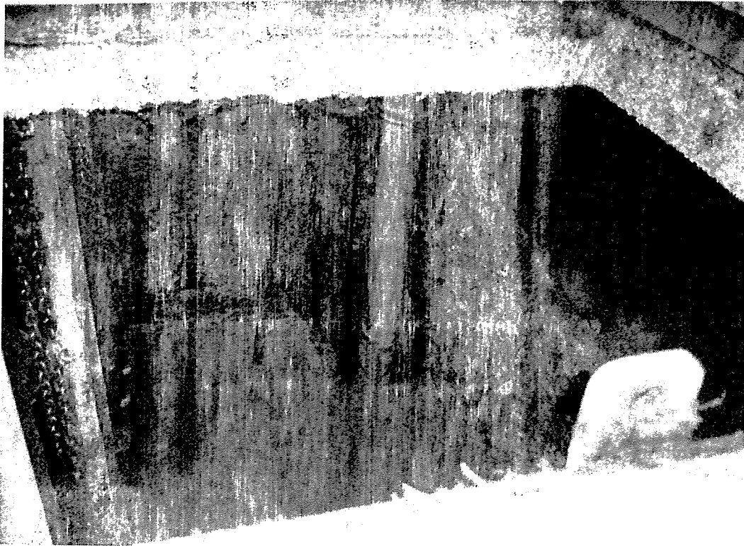
Wet Well – Signs of severe concrete deterioration
