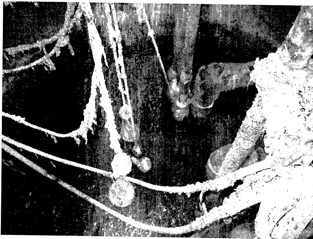
Discharge piping with trash and floatables attached to the cables
