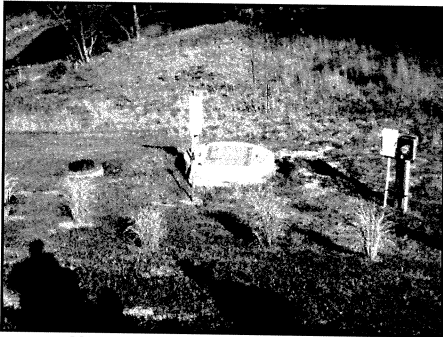
MALLARD POINT DRIVE PUMP STATION
