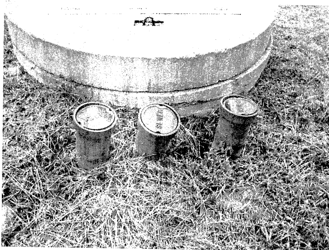
Discharge piping isolation valves
