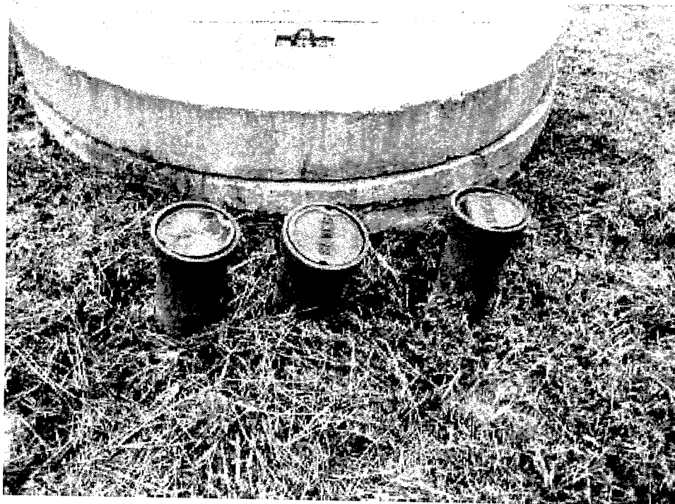
Discharge piping isolation valves
