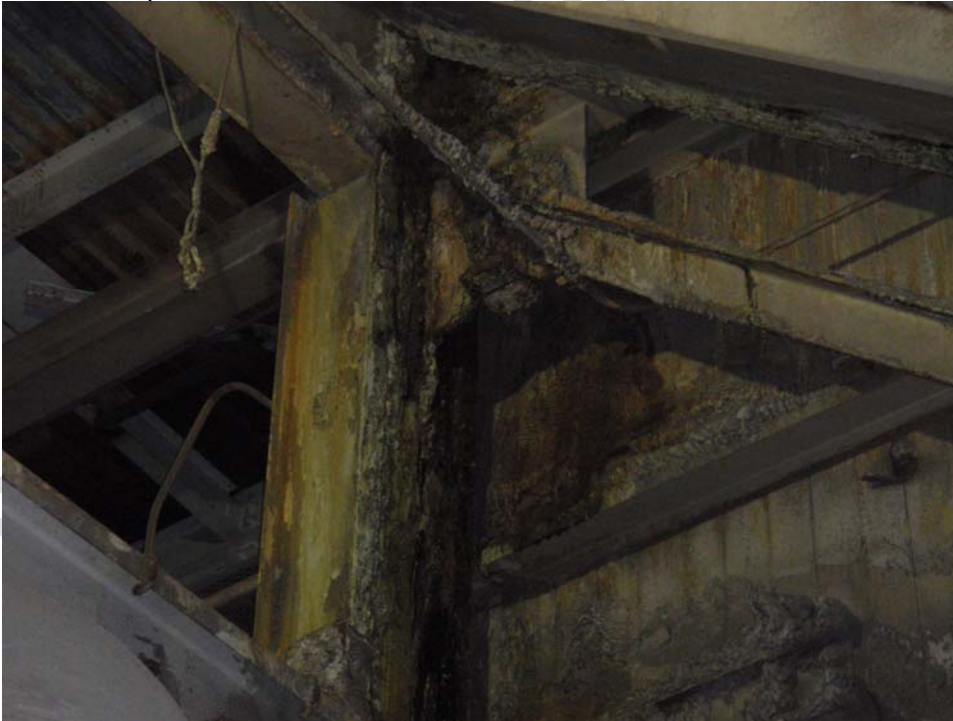
Unit 4 Inside Building are leaking duct.
