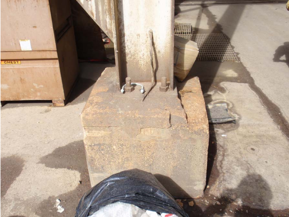
Unit 4 Typical of column bases at column lines L, M, N, and P
