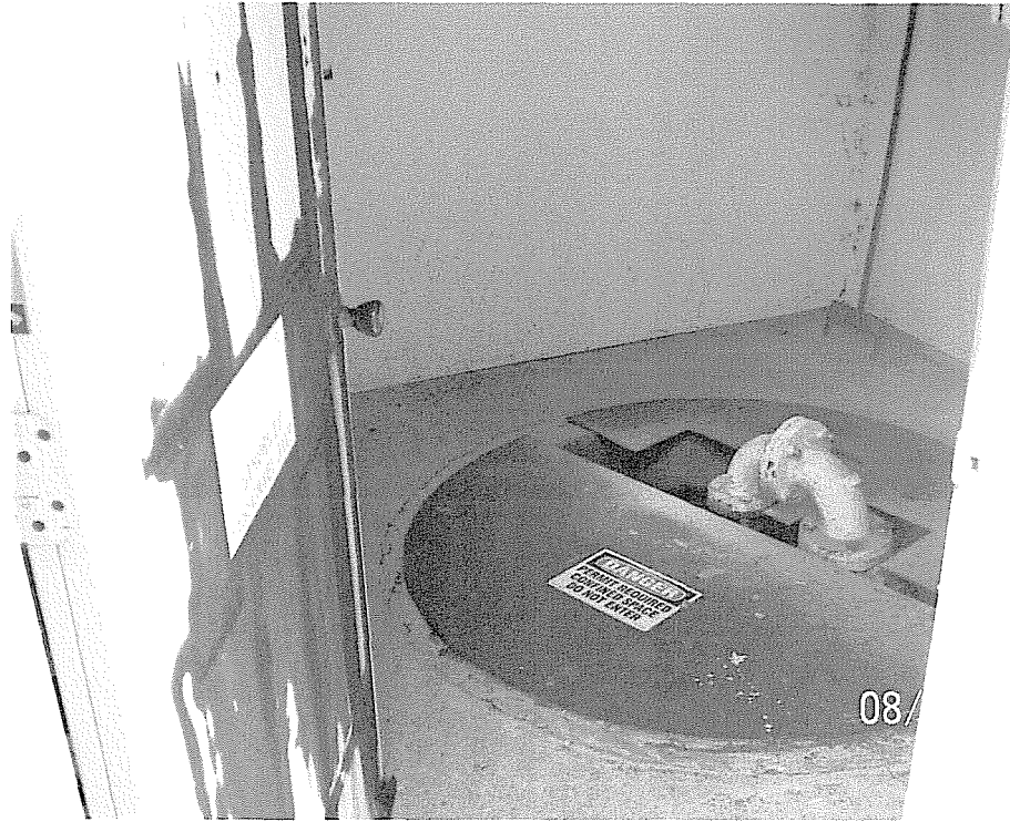
Blow off pumps for clarifier tanks located in small shed, away from other buildings. Extensive rust occurring on residential metal door. Pump and wet-well subject to freezing and corrosion.
