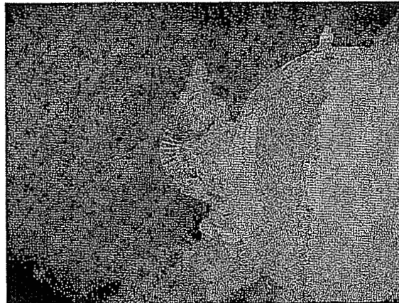
Figure 7 - 24-inch horizontal gate valve and operator
