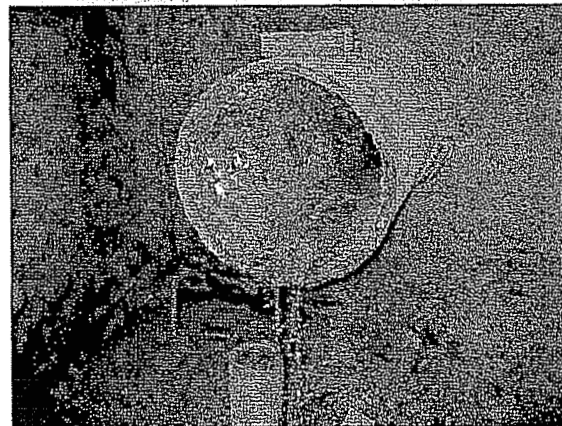
Figure 9 – Abandoned 24-inch line penetrating tunnel wall
