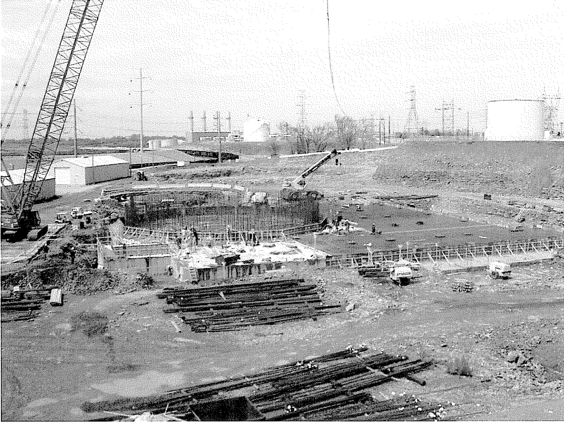
The picture above (dated 4/11/2007) shows a closer view of the main FGD foundation and absorber foundation from a different angle. The edge of the excavated area indicates the amount of soil that was removed and the amount of rock that was blasted and excavated to prepare the site for the FGD construction.
