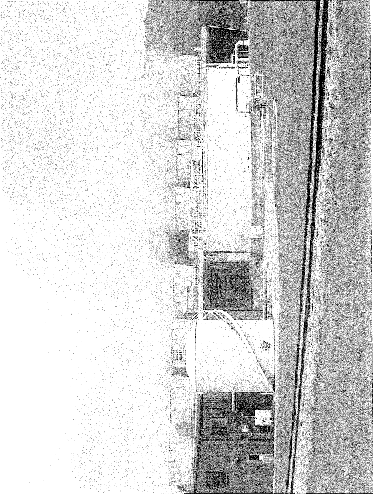
PHOTO 8: Cooling Towers for Units 1 and 2.
