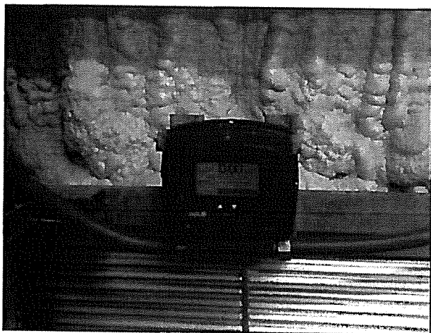
Influent flow meter showing no flow.
