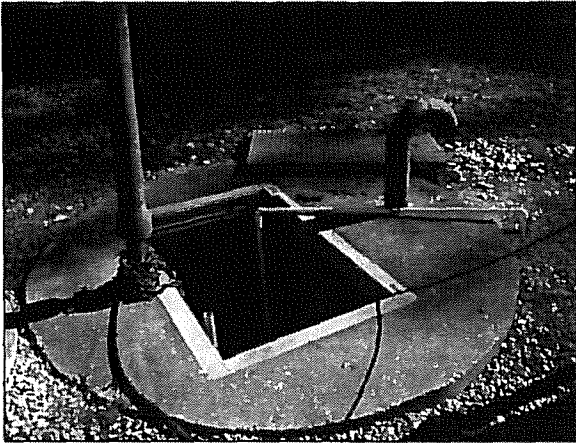
Lift station with detached lid
