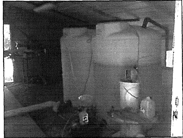
Liquid chlorine and de-chlorination.
