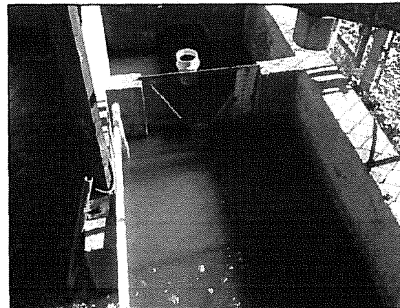
The effluent flow meter in the chlorine contact basin (color of water should be clear)
