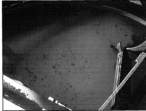
Clarifier (should be clear)
