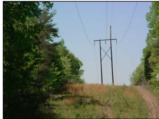
PHOTO 21: Typical 69kV Transmission Line in Rural KY
