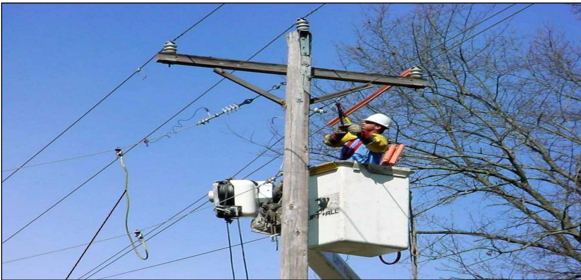
PHOTO 37: Three-Phase Distribution Pole and Hardware (insulators, cross-arm & braces, insulators & brackets, conductors, bolts, etc.)
