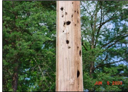
PHOTO 33: Wood Pecker Holes Limit the Strength and Shorten the Life of Wood Poles
