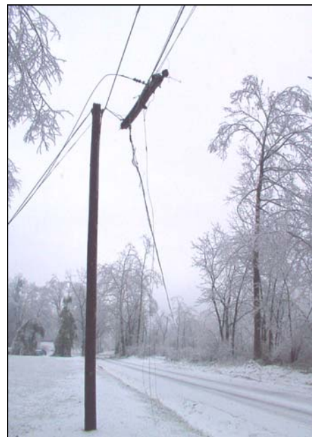
PHOTO 20: Pole Broken at Point of Joint Attachment by possible improper loading
