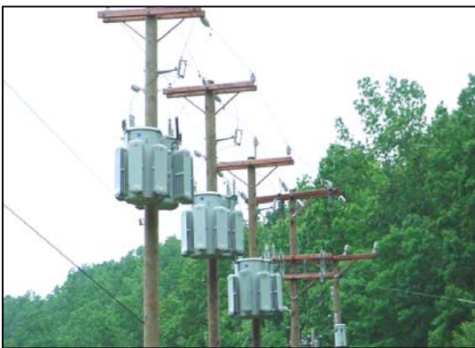
PHOTO 35: 34.5 x 12.4 kV Transformers
