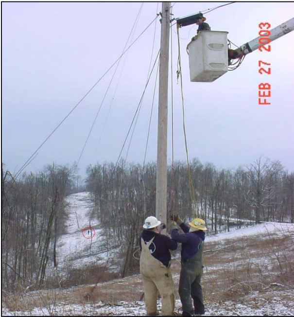
PHOTO 13: Lewis County, KY ~ Pike Contractor and Grayson Crew... Note Lineman in Distant R/W
