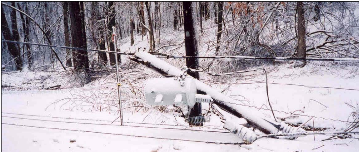
PHOTO 18 – Fleming County ~ Damaged Material Left While Repair Work Continued Elsewhere
