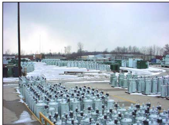
PHOTO 10: KU / LGE Transformer Storage Facility
