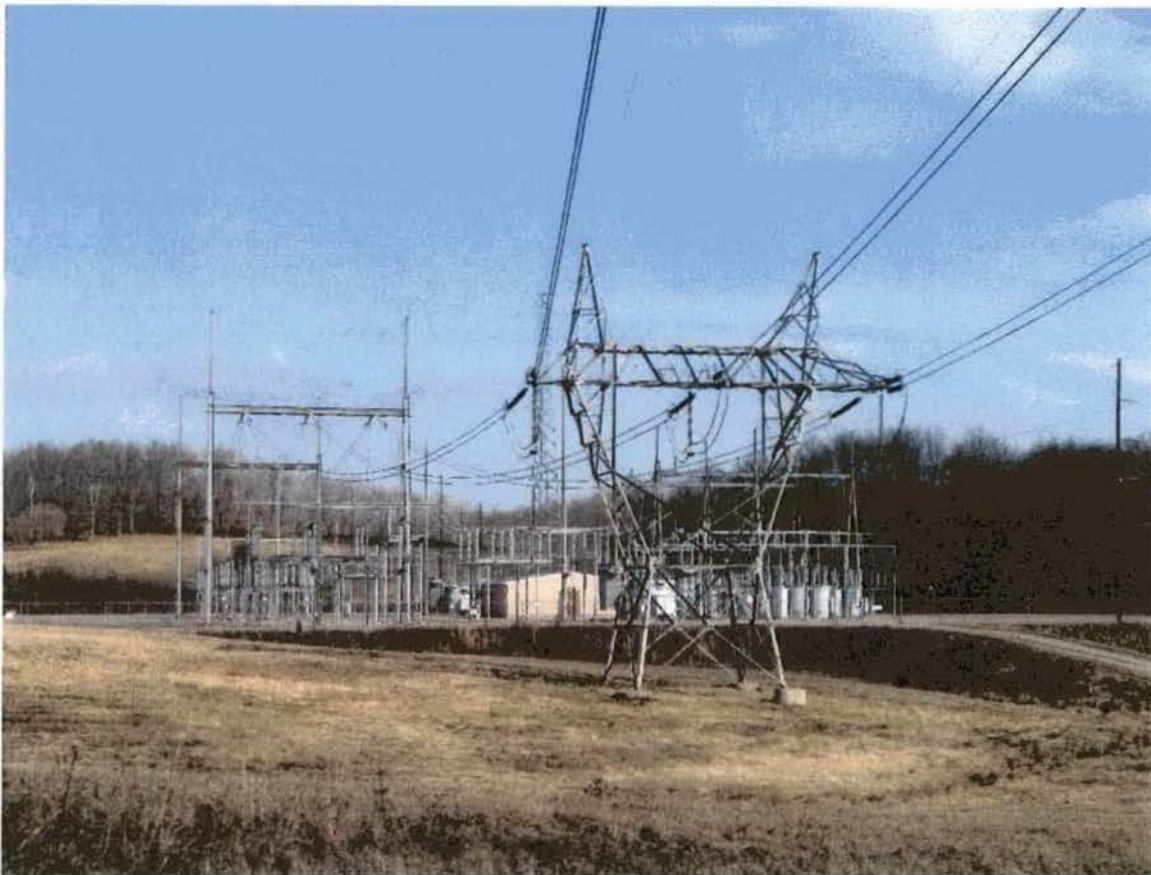
PHOTO: Coleman EHV Substation, Henderson, KY
