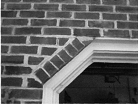
all brick and mortar separations should be repaired
