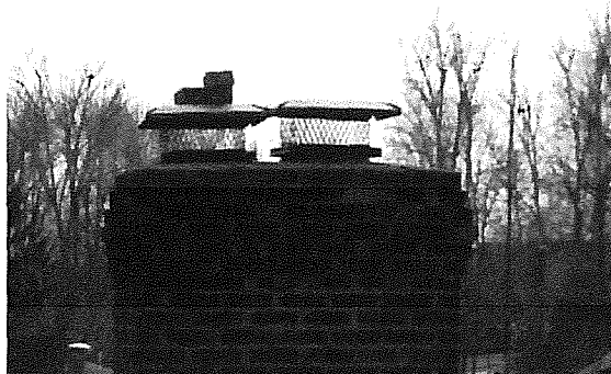
bricks could be a safety concern
