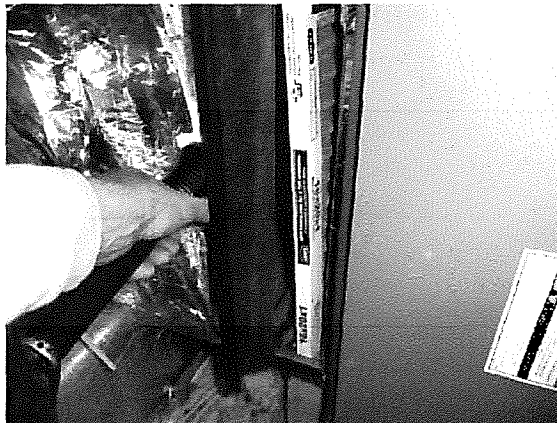
second filter location in the attic space
