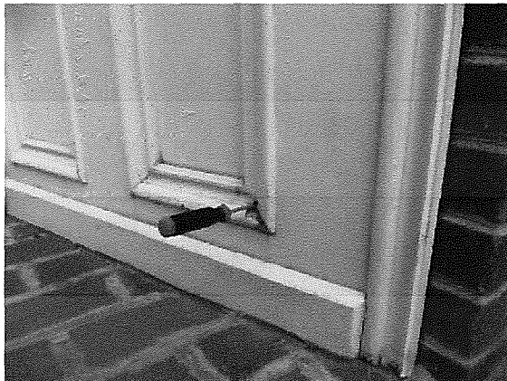
wooden trim was damaged at the front entry
