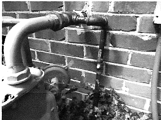
gas shut off valve for the basement fireplace gas log
