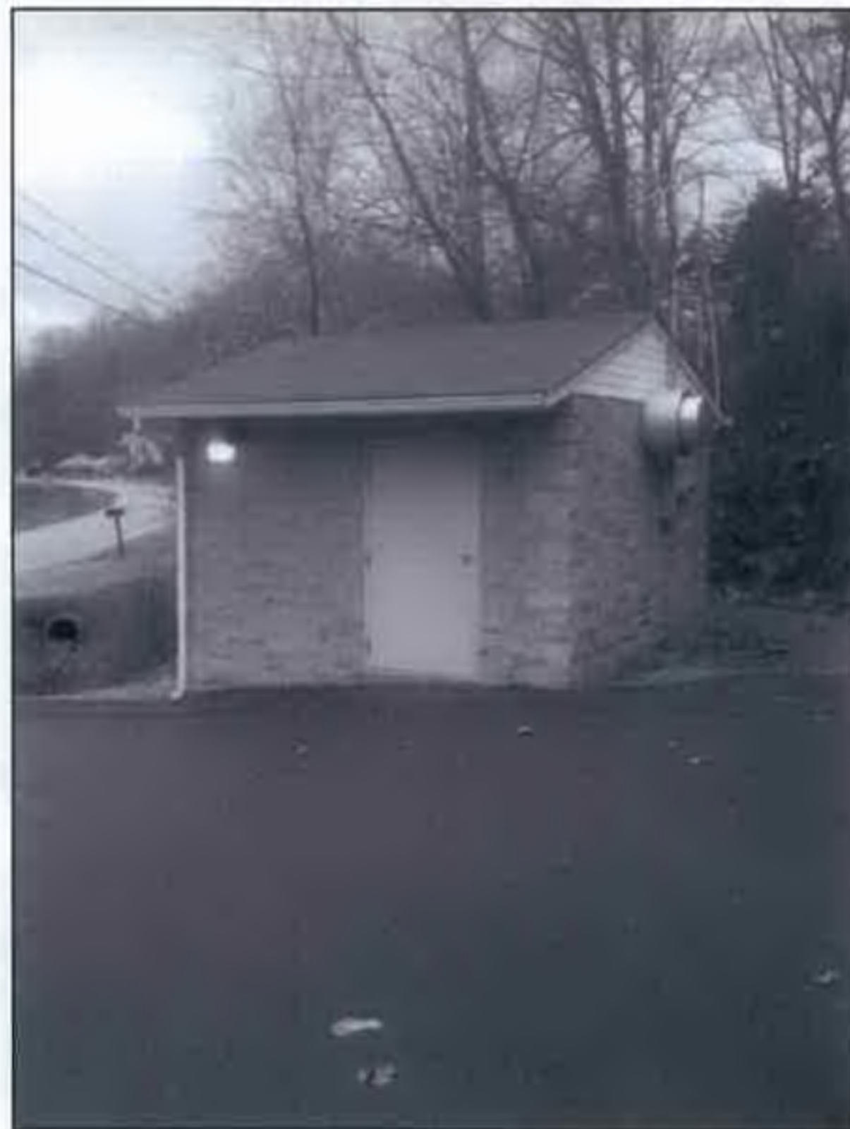
KY 7 PUMP STATION
