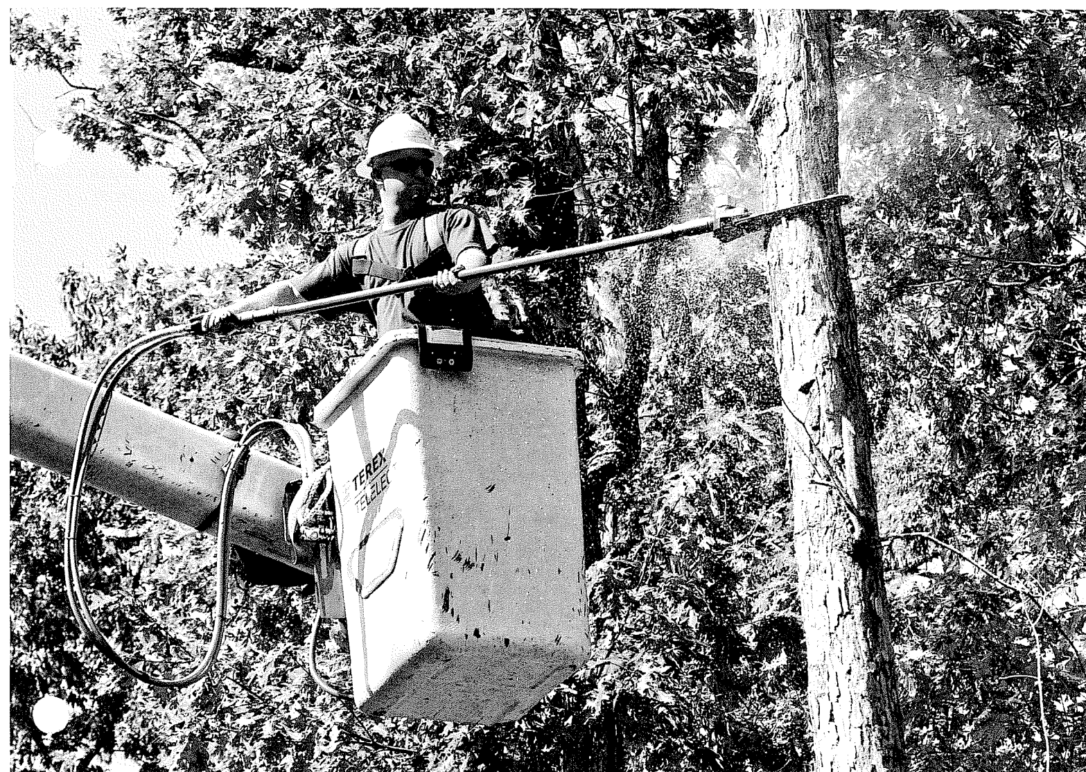
Keeping your electricity flowing means year-round trimming of vegetation that could damage power lines. Here, a contractor working for Fleming-Mason Energy Co-op uses a pole saw to remove threatening branches.
